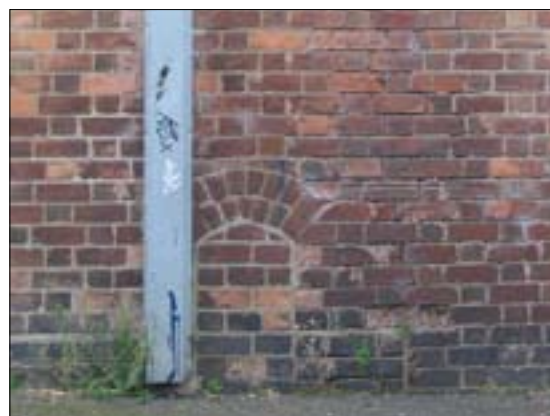
Figure 35 A blocked opening in the northern wall of block G. Hannah Waugh.
