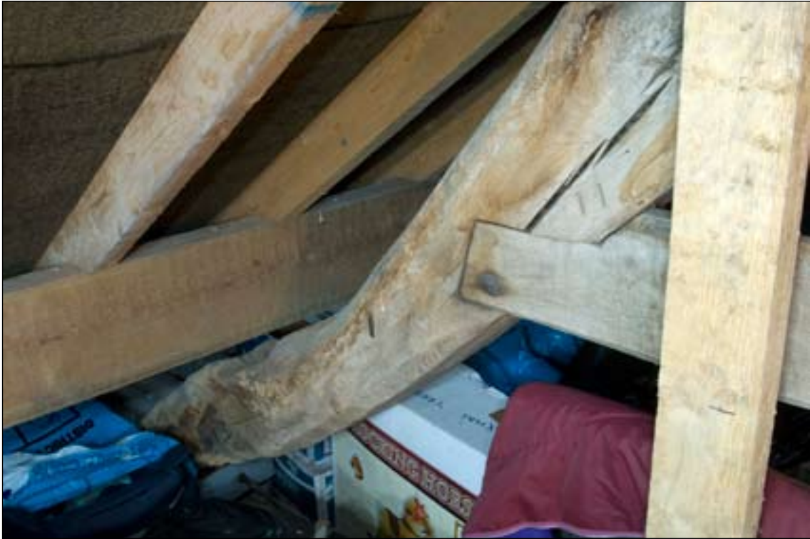
Fig. 14: The lower part of the northern principal rafter of the truss, showing the start of the curve of its foot. The marking on the principal denotes it as truss II. [DP072103]
