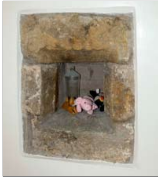
Fig. 10: detail of the chamfered window on the first floor of the north wall of the bastle, blocked when the northern addition was built. [DP072099]
