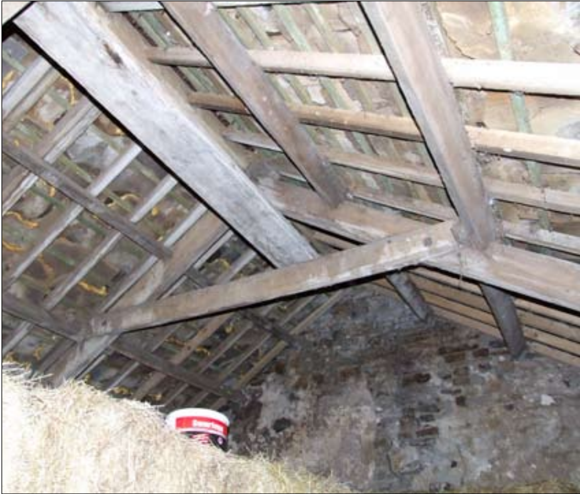
Fig. 26: View into the roofspace of the mineshop, showing one of the softwood trusses and traces of plaster on the east gable. [DPI35352]
