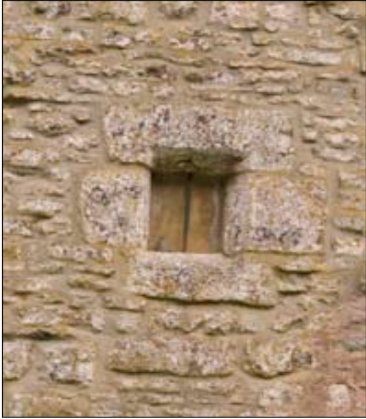
Fig. 9 : detail of the fire window on the first floor of the south elevation. [DP072082]
