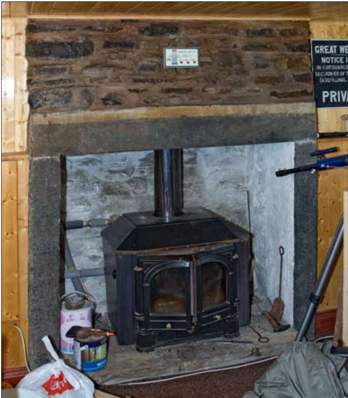
Fig. 20: The monolithic-jambed fireplace in the self-contained first-floor dwelling, situated at the western end of the early 19th-century northern addition. [DP072100]
