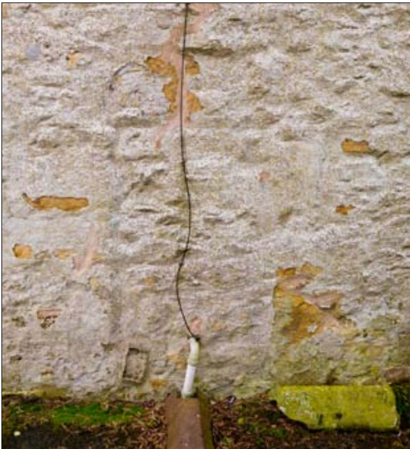
Fig. 11: the blocked byre doorway in the east gable wall of the bastle. [DP072097]
