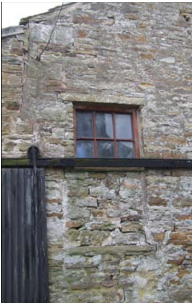
Fig. 24: The blocked first-floor doorway, now a window, in the west gable wall of the mineshop, [DPI35349]
