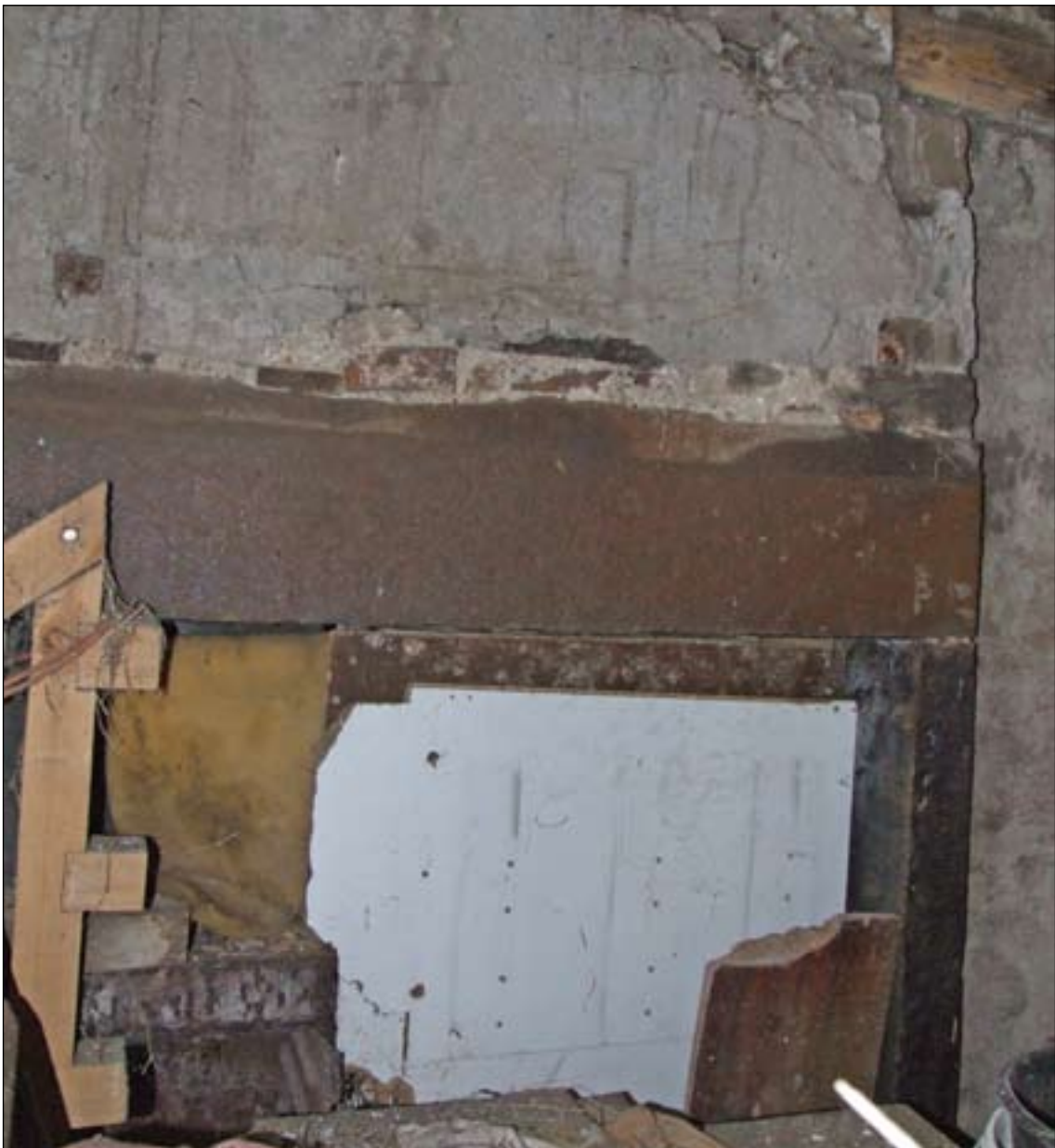
Fig. 25: The first-floor fireplace, with monolithic jambs and lintel, at the west end of the mineshop. [DPI35351]
