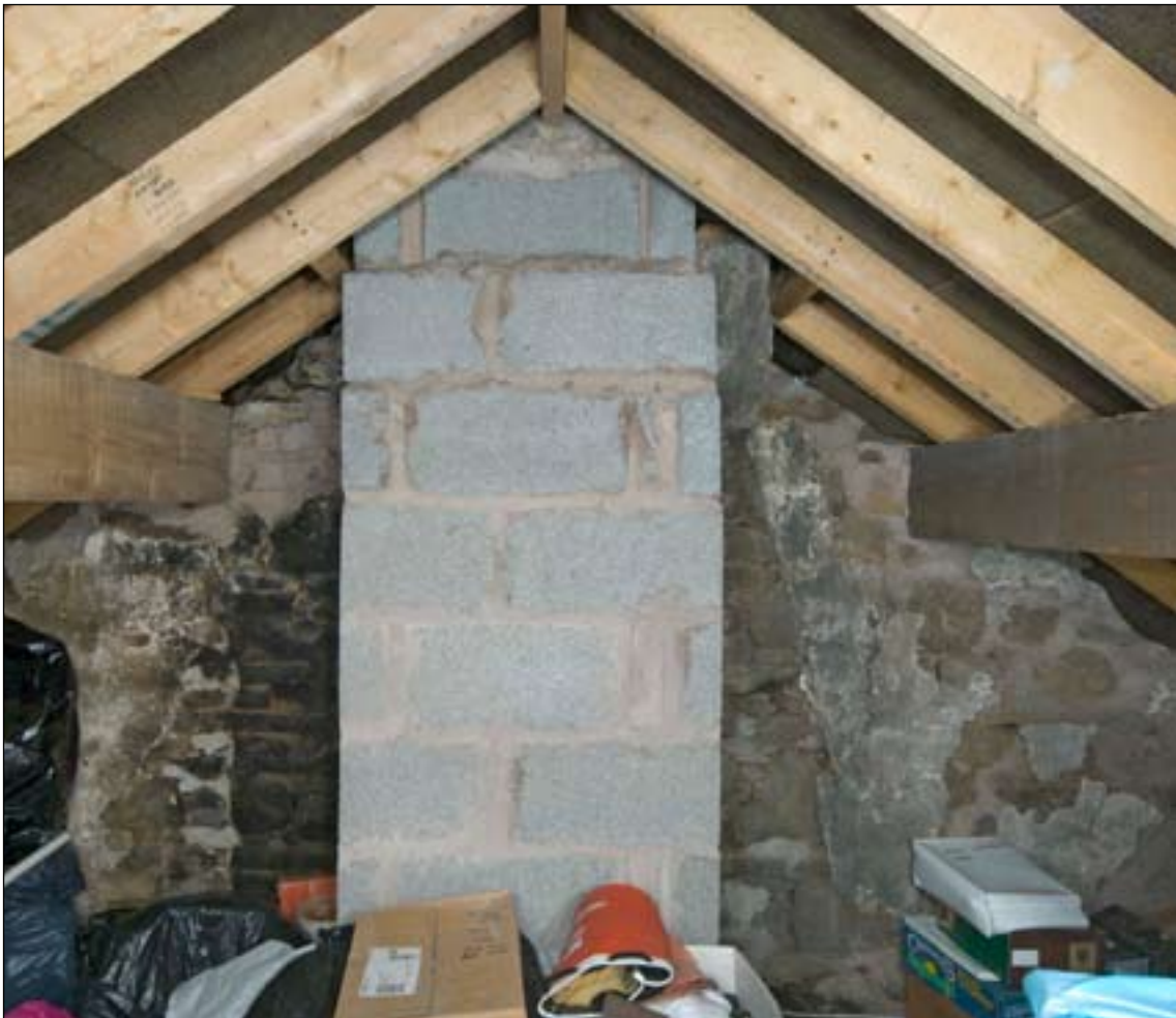
Fig. 12: view within the roof towards the west. The diagonal plaster scar to either side of the modern stack shows the form and position of the removed smoke hood. [DP072104]
