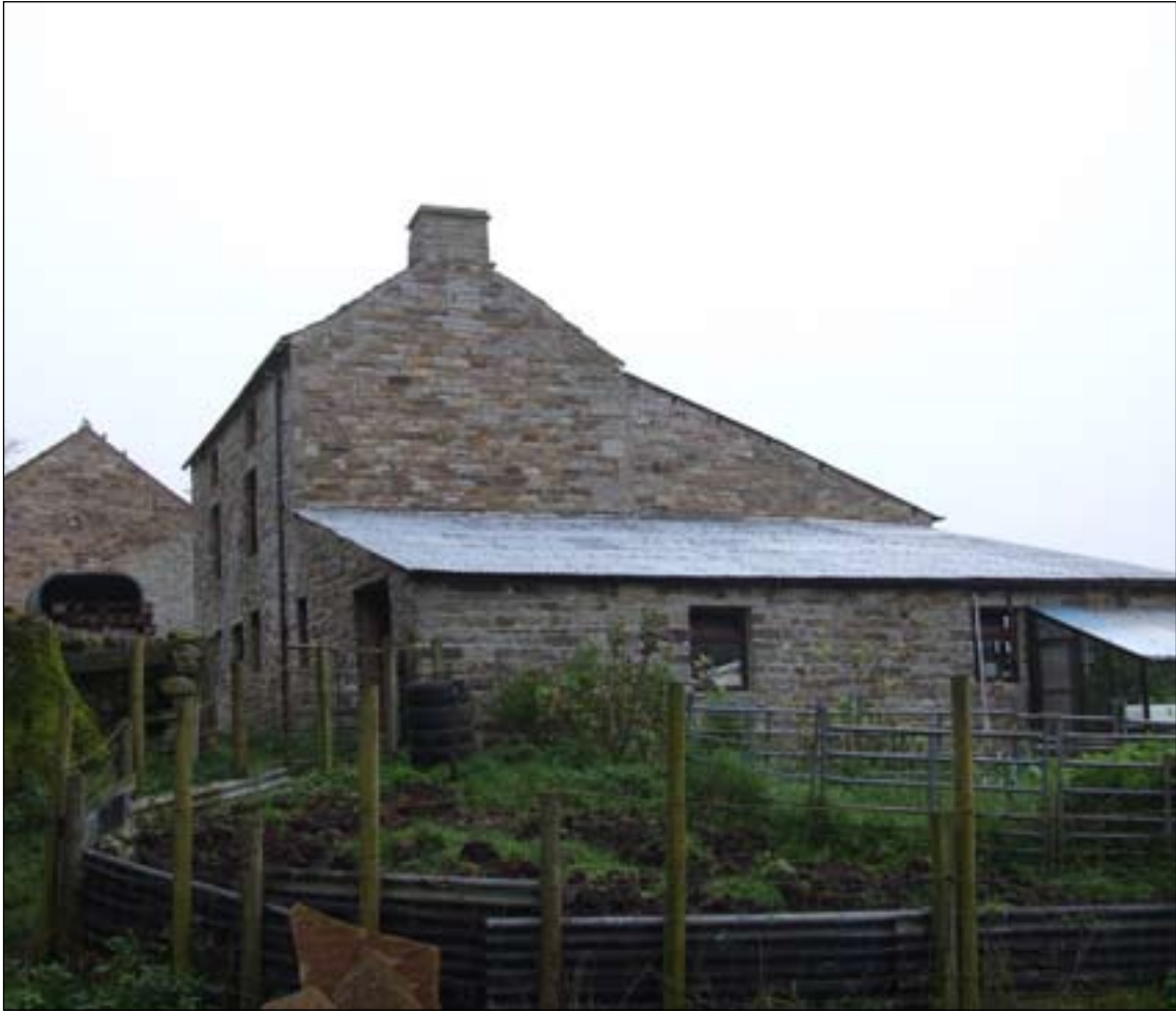
Fig. 27: View of the mineshop from the south east, showing the redundant eastern stack and the stable added to the east wall. [DPI35353]
