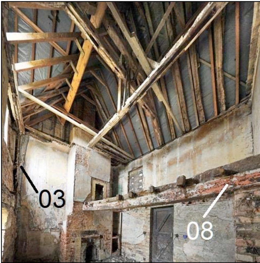
Figure 3. Photograph of the interior without scaffold in place, showing two of the timbers sampled for dendrochronology (adapted from an original supplied by Caroe Architecture)
