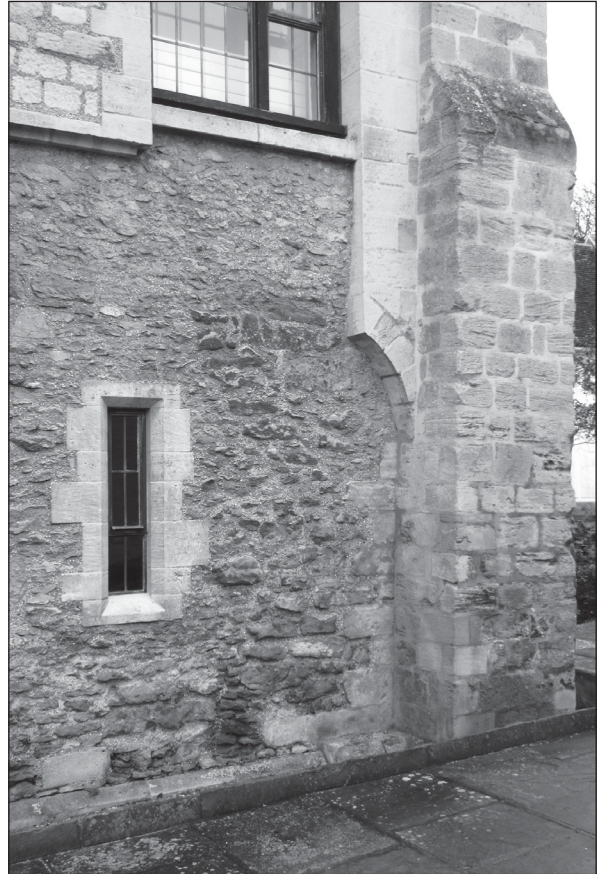
Figure 30. The arch rising out of the north-east buttress, to support the north jamb of the original first-floor doorway.
