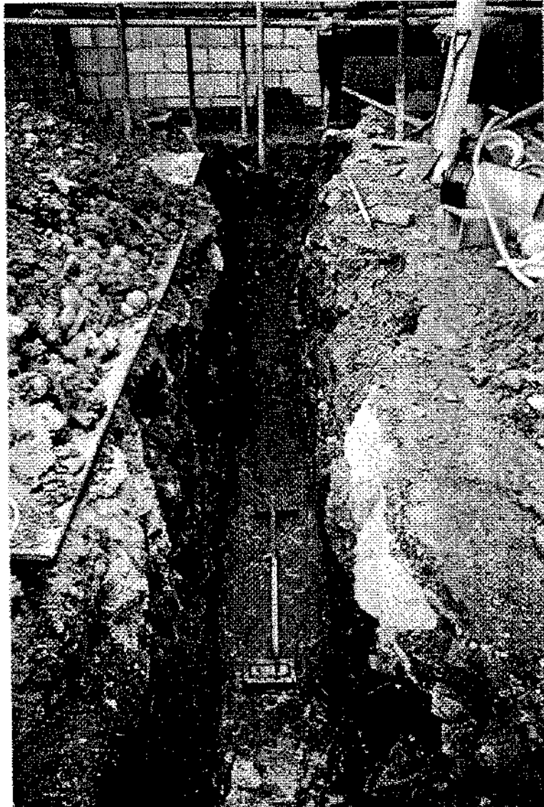
Plate 1: Trench 3. Machine-brick walls in foreground, subsoil with overlying post-medieval deposits in background. Black plastic sealing base of Evaluation Trench B visible in Trench 3 sections.
