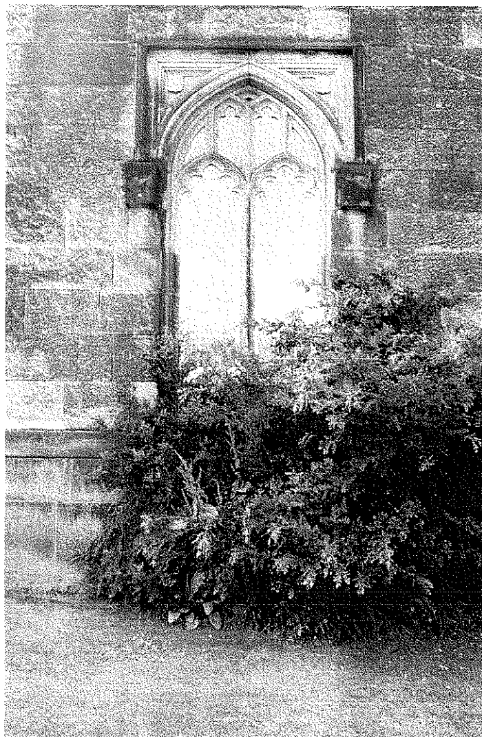
Plate 5 Priory Hall window detail
