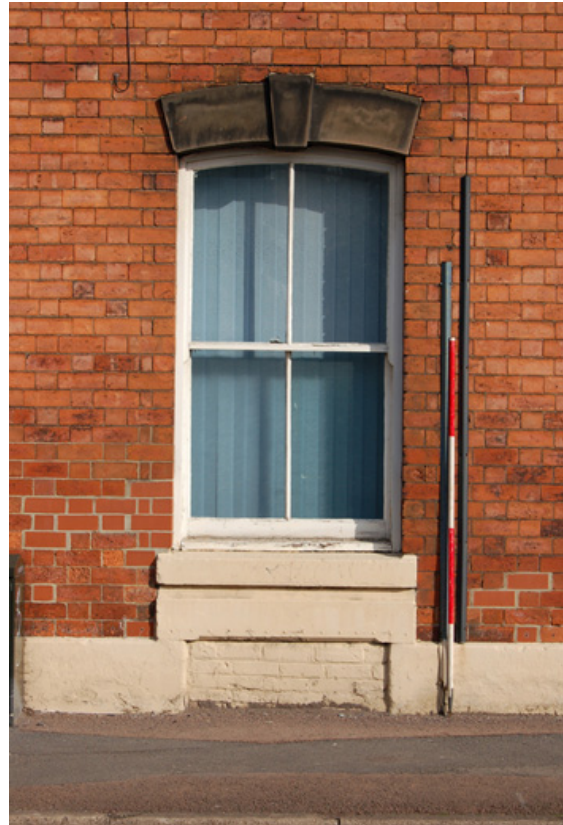
Plate 4: 2-8 St Helen's Street; detail of window, note blocked borrow-light below.
