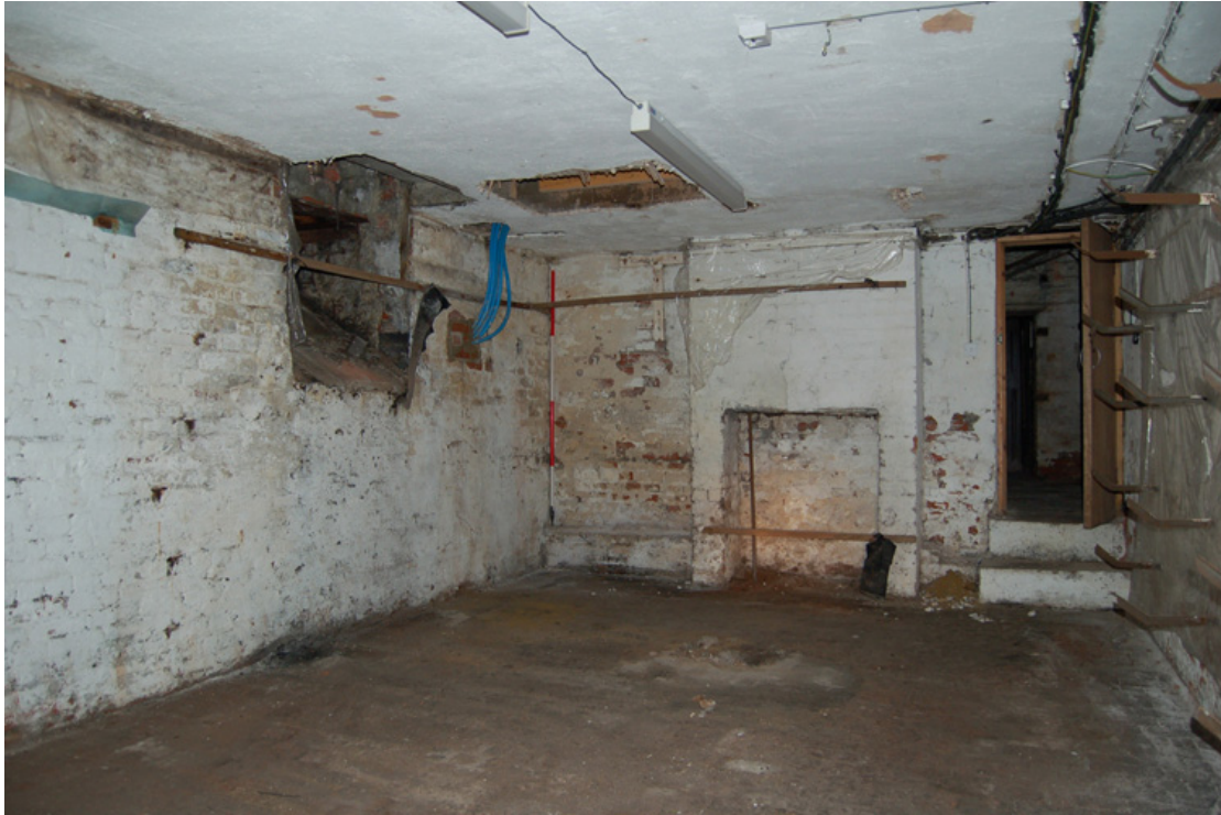
Plate 6: Basement Room B1, looking west. Note coal chute to south wall (left).
