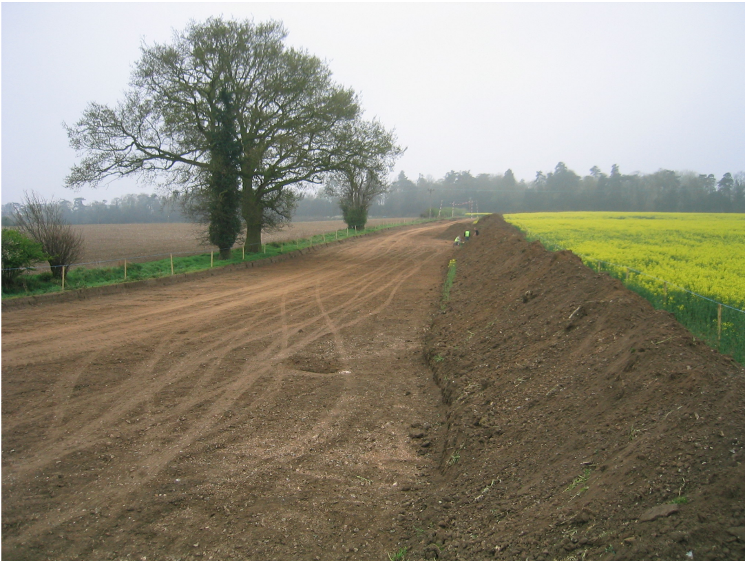
Figure 2: A section of the proposed pipeline route cleared by Anglian Water for archaeological and palaeoenvironmental assessment. Looking southwest towards A134 Sicklesmere Road.
