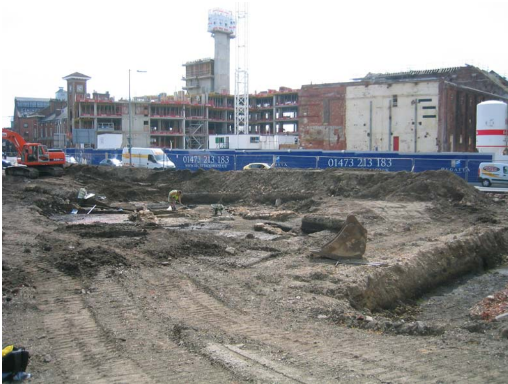
Figure 1: Ipswich triangle West, Ipswich. Looking southeast across the site, with Albions Wharf located to the south.
