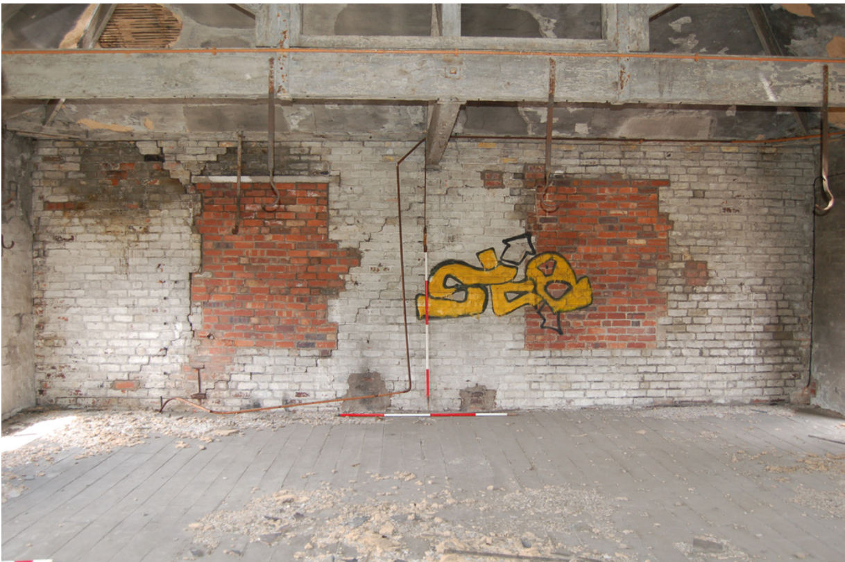
Plate 41: Building D; Level 3, blocked windows in west wall.
