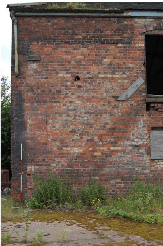
Plate 46: Bldg E, scar of former stair (Bay 1).
