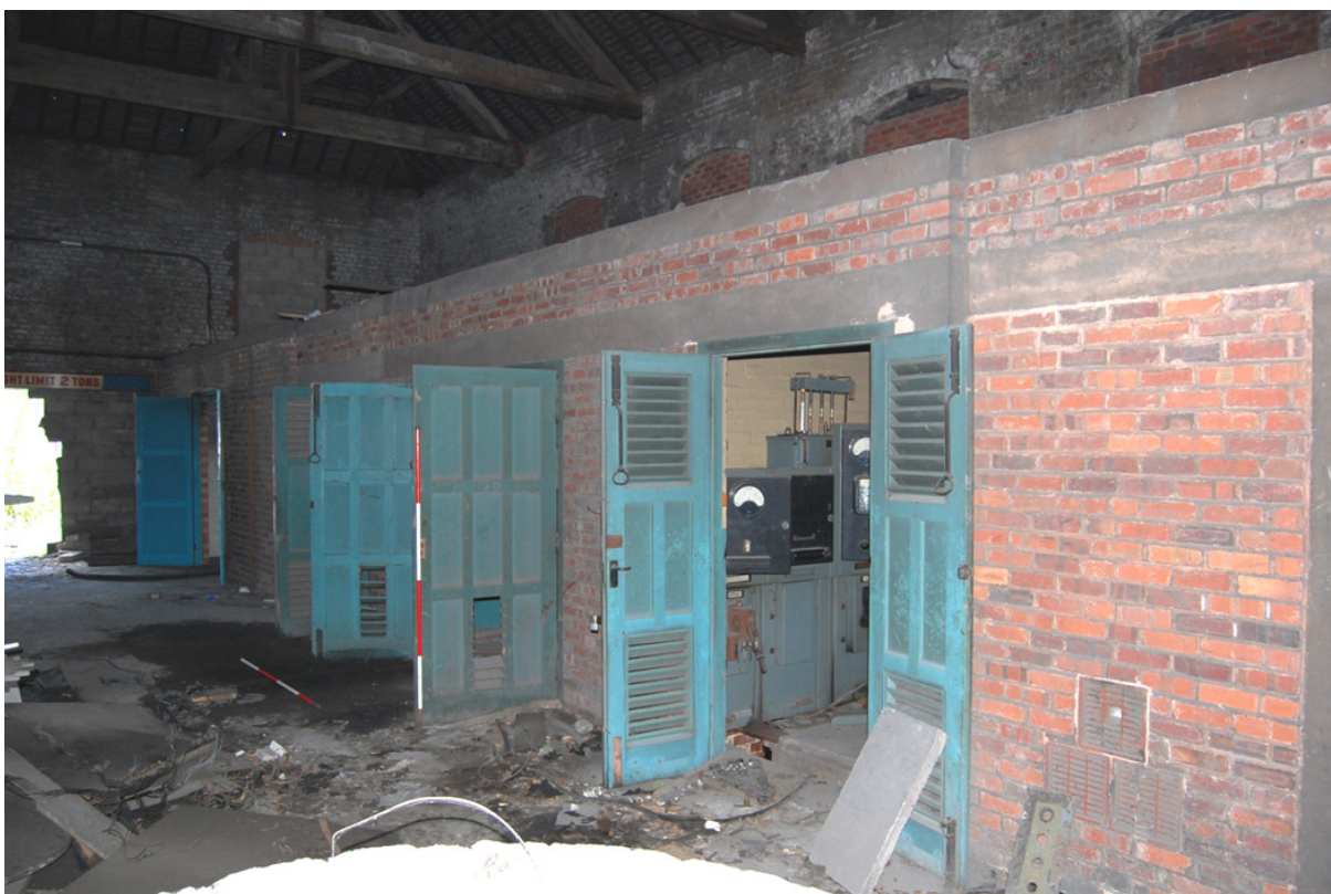
Plate 19: Building B, interior view looking east, note blocked windows visible above plant rooms.
