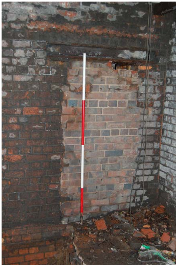
Plate 10: Building A, north wall, blocked door.
