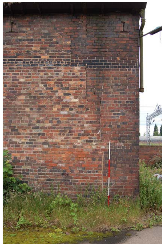
Plate 47: Stepped straight joint at Bay 12.
