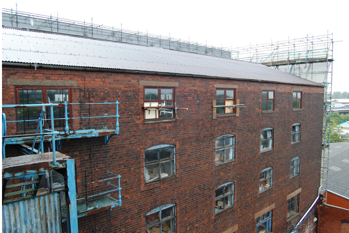
Plate 60: Building K, North Range; note rebuild of upper wall and alteration of windows.
