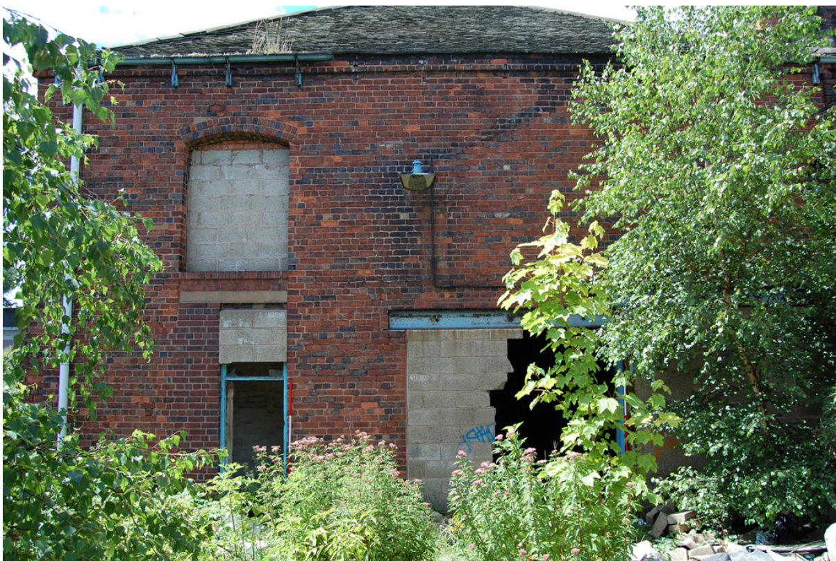
Plate 17: Building B, east elevation. Note shadow of former infill block (see Figure 17d).
