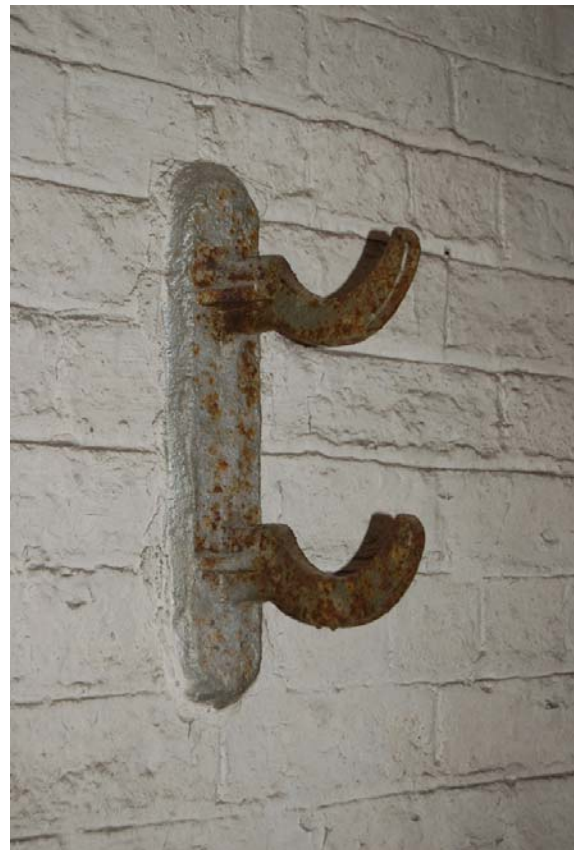
Plate 43: Bldg D; Level 3, wall mounted heating pipe brackets.
