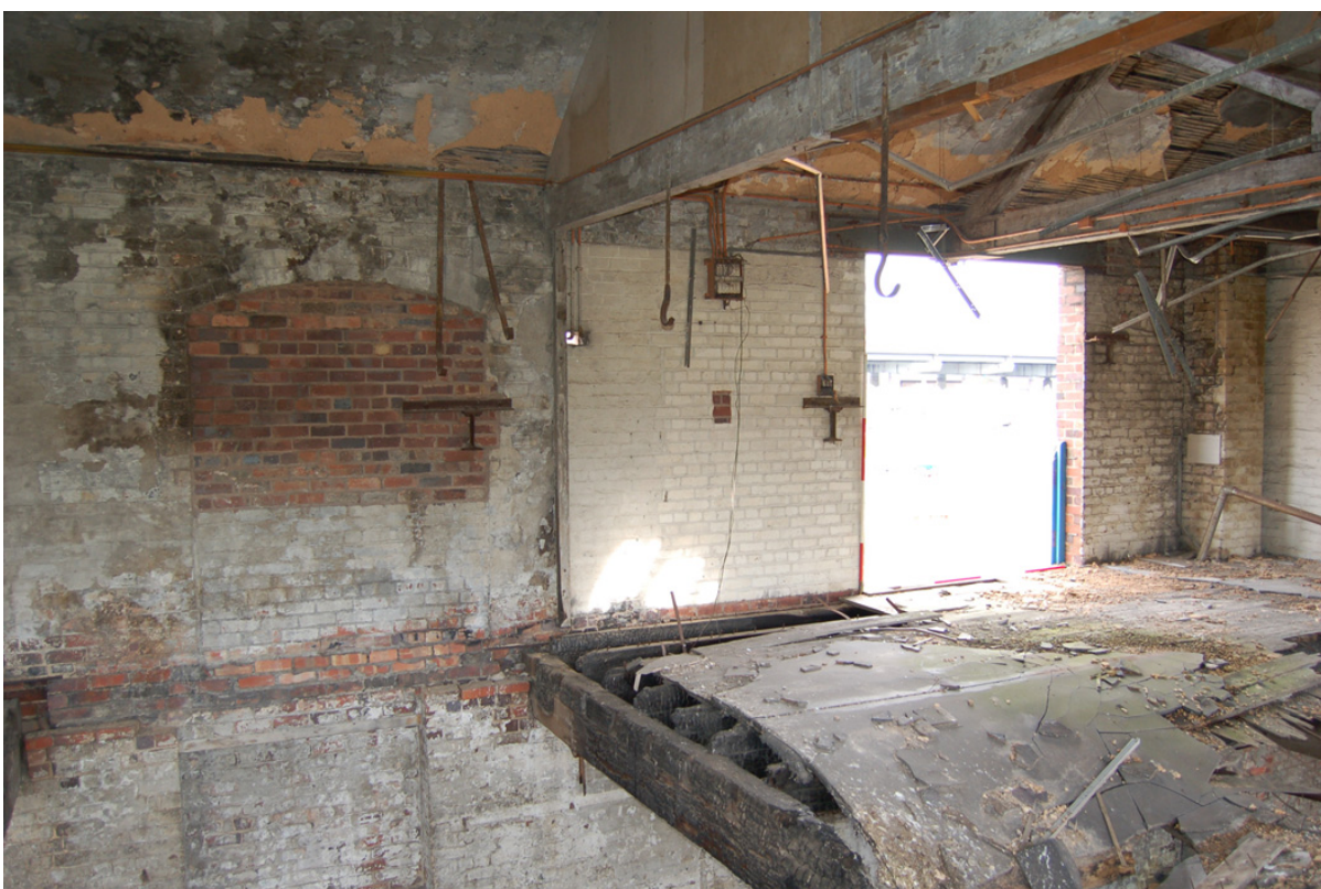
Plate 38: Building D, Level 3, blocked doors in Bays 8, 9 and 10 (north)
