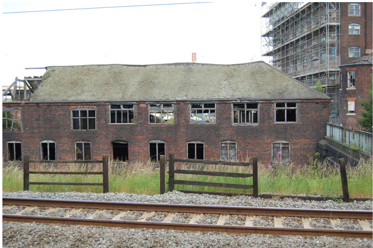
Plate 2: Building C, south elevation, east end from south side of NML canal.
