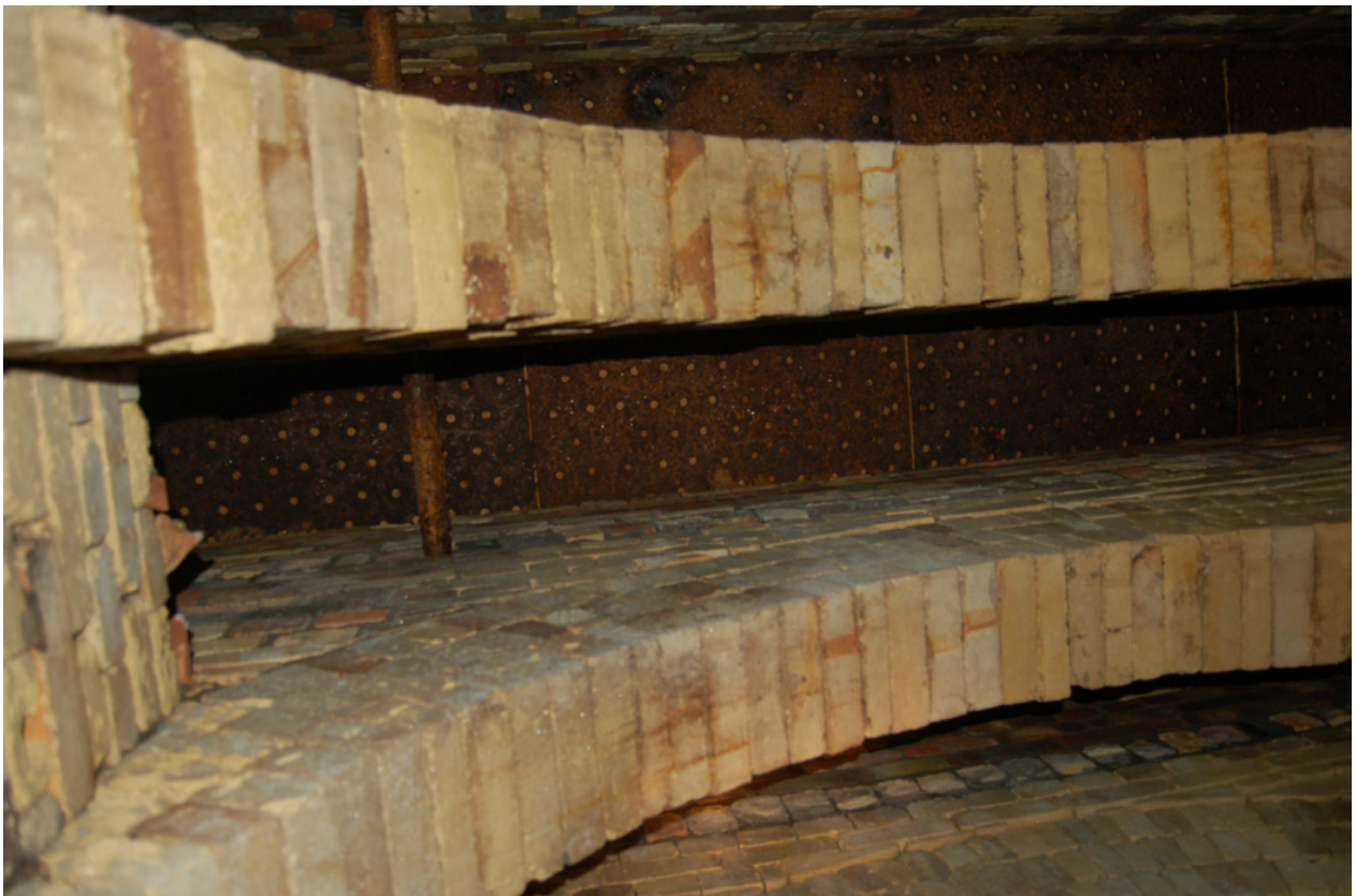
Plate 23: Tunnel C, detail of voids extending upwards to soffit of perforated iron plate. Note iron tie rod.
