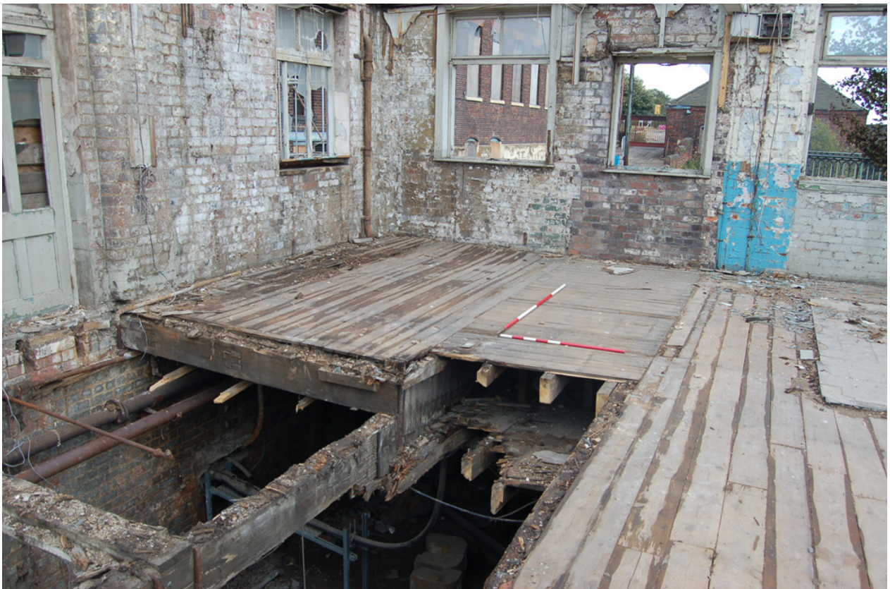
Plate 12: Building C, Level 2; evidence of former ramp (centre) exposed beneath office partitions.
