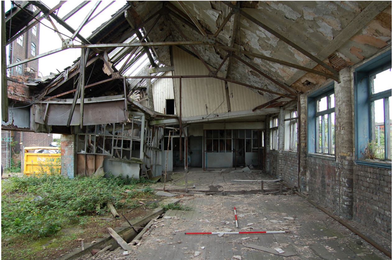
Plate 5: Building C, Level 2 interior looking east; office sub-divisions, note collapsed roof.
