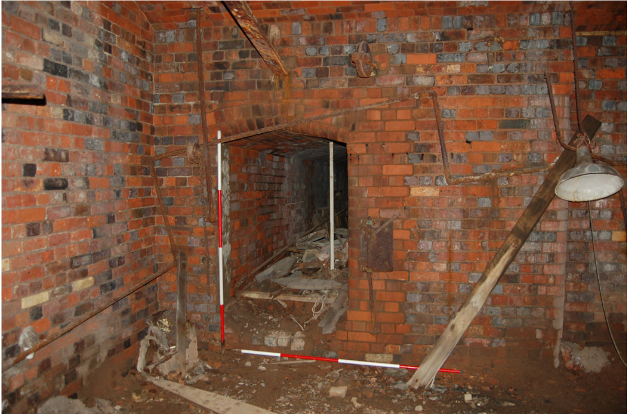
Plate 33: East end, south wall, (eastern passageway leading to Building C, Level 1; inserted).
