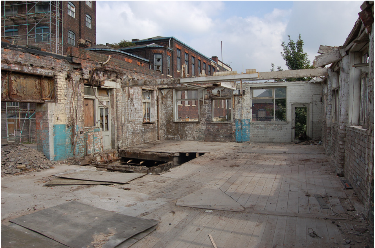
Plate 11: Building C, Level 2 looking east after removal of office partitions and unsafe roof structure.
