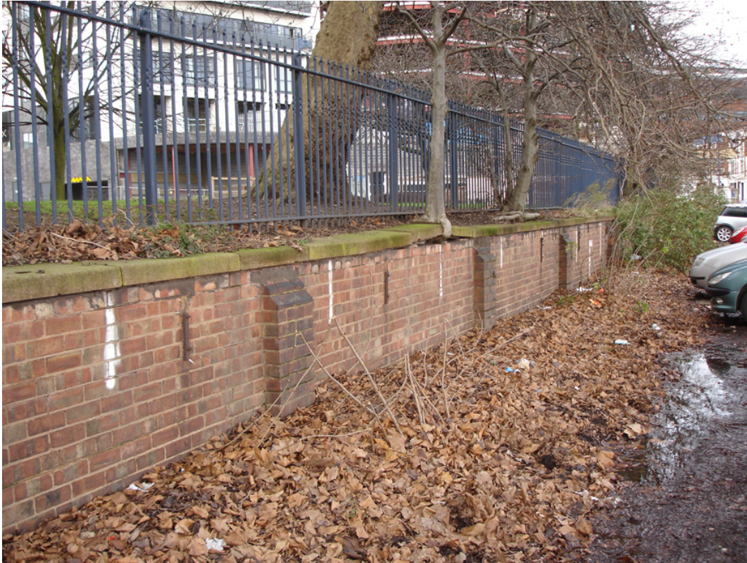
Plate 15: Retaining wall of Park Street Garden, which forms west boundary of study area, note change in ground level.
