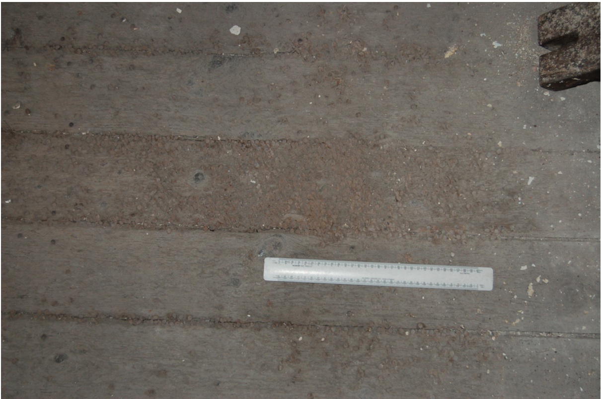
Plate 28: First floor; concentration of nails in floorboards at east end of range.
