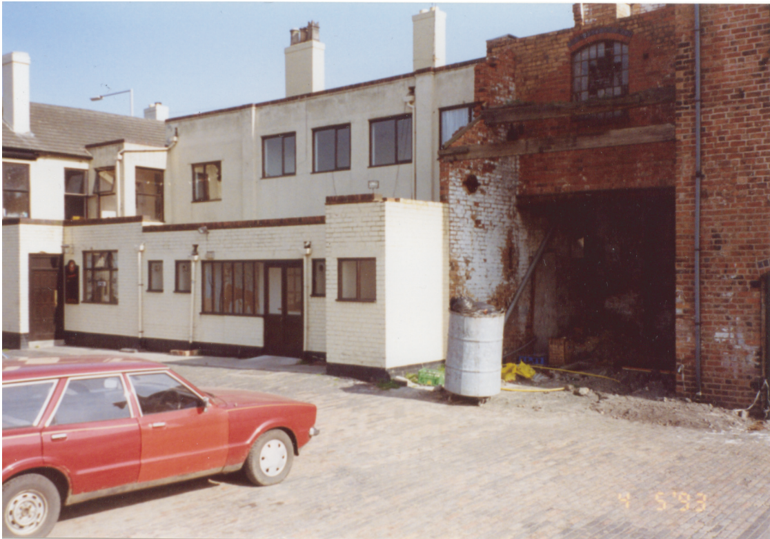
(a) Tower section of brewhouse range photographed prior to refurbishment/rebuilding, 09.05.1993. Note form of original windows matching those of surviving range (photo courtesy T. Batham).
