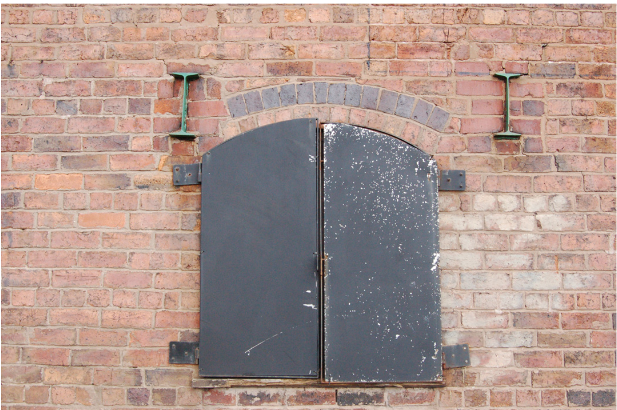
Plate 6: South elevation, fenestration detail; note patching around inserted joists.
