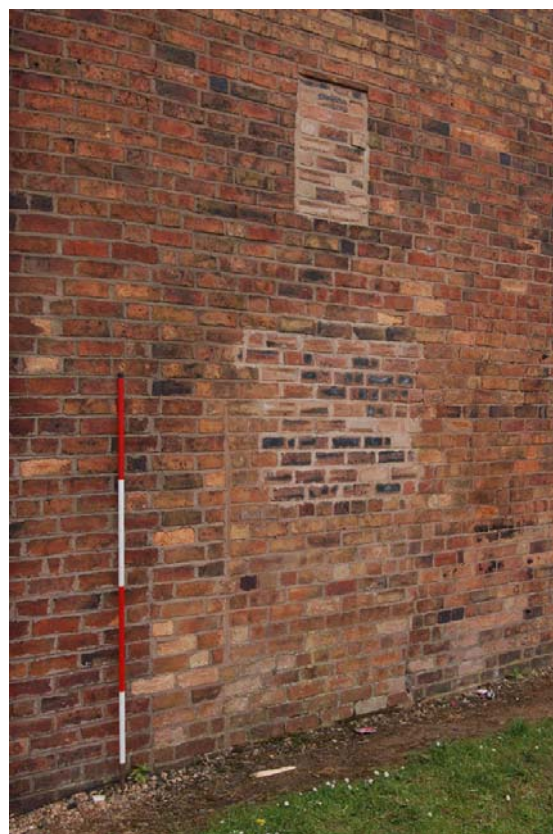
Plate 14: Stairwell/lift shaft; blocked door.
