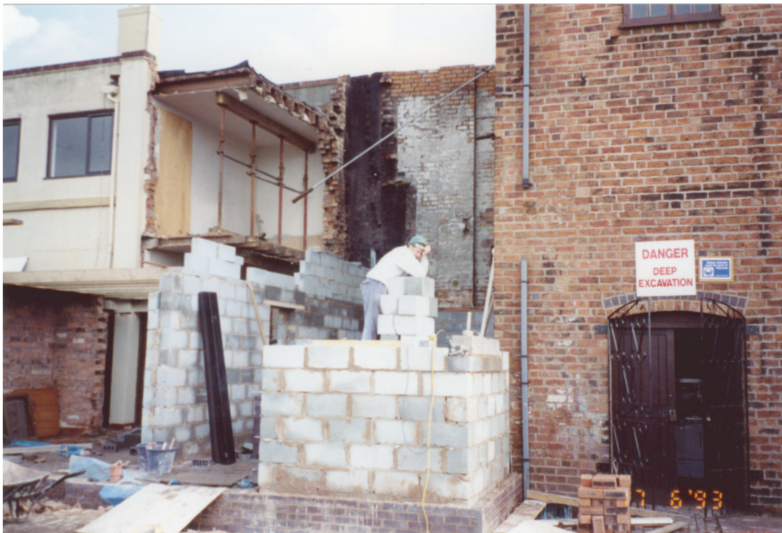
(b) Tower section of brewhouse range photographed during refurbishment/rebuilding, 17.06.1993. Note smoke blackened flue to rear wall (photo courtesy T. Batham).
