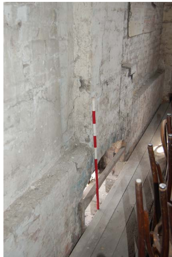
Plate 26: Window cut by lowered floor.
