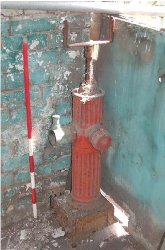
Plate 12: 2F, pump in SE corner.
