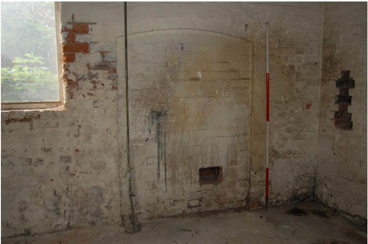
Plate 341: Building H, ground floor; blocked door at Bay 4 (south).
