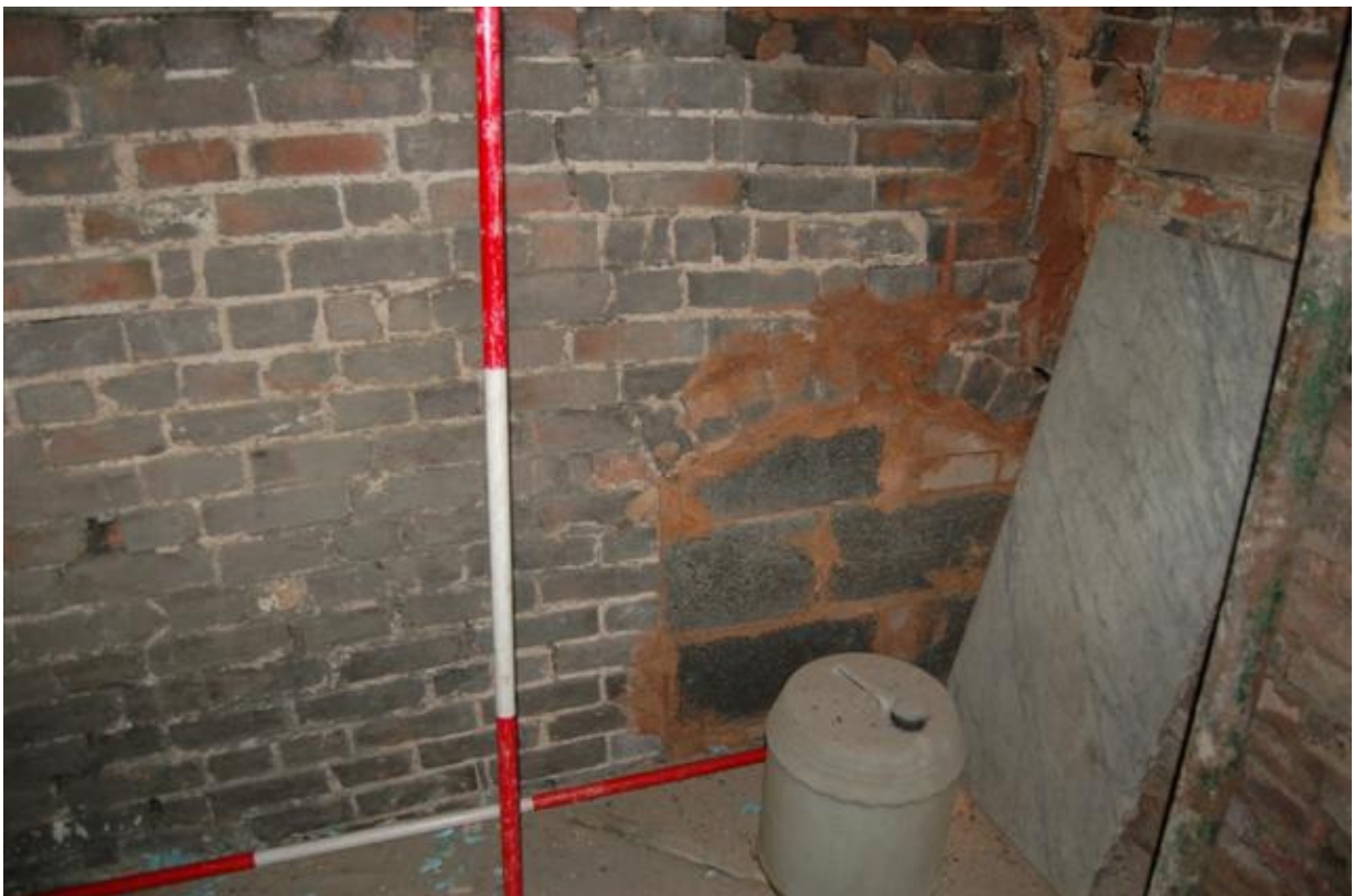
Plate 106: Building A, Block A7; Room AF15 blocked window.
