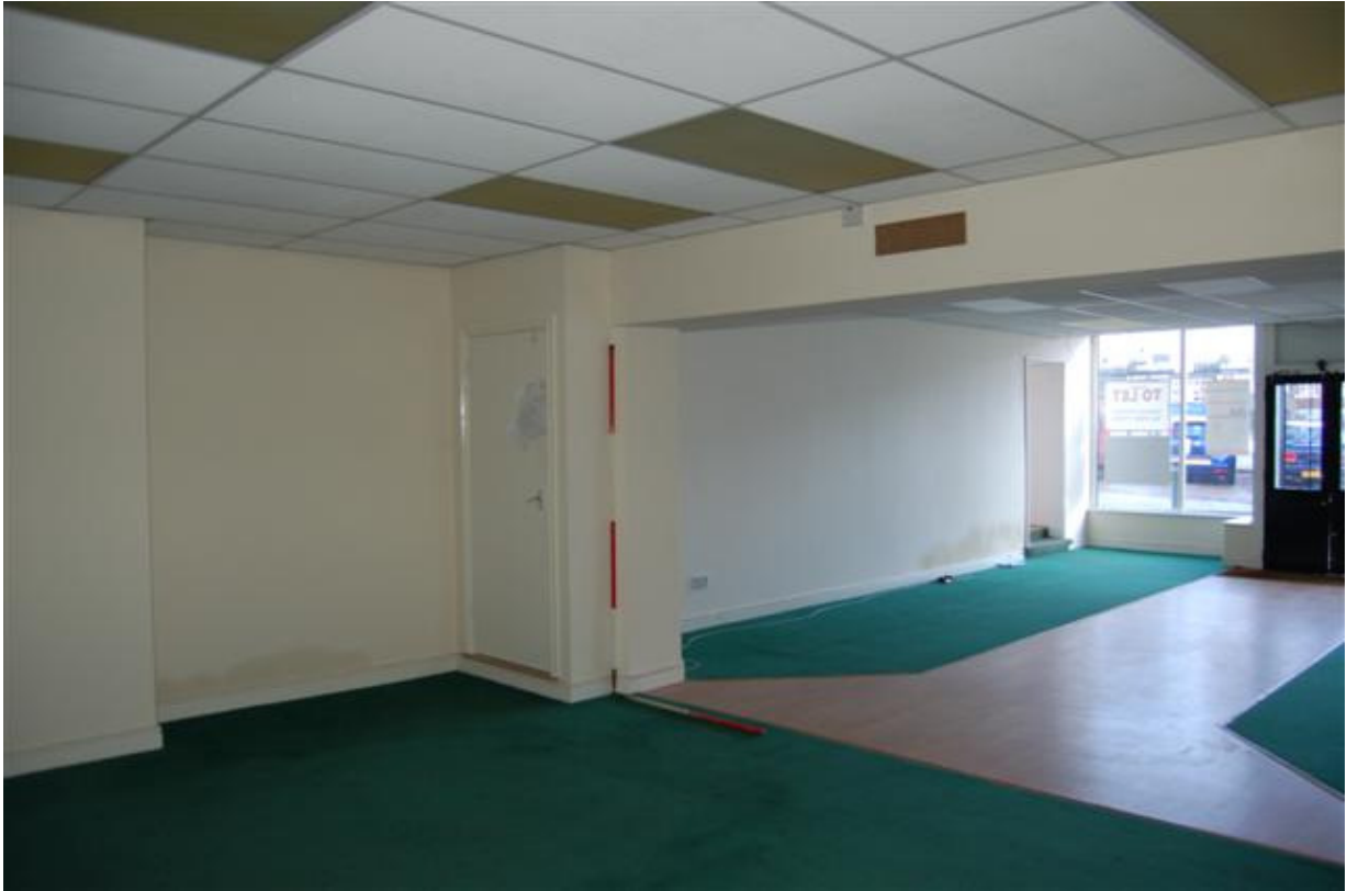
Plate 13: Building A, Block A2; Room AG2 looking north-east (Room AG1 to right).
