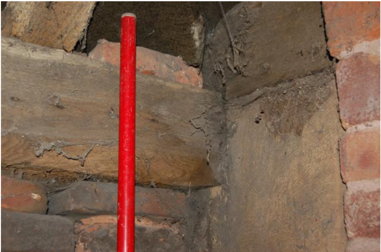
Plate 91: Building A, Block A6; Room AF14, detail of east wallplate (south end).
