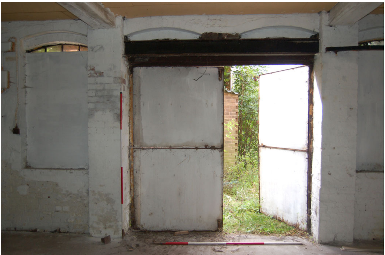
Plate 304: Building E, ground floor looking west; original windows (Bay 2) converted to door.
