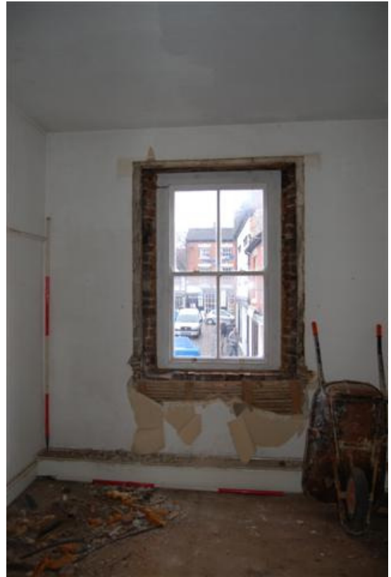
Plate 137: Bldg B, Block B1; Rm BF2 window.
