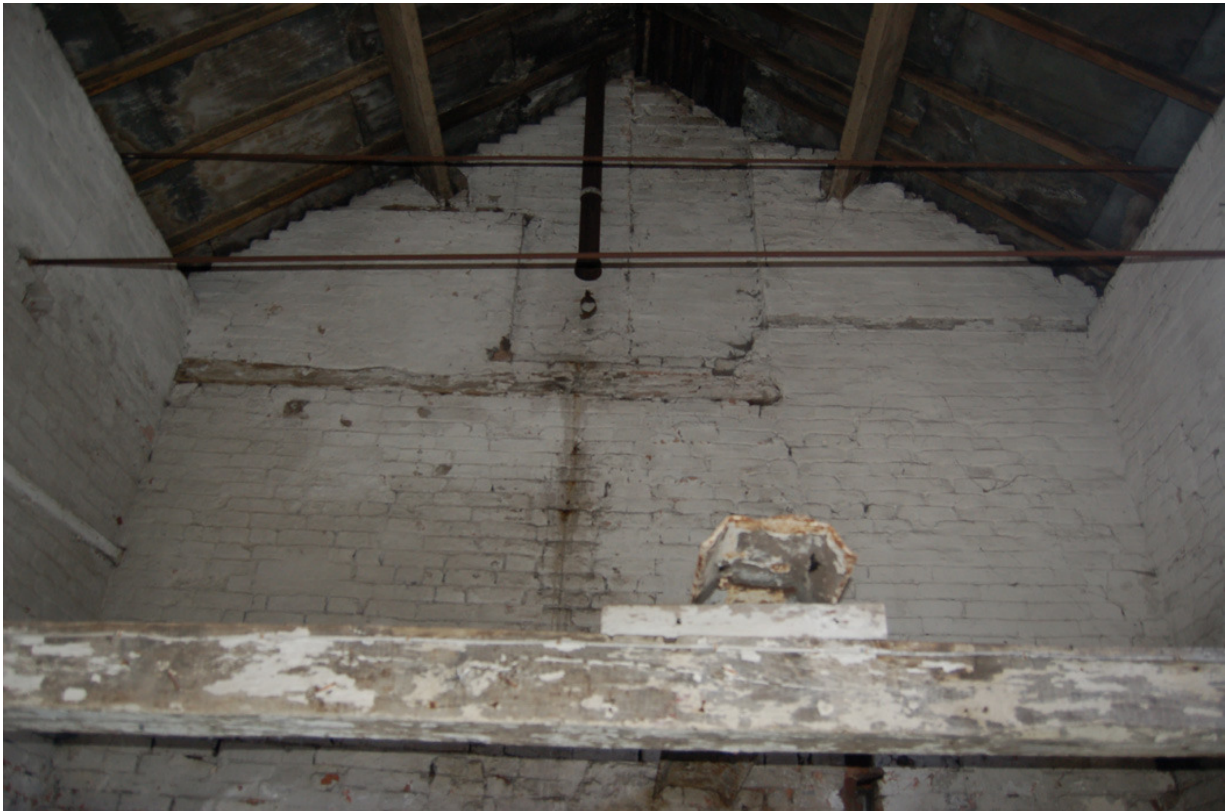
Plate 216: Building B, Block B7; Room BG25, east wall; blocked opening at high level.
