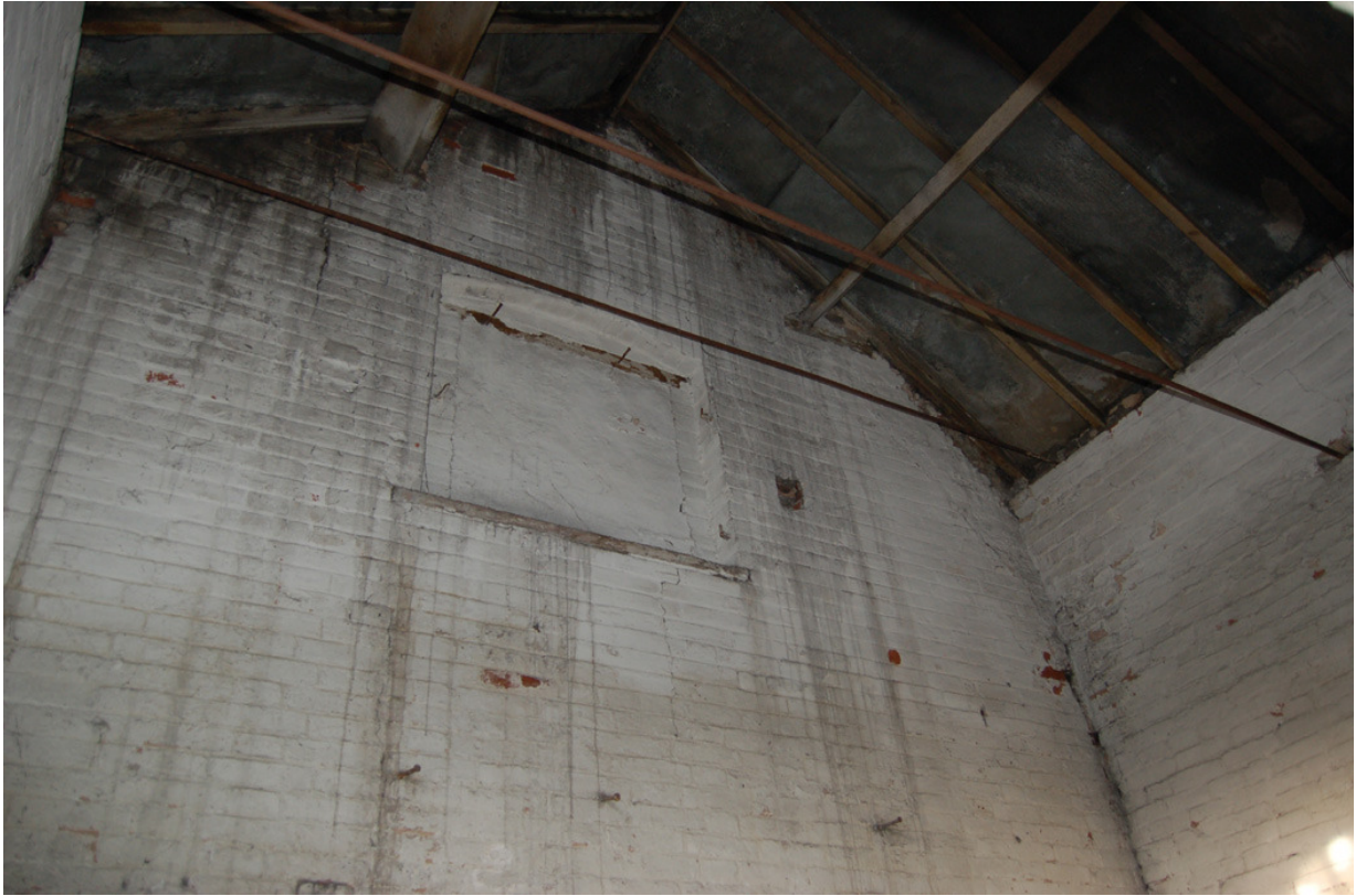
Plate 217: Building B, Block B7; Room BG25, west wall; note raised brickwork of north wall and former roof scar.
