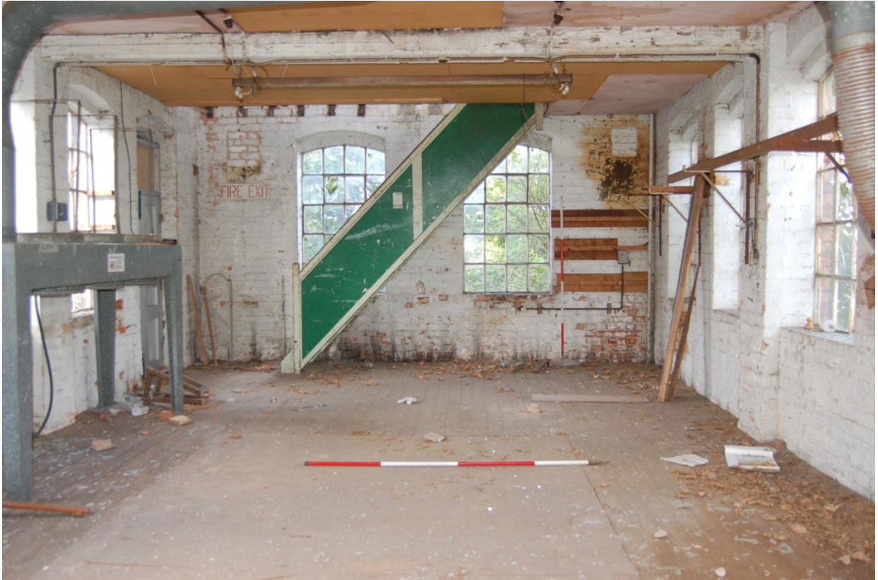
Plate 305: Building E, 1 st floor looking north; note patches to suggesting location of former line-shafts.
