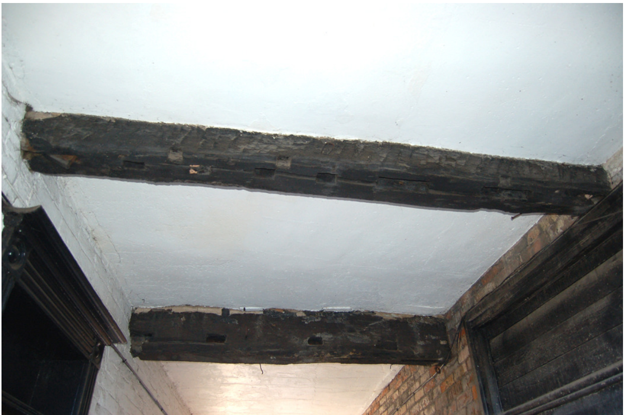
Plate 23: Building A; Block A3; Passage to north of No. 16 Church Street, detail of timber ceiling beams.
