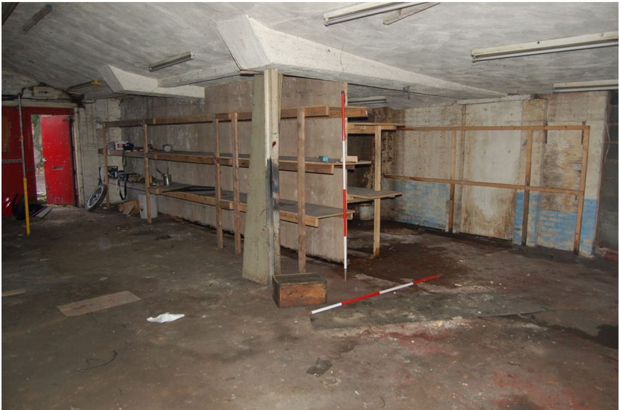
Plate 352: Building I, interior looking north-east: note ribs of original 'Nissen Hut', truncated and encased.
