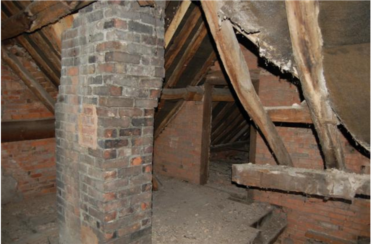
Plate 251: Building C, Block C1; Room CS2 roof structure and stack looking south-west.
