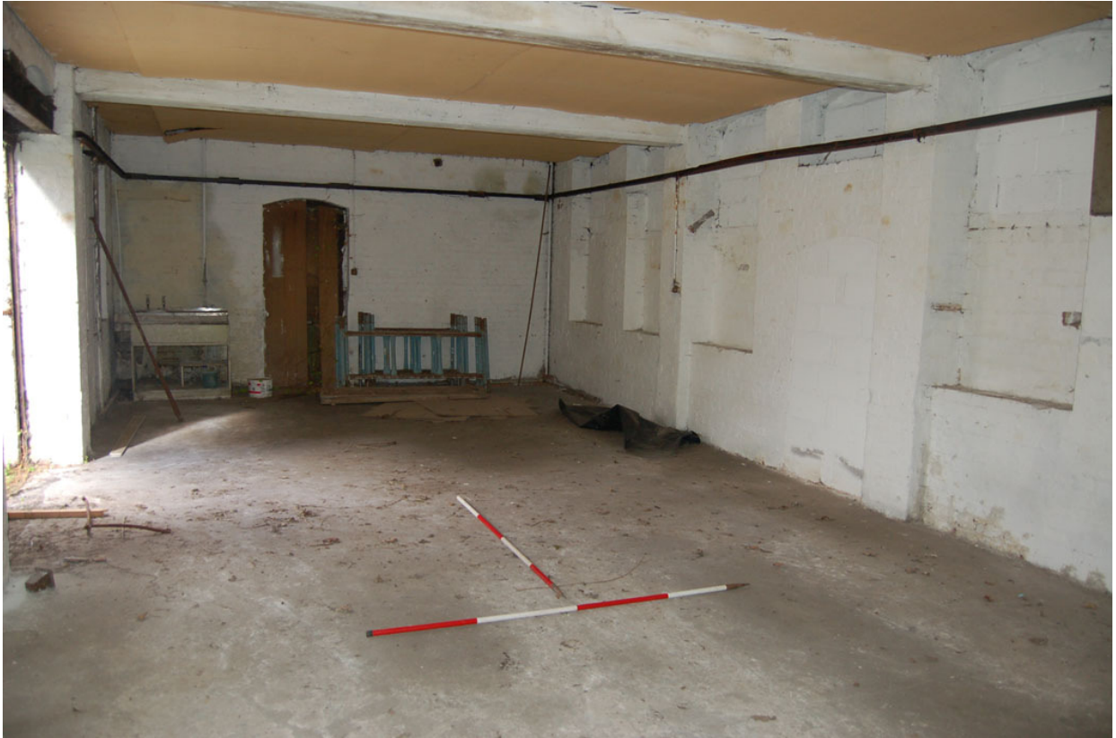
Plate 303: Building E, ground floor looking north; note windows blocked in two phases (right).
