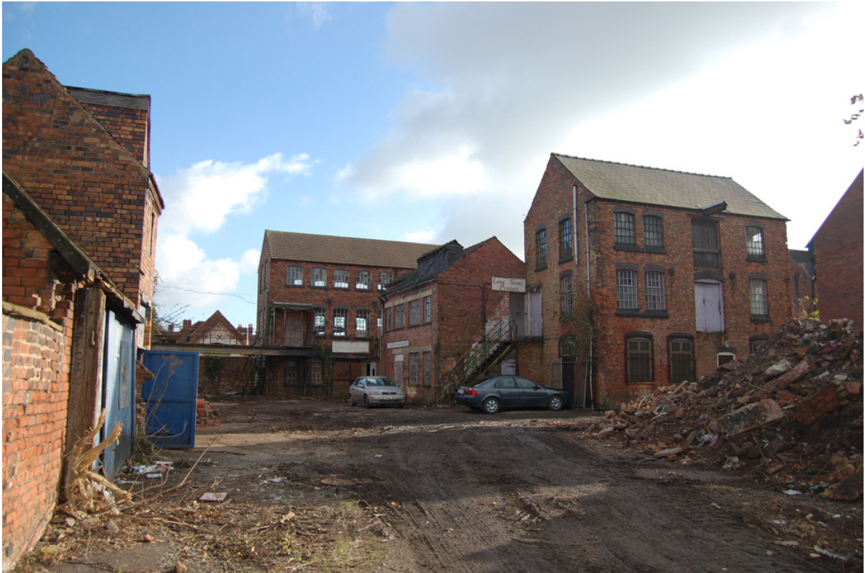
Plate 298: Former hat manufactory; Buildings H, E, F and G (left to right), general view.
