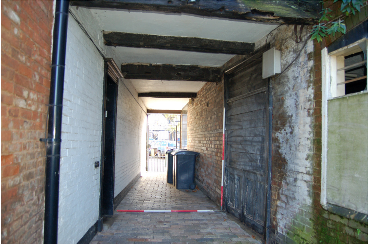
Plate 22: Building A, Block A3; Passage to north of No. 16 Church Street, looking east.
