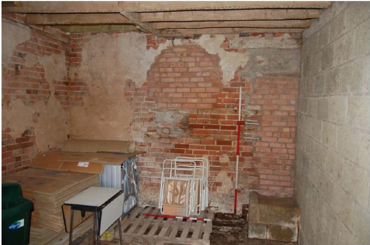
Plate 35: South range, interior; Room GF04 looking west, NB blocked window and door.
