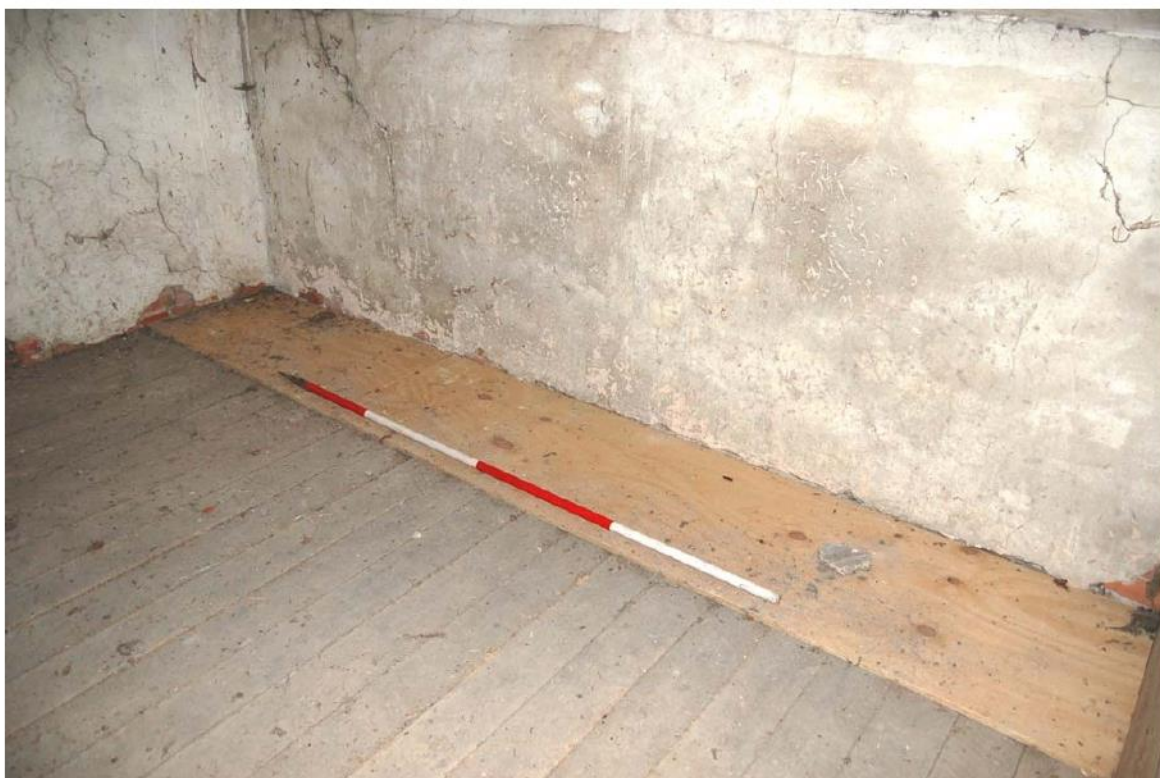
Plate 44: North range, interior; Room 1F03, floor to east side of range (? former feed drop).
