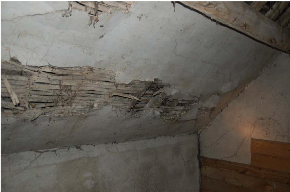
Plate 41: North range, interior; Room 1F03 lath and plaster render to east wall/roof slope.
