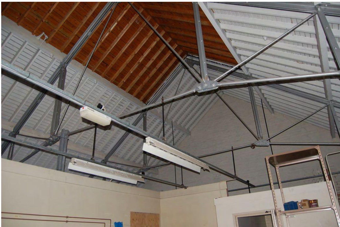
Plate 63: Building 28: rear range, detail of roof, note renewed section between upper purlins.
