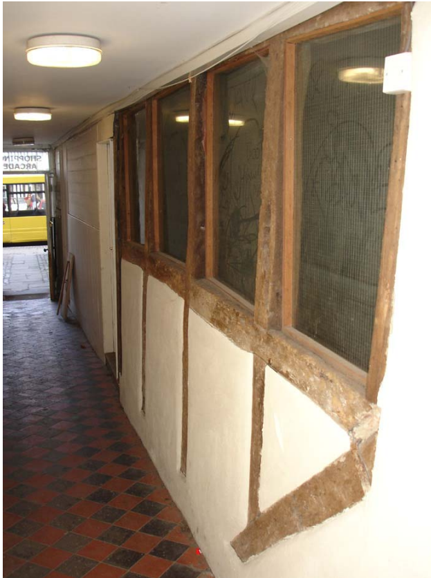
Plate 11: Passageway flanking west side of Arbery's, looking towards Market Place, note C17th framing.
