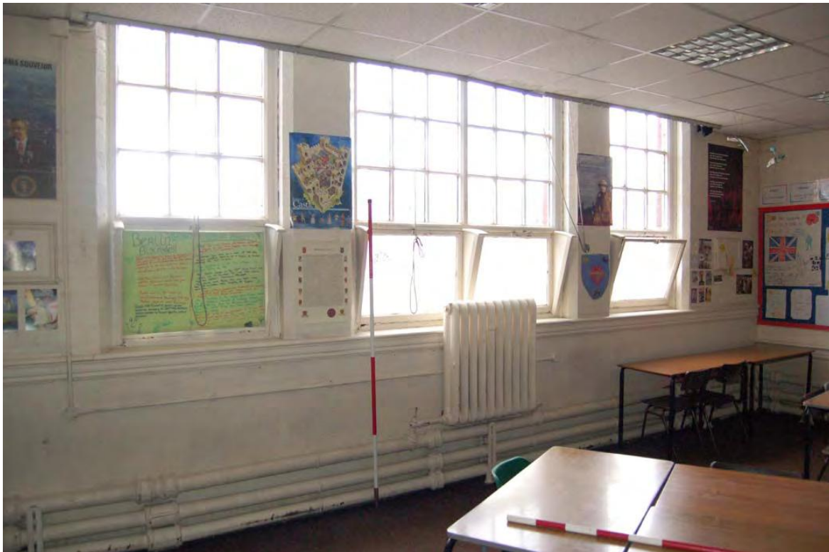
Plate 35: Suspended ceiling cuts across windows within primary classroom.
