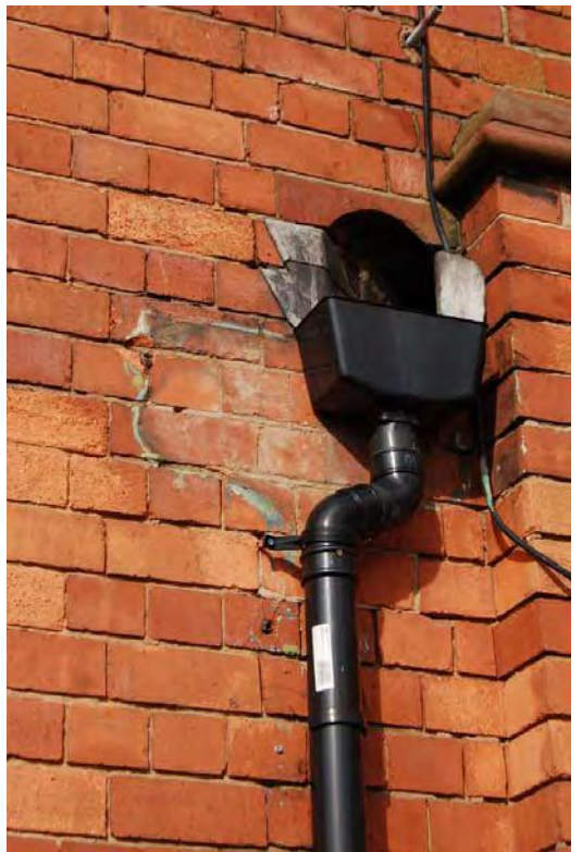
Plate 24: Unsympathetic replacement, NB: note shadow of original hopper.
