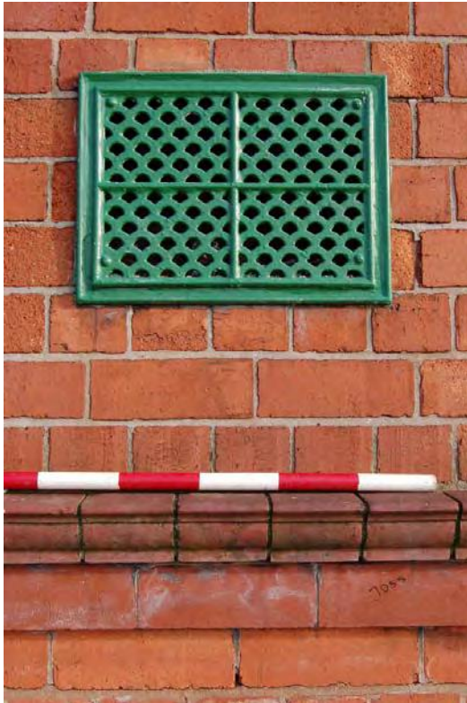
Plate 25: Decorative string and vent/grill.
