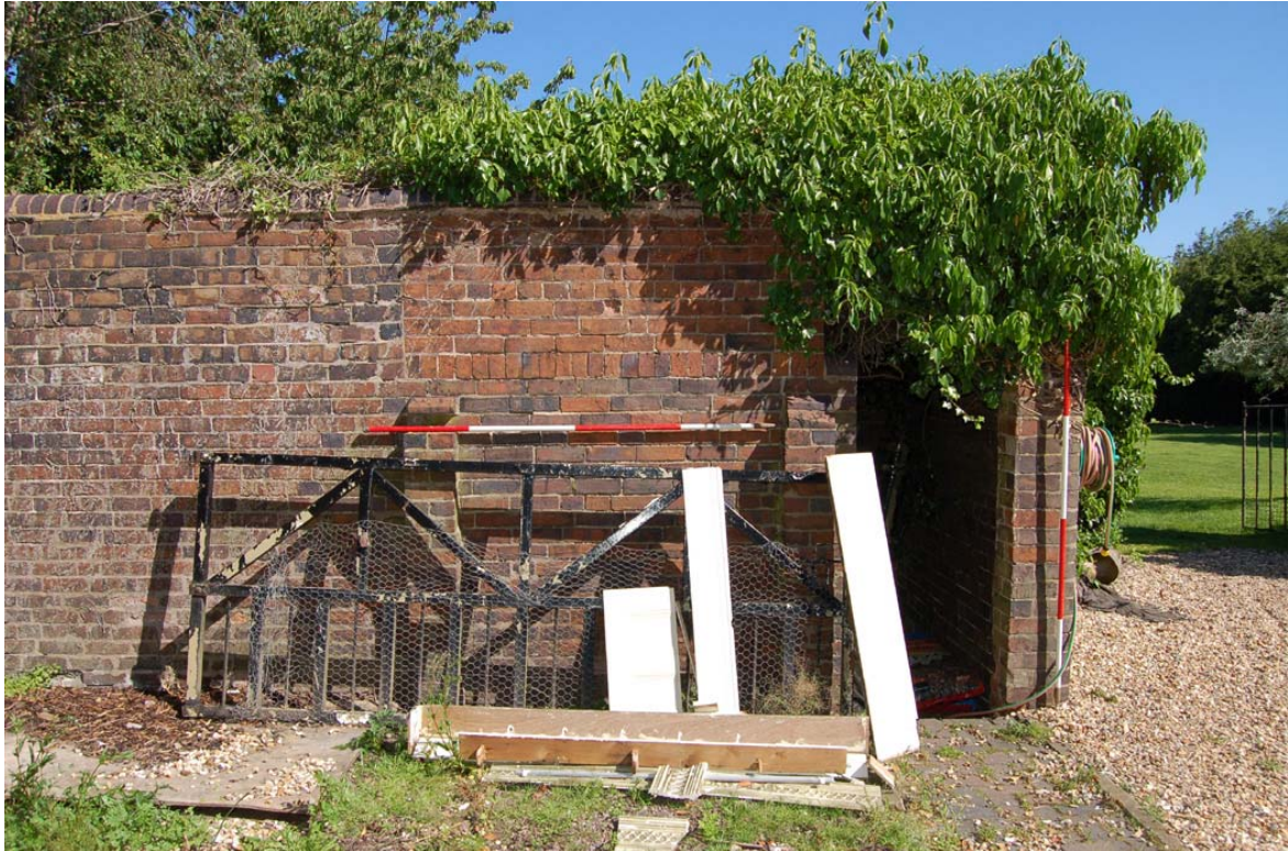
Plate 5: Outbuilding; south elevation, east end: note area of secondary brick to lhs of door.
