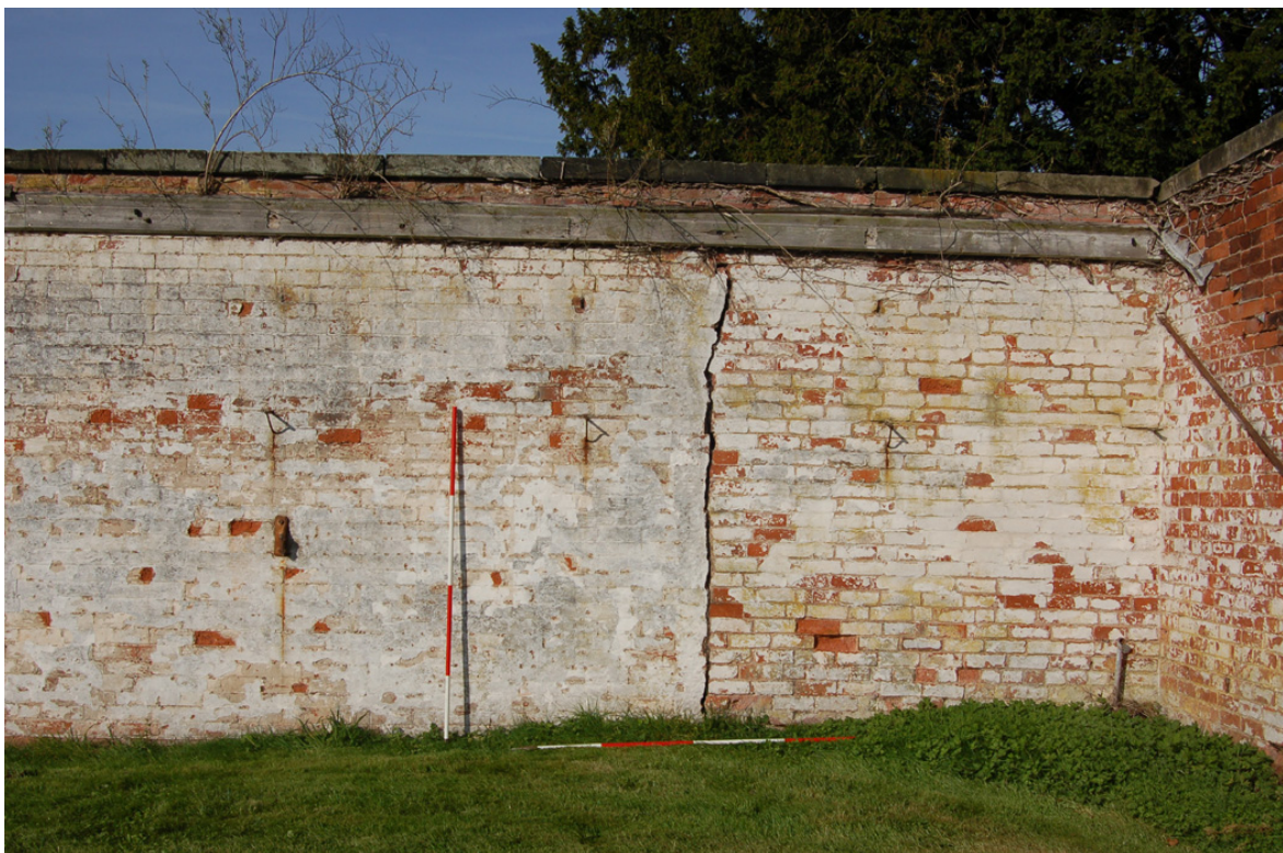
Plate 8: North garden, west wall; brickwork north of gateway (note rebuild to tight).
