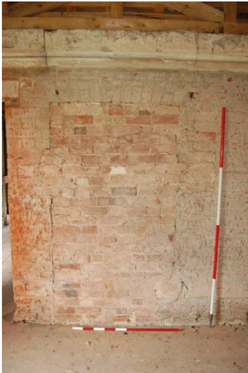
Plate 104: Detail of blocked window/door.
