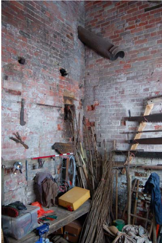
Plate 114: Rm B5; Flue and blocked doorway in south wall at SW corner.
