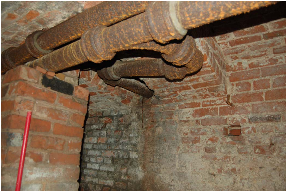
Plate 43: Room B1; secondary piping breaking through primary brick vault.
