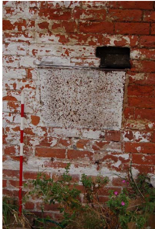
Plate 135: Fe bin set into wall.
