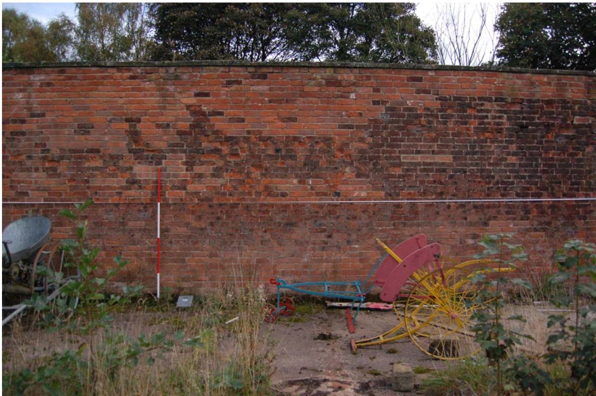
Plate 141: South garden, south wall; representative section of walling. NB. Rebuild of upper wall in paler orange, stretcher bond brick.
