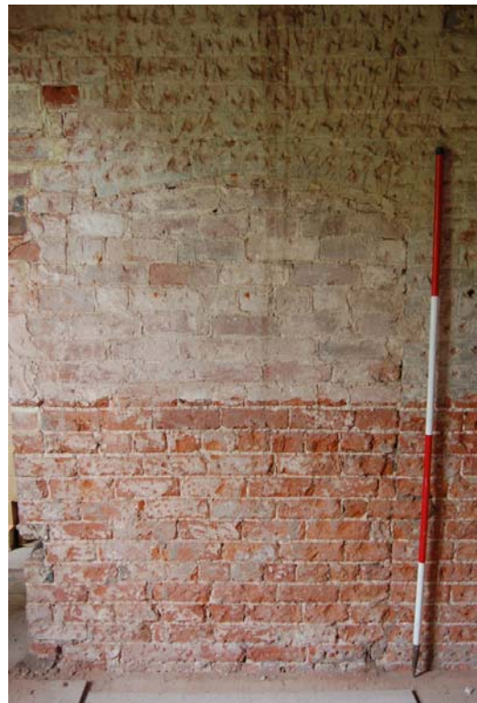
Plate 67: Room G5 (S), blocked door.
