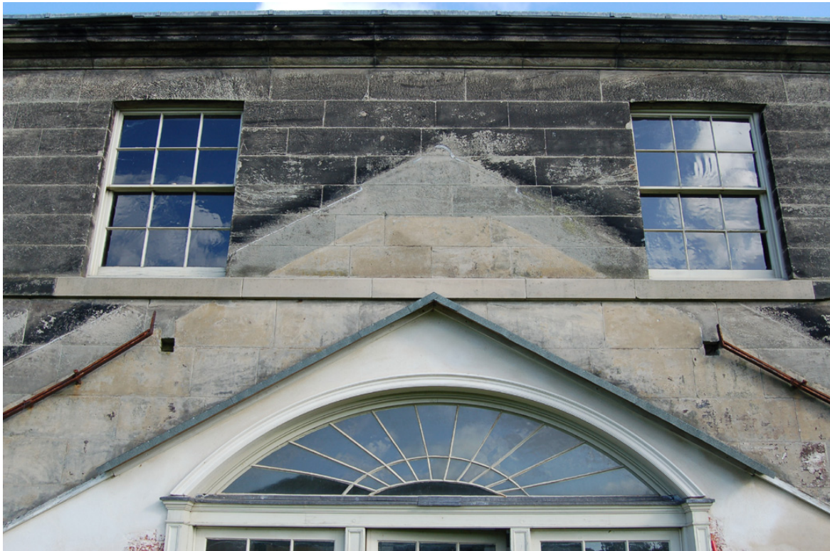
Plate 30: Detail of glasshouse profiles; note upper ridge cuts across corners of windows .
