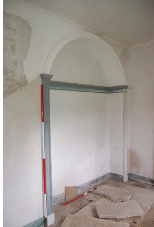
Plate 48: Rm G1, east end recess. ( NB: slabs conceal entrance to mushroom tunnel).
