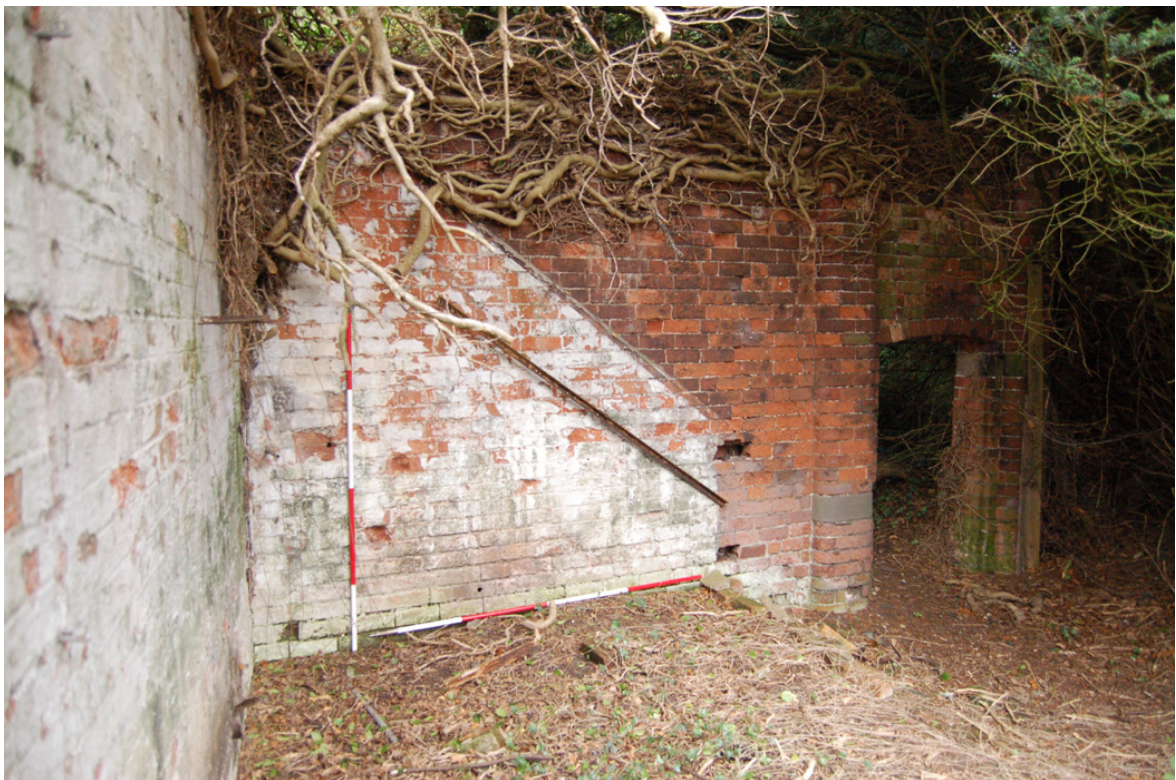
Plate 165: Profile of glasshouse in short section of eastern wall, pedestrian doorway to right.
