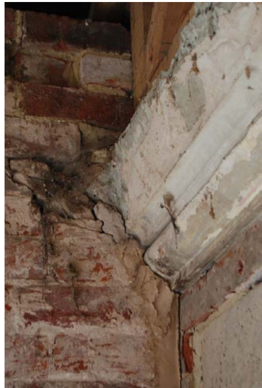
Plate 105: Truncated exterior cornice.
