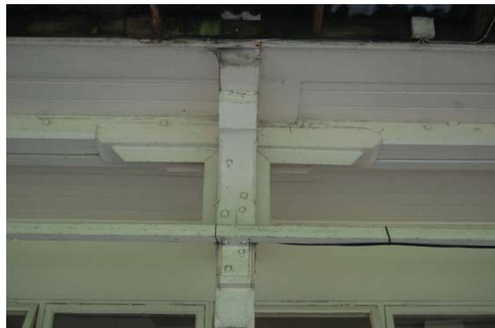
Photo 36: Partially surviving original stanchion and bracket from north.
