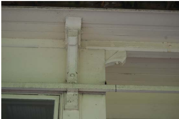
Photo 39: Partially embedded original stanchion and bracket (east) from north.
