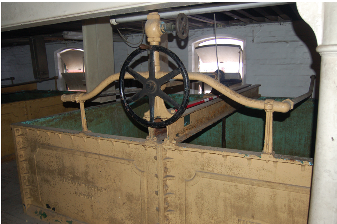
Plate 26: Barley intake range, [3F01]; detail of steeping vessel – water supply and opening mechanism.
