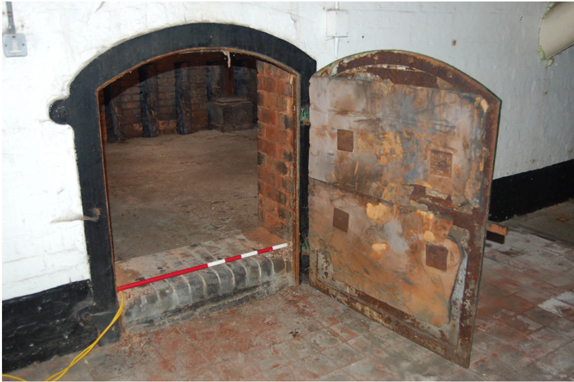
Plate 42: 2F working floor [2F01], east wall; detail of door to heating chamber.
