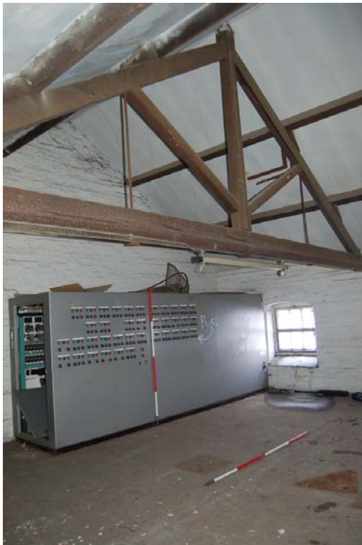
Plate 74: Out-loading bays, [3F05] roof and switchgear.
