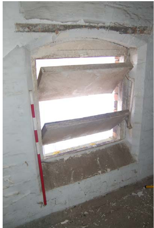
Plate 16: Primary window with boarded lights.
