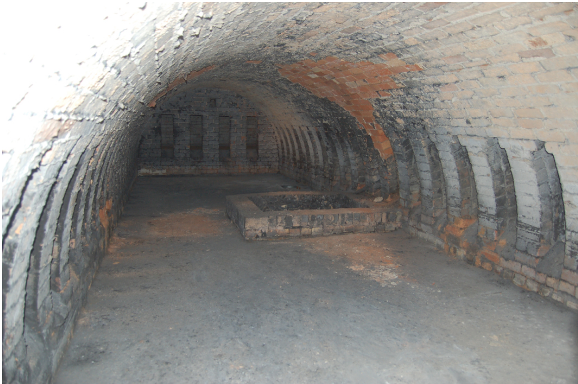
Plate 62: Heat chamber [2F02]; detail of interior of disperser with central flue opening.
