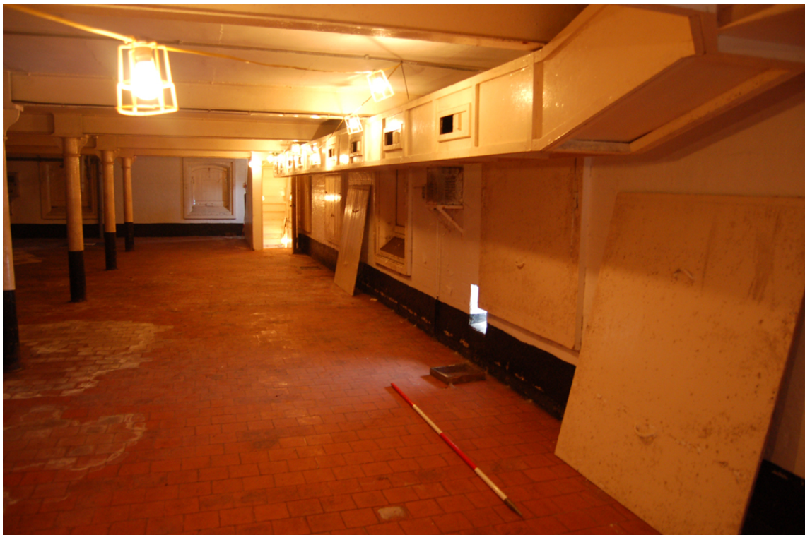
Plate 45: Working floor [1F01]; secondary ducting looking west.
