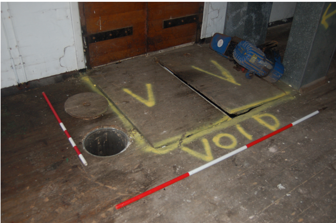
Plate 36: Working floor [3F02]: timber hatches and chute cover before kiln floor doors.
