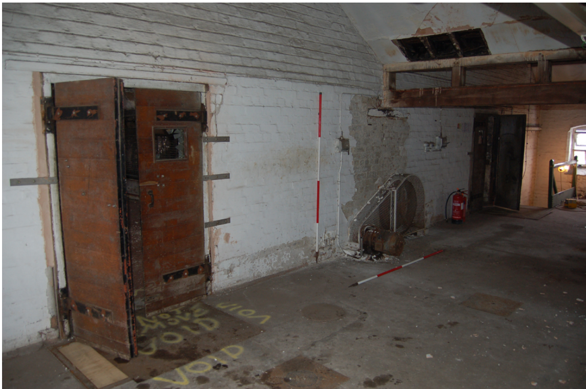
Plate 73: Eastern out-loading [3F05]; west wall with doors to kiln floors and engine / drive wheel for north kiln turner mechanism (centre).
