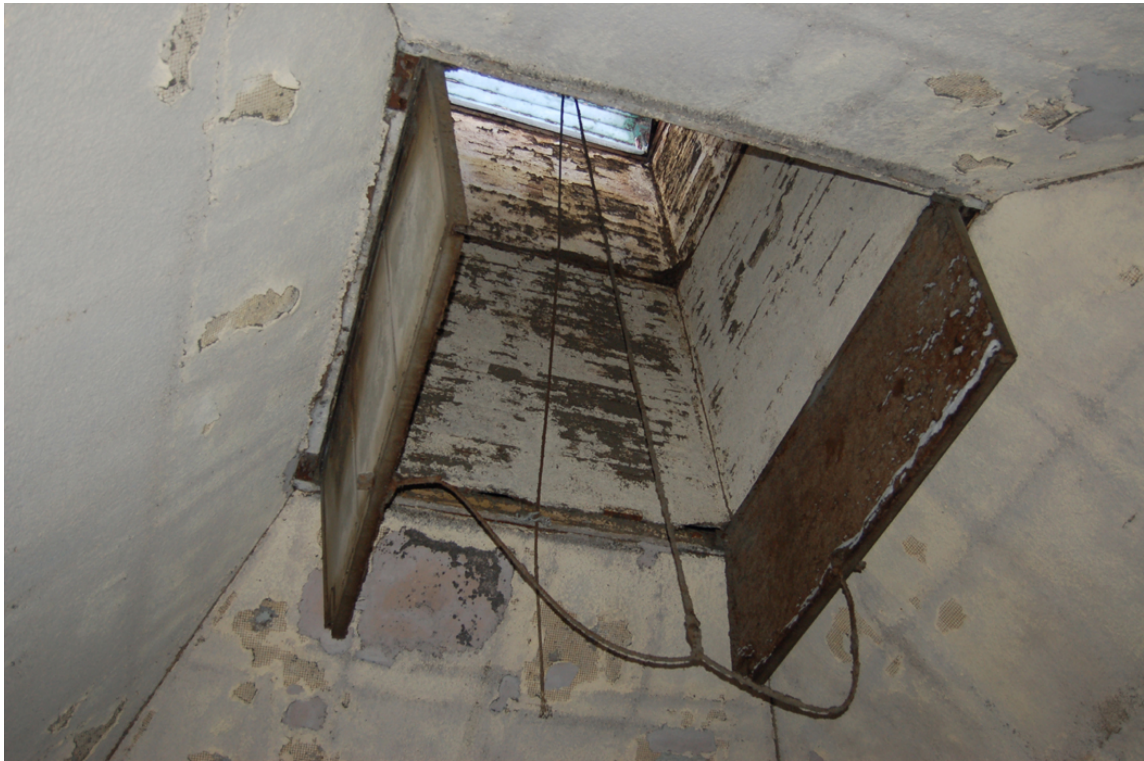
Plate 72: Smoke evacuation shutters.
