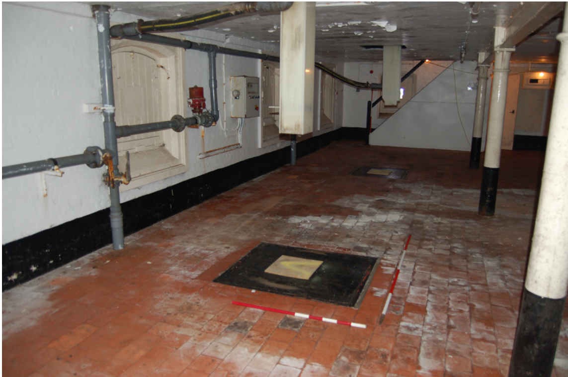
Plate 44: Grain intake range, [1F01]; detail of floor voids below steeping vessels at Bay 1.
