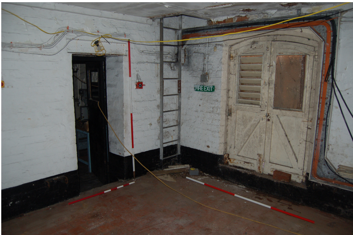
Plate 47: Working floor [GF01], south-east corner: door to kiln range (left), fire escape ladder (centre) and door to exterior (right).
