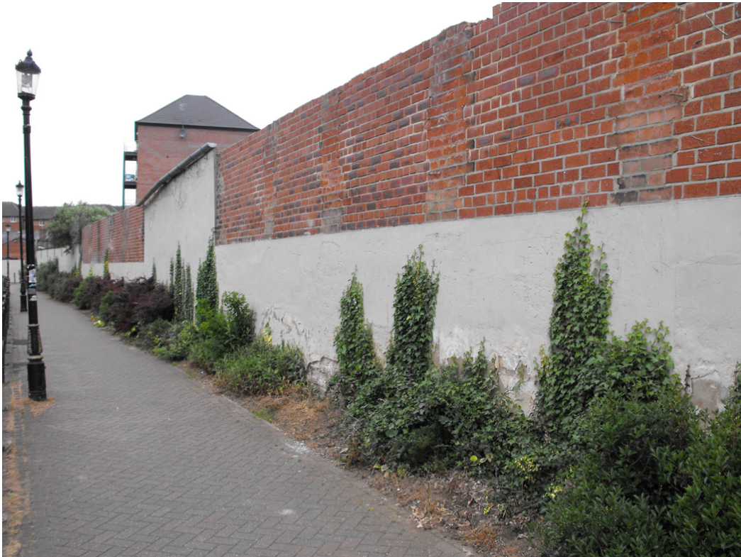
Plate 5: General view looking north-west along Brook Walk, site bounding wall to right.
