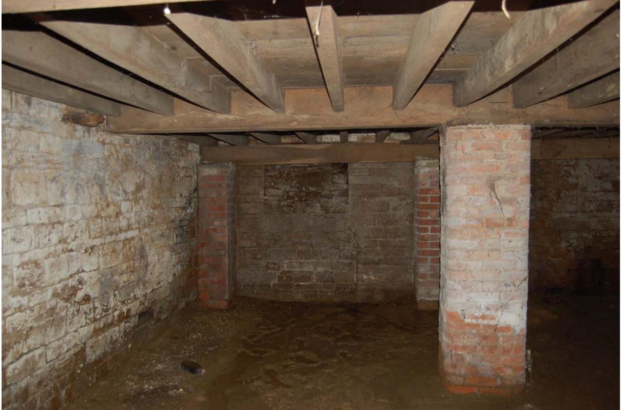
Plate 38: Basement Room [B01]; general view looking east, note blocked window to left.
