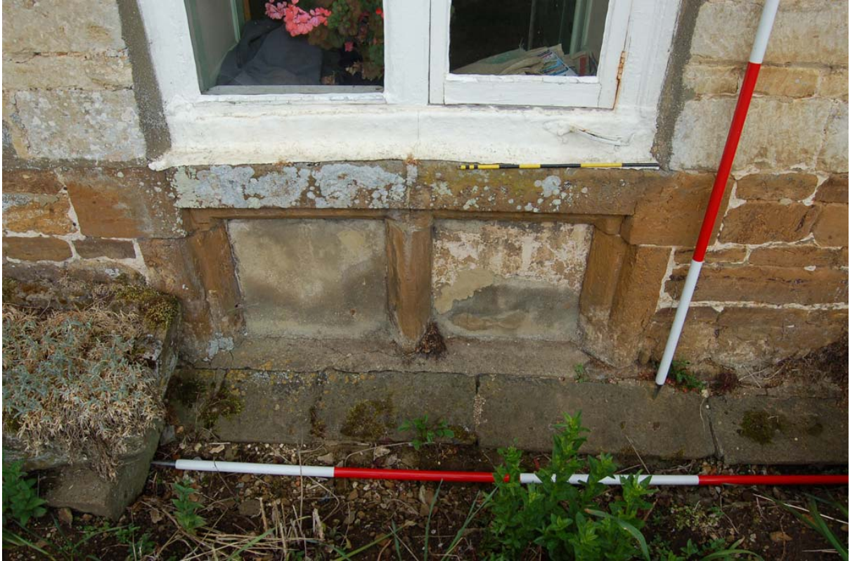
Plate 11: Detail of blocked basement window.
