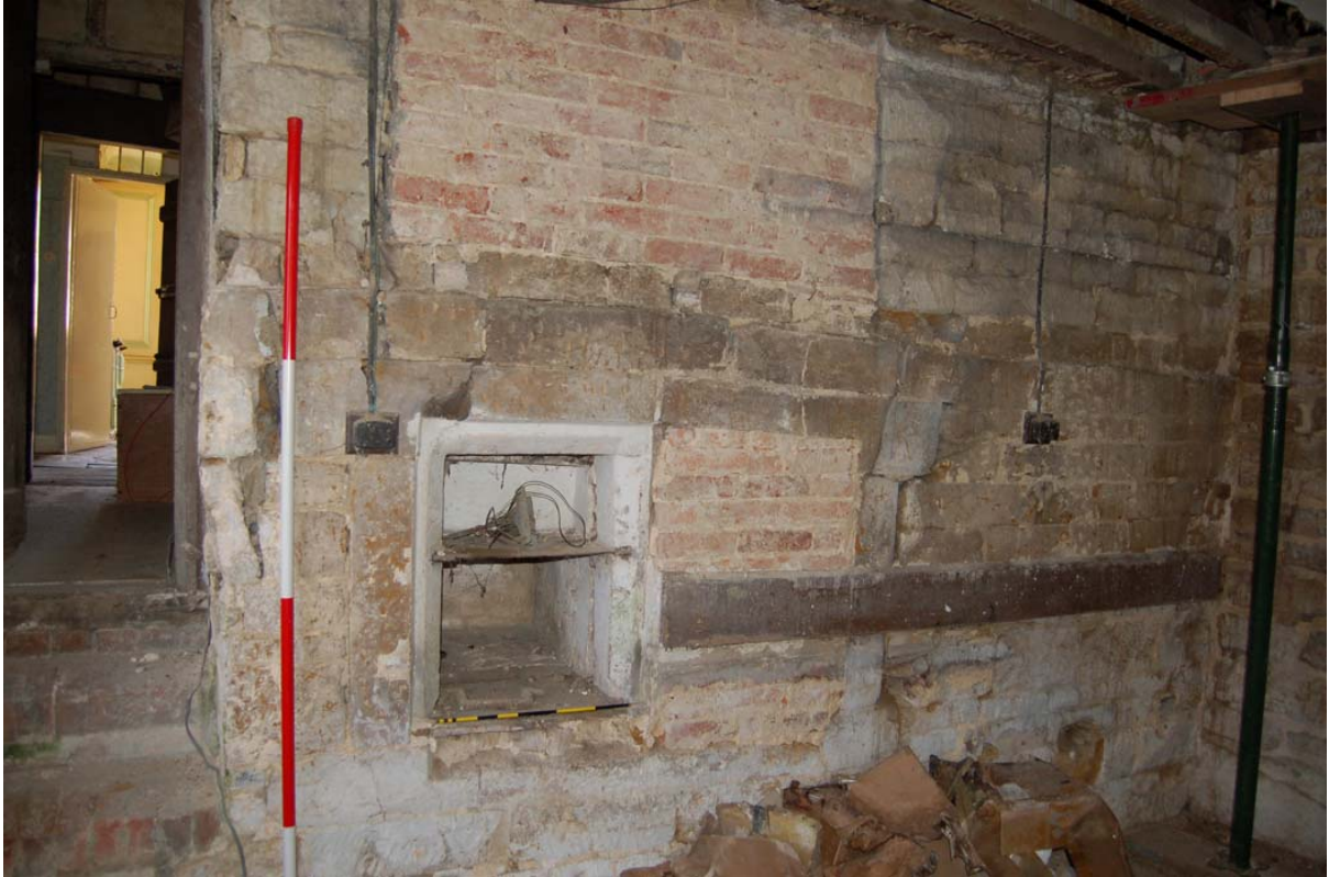
Plate 34: Room [GF11], east wall showing recess (former cellar window) and blocked GF window Over (brickwork).
