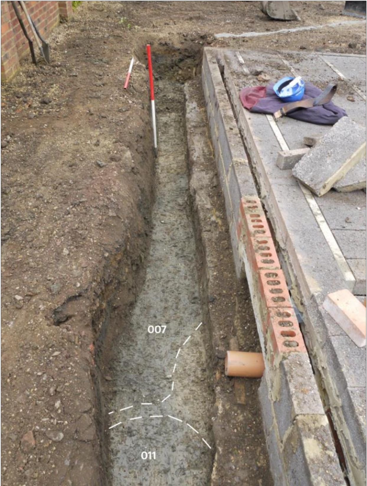
Figure 15. Overview of drainage trench along the west side of the new building showing exposed medieval pits [006] and [009]. Facing north-northeast
