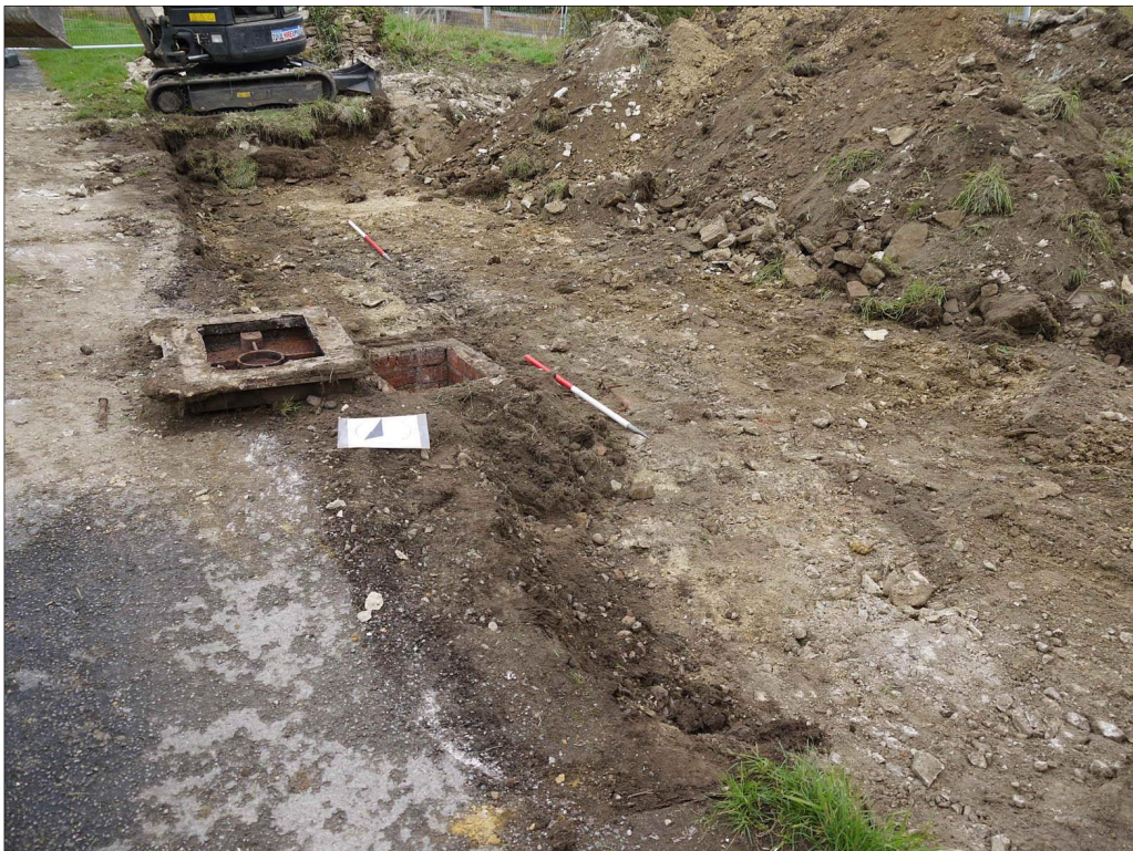
Figure 5. Overview of central strip facing N, showing extent of modern drainage disturbance
