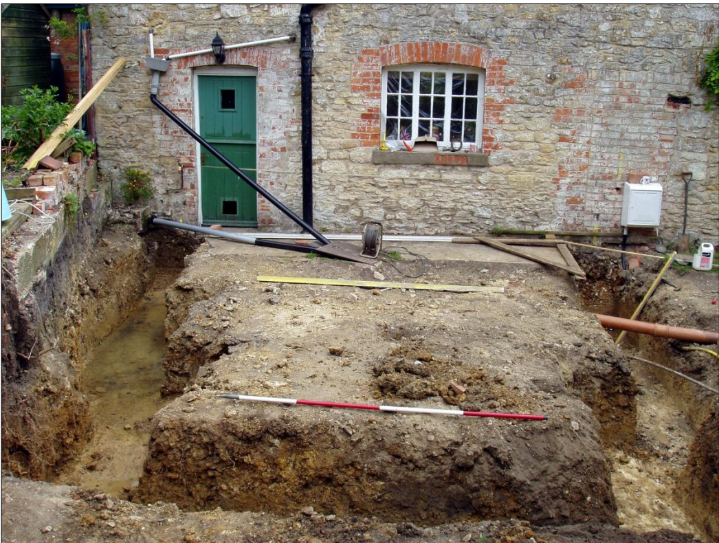
Figure 4. Viewpoint 1 (top): overview of site prior to excavation, facing SW. Viewpoint 2 (bottom): overview of foundation trenches, facing NW
