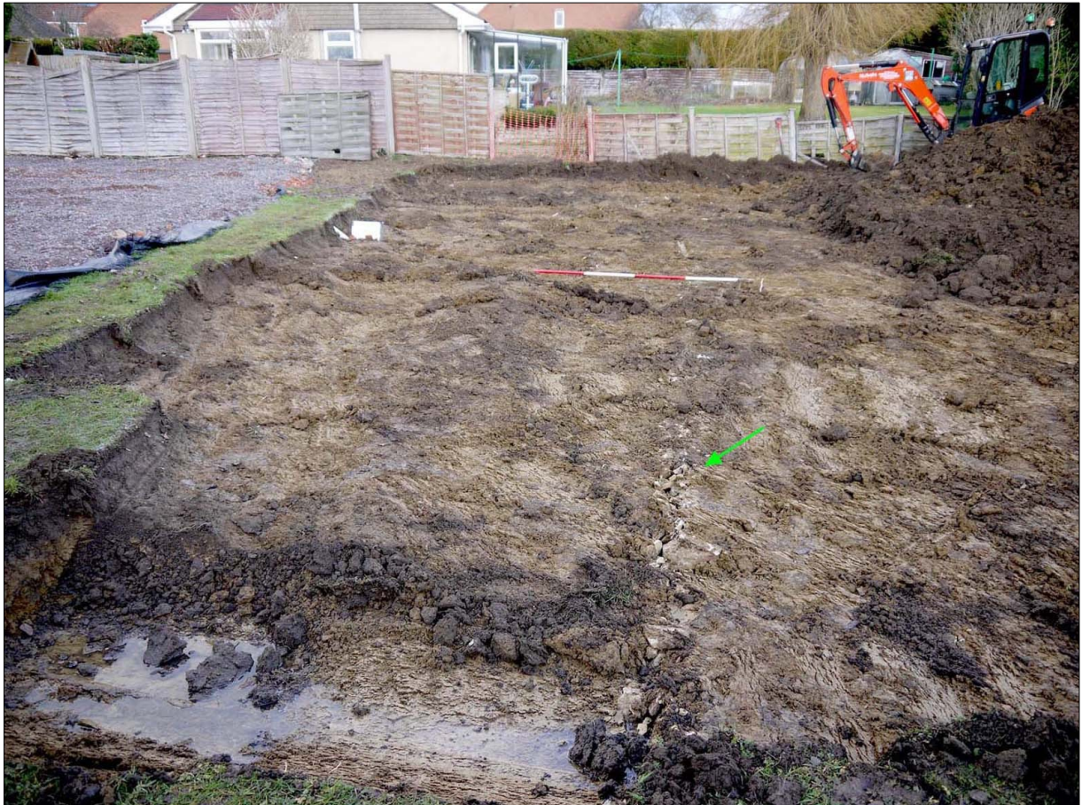
3. Overview of site after ground reduction. Green arrow marks position of stone field drain. Facing NE
