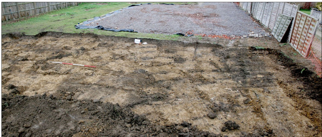
4. Overview of site after ground reduction, facing NW. Dark brown patches in central area and at top right denote recent grubbing out of trees
