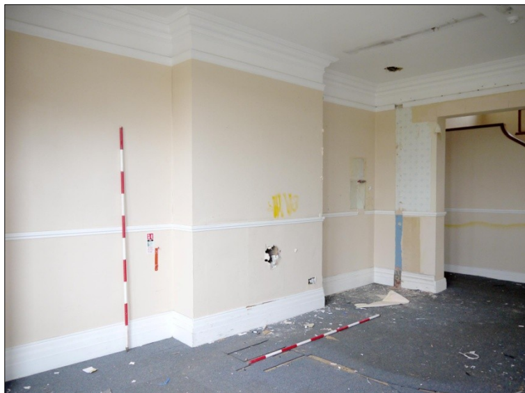
84. N-S Wing. Room 5. Chimney breast with blocked fireplace in north wall. Facing NE
