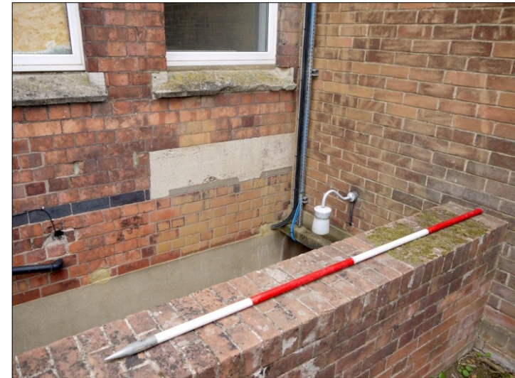
38. Stone mullioned lintel (with blocking) denoting former lights of lower ground level. Facing N
