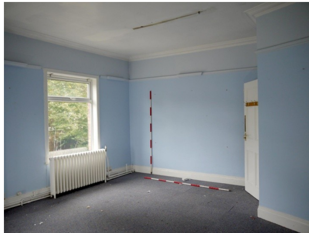
135. N-S Wing. Room 17E (bedroom). Entrance from corridor to right. Facing SE.
