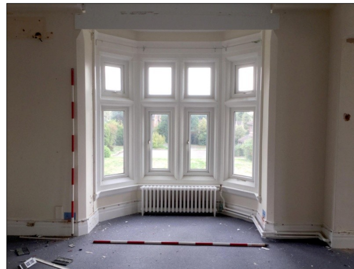
112. E-W Wing. Room 14. Bedroom. 3-sided bay window overlooking rear garden. Facing SW
