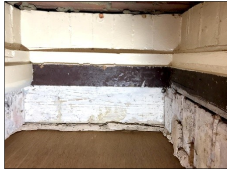
91. Room 6. Upward view inside former window opening. Outer brick walls at top
