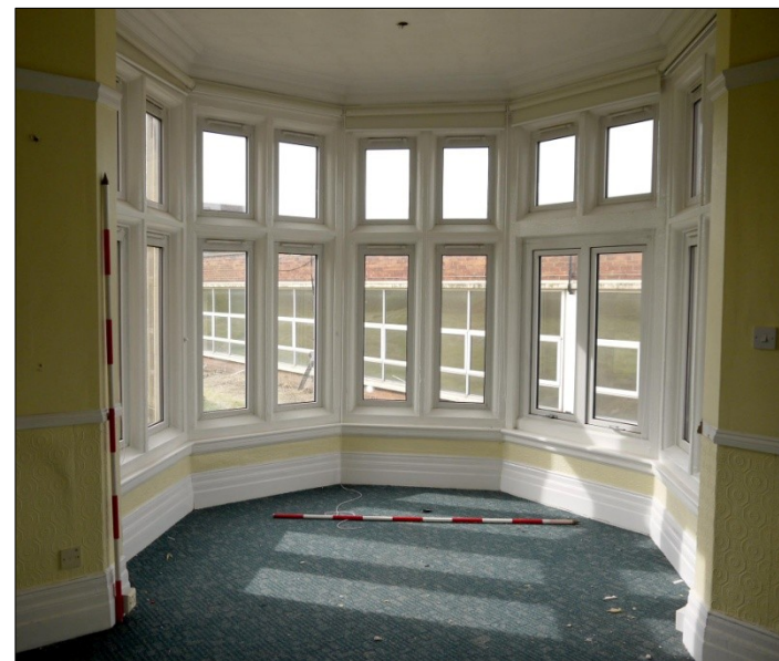
71. E-W Wing. Room 4. Living room. 5-sided bay window (SW turret) with former access to rear garden (see also photos 72 and 25-27). Facing SW
