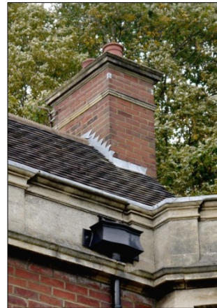
10. E-W wing, view of chimney and cast-iron rainwater hopper head. Facing NE
