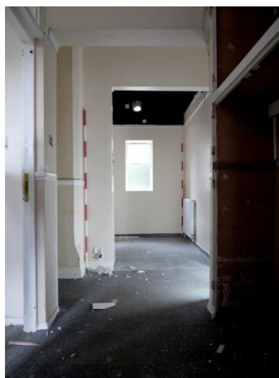
87. N-S Wing. Passageway between Rooms 5 and 6. View across central corridor to Room 9. Facing E
