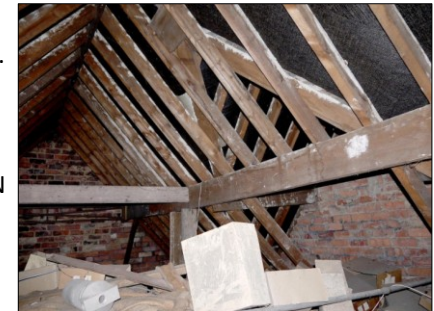
143 (top) & 144 (bottom). N-S Wing. Roof frame (east side of roof) Facing N
