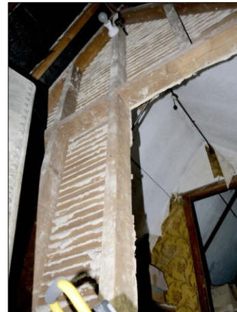
142. N-S Wing. Attic room. Stud wall with plaster & lath infill. Facing SE
