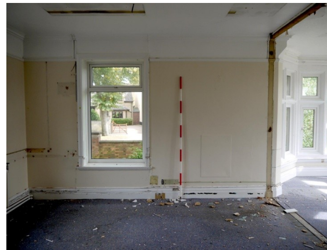
100. E-W Wing. Room 12. Position of former fireplace on right side of ranging rod. Facing E
