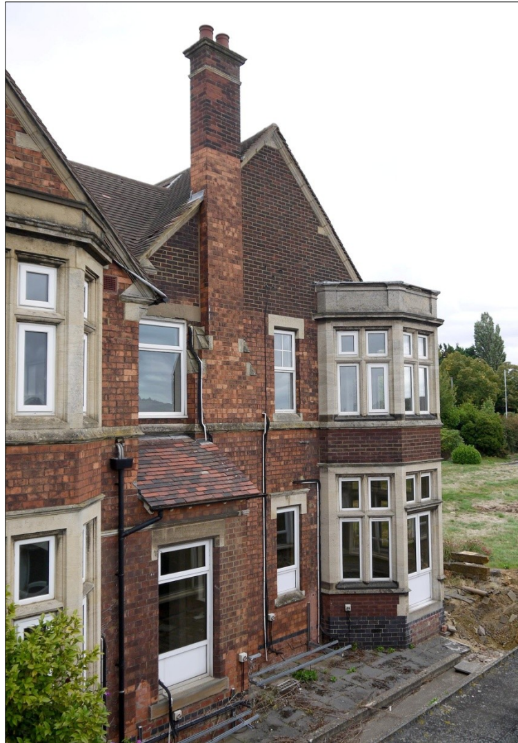
29. N-S wing. Brick colour (orange-red) distinguishing the late 19 th house from the early 20 th century enlargement. Facing SE
