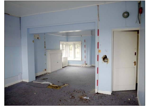
139. N-S Wing. Room 17W (bedroom). View towards Room 17E. Entrance from to right. Facing NE
