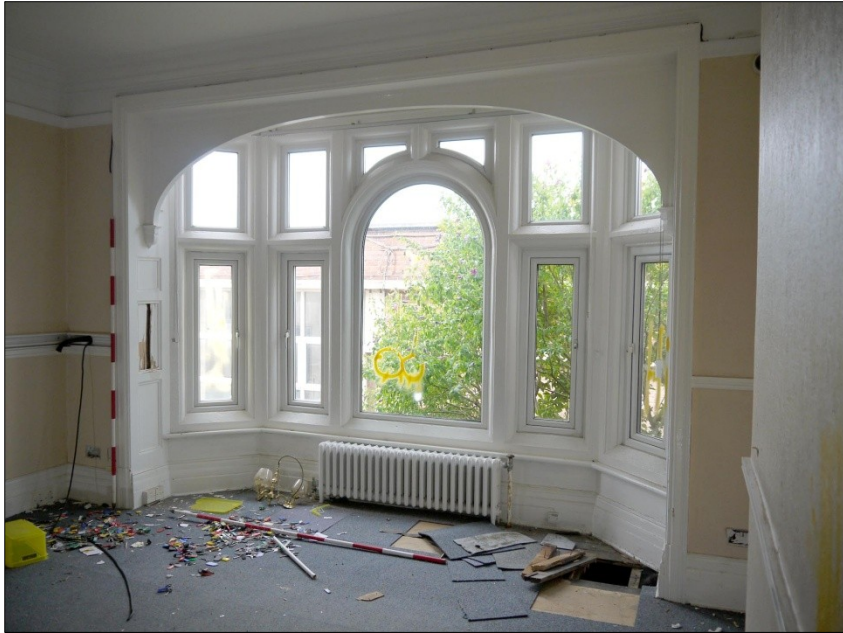
79. N-S Wing. Room 5. Bay window of original C19 house with moulded pelmet. Facing SW
