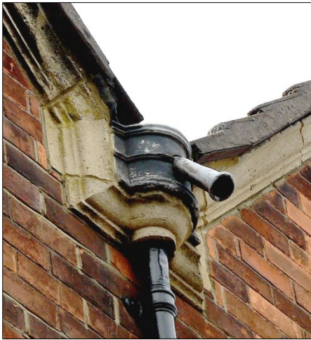
47. North elevation. Cast-iron rainwater outlet. Facing SW
