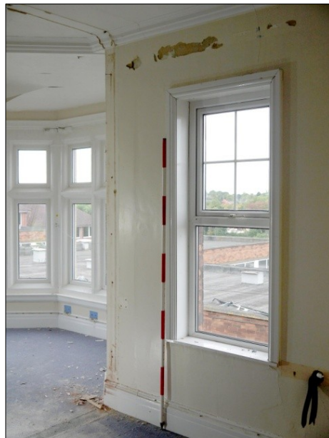
114. Room 14. Sash window in west wall (SW corner of original C19 house). Facing SW
