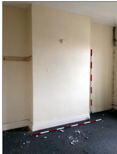
126. N-S Wing. Room 16. Chimney breast /blocked fireplace in south wall. Facing SW
