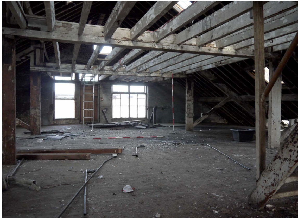
56. Third Floor. Overview of NW end from top of stair. Stair to Fourth Floor at R (Floorboards have been removed on Fourth Floor). Facing NNE
