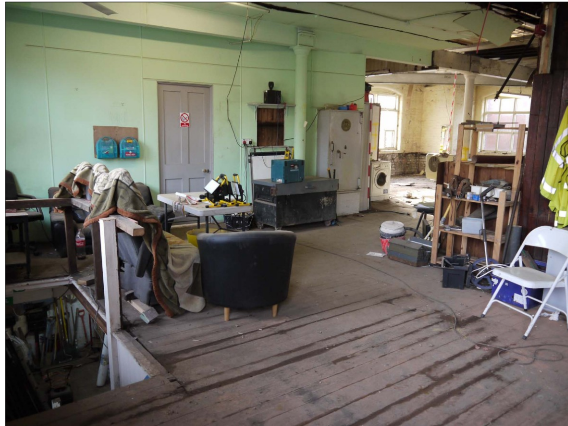
41. First Floor. Former office area. Former office stair to L. Facing SW
