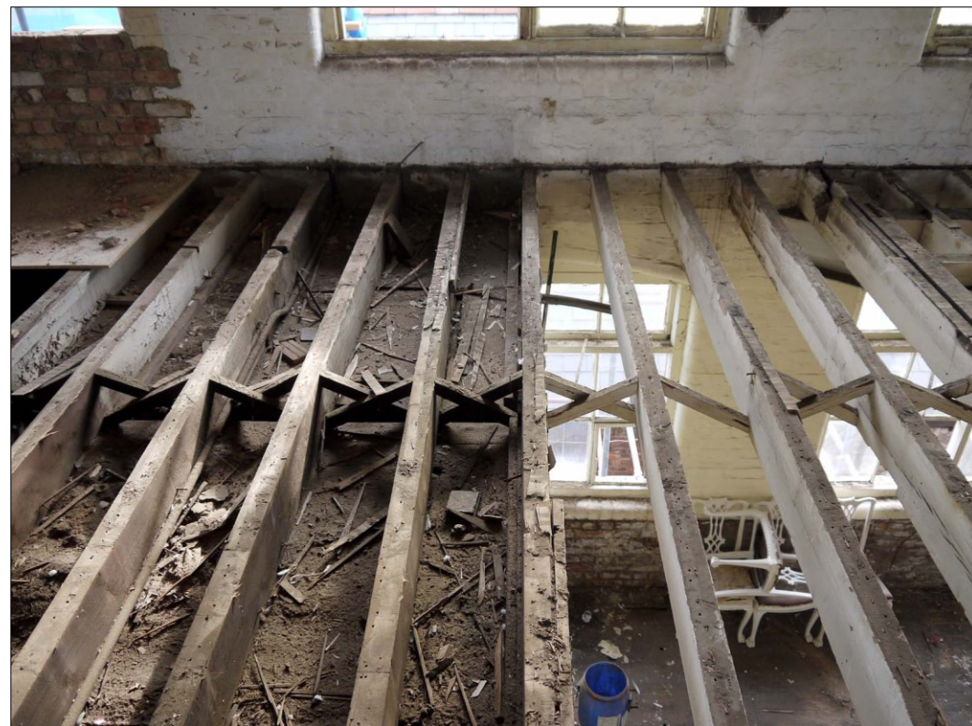
52. Second Floor. SE end. Exposed joists with herring bone struts. Facing SSE
