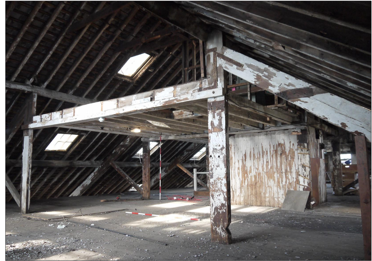
65. Third Floor. Overview of SE end and truss. Lift shaft background R. Facing NW
