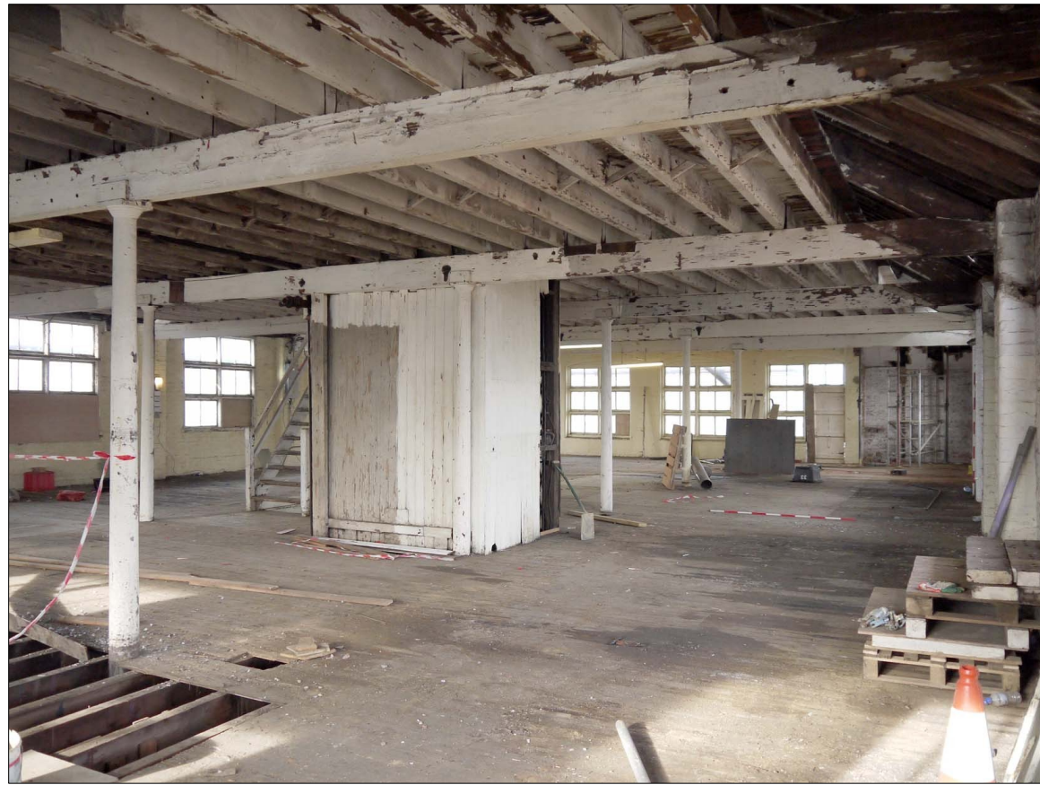
50. Second Floor. Overview from SE end. Lift shaft in centre. Facing NW
