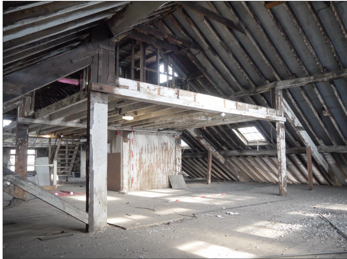
64. Third Floor. Overview of SE end and truss. Lift shaft background centre. Facing NE
