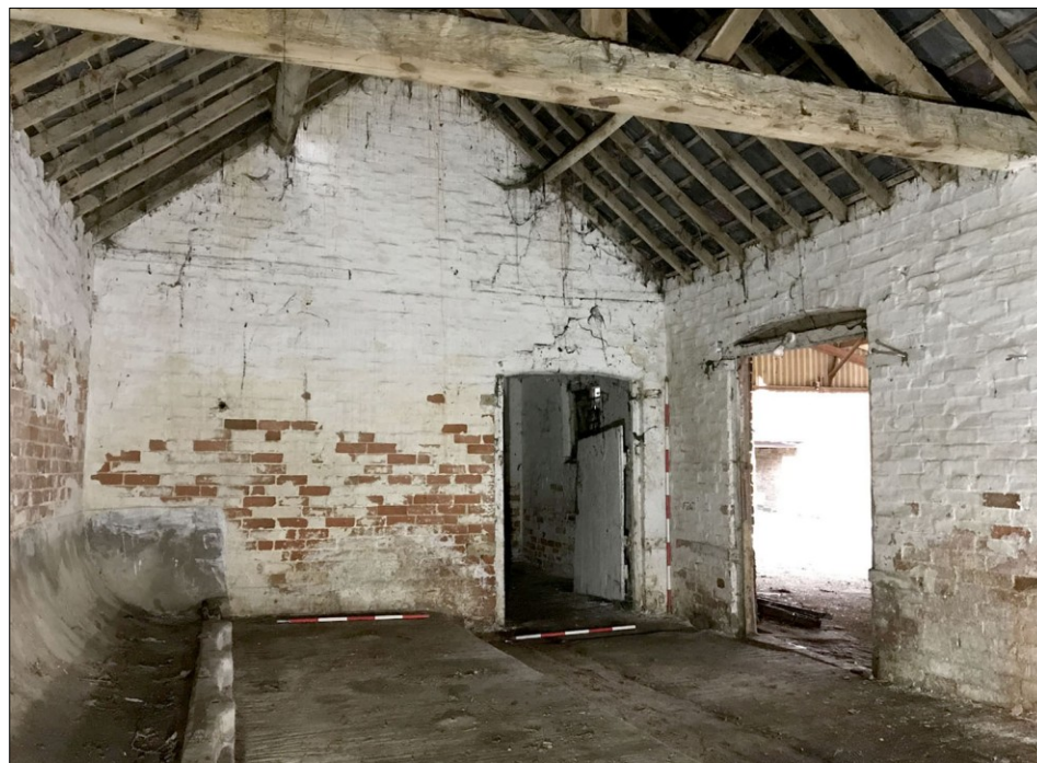
48. Interior of the Building 3, cow house/milking parlour. Trough manger to L. Facing E
