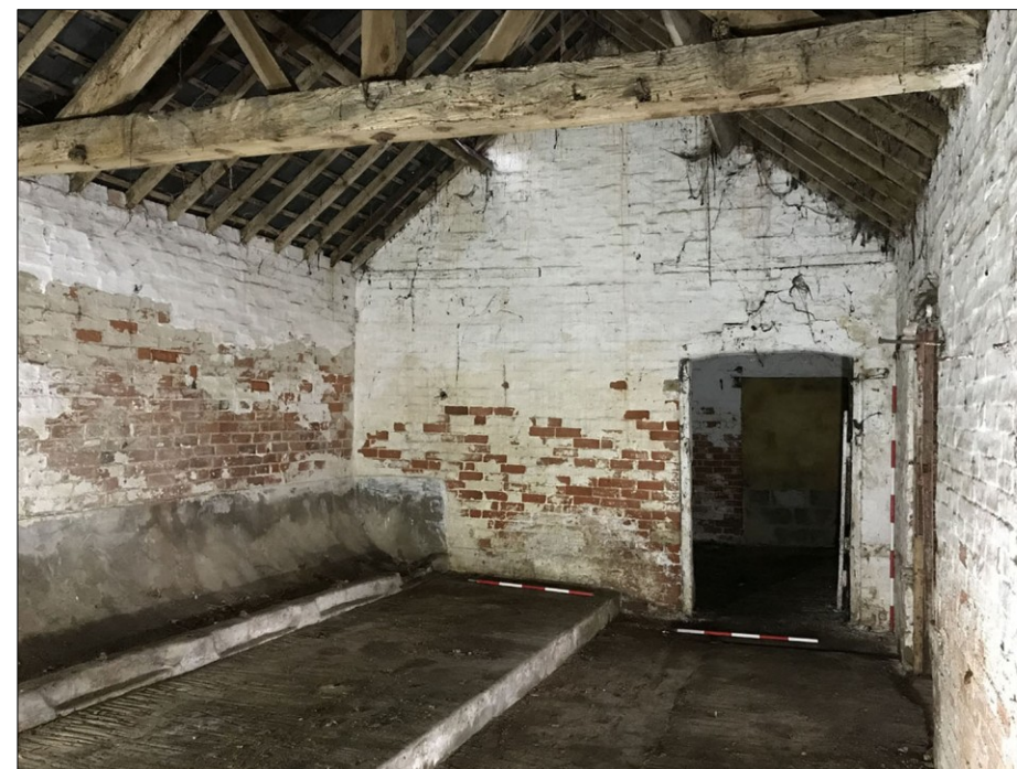
49. Interior of the Building 3, cow house/milking parlour. Trough manger to L. doorway to Building 2. Facing NE
