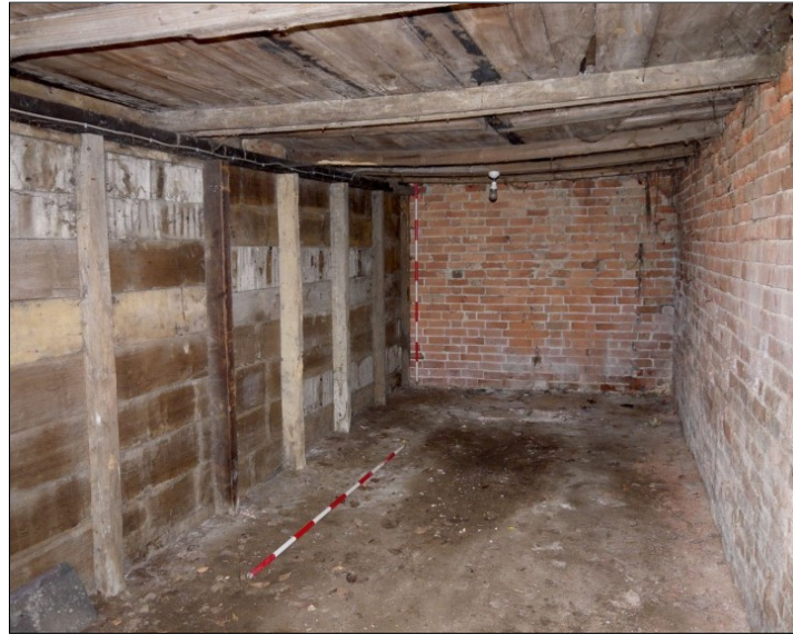
51. Building 4. Partitioned vehicle lock-up at the SW end of the Open Shelter. Facing SE
