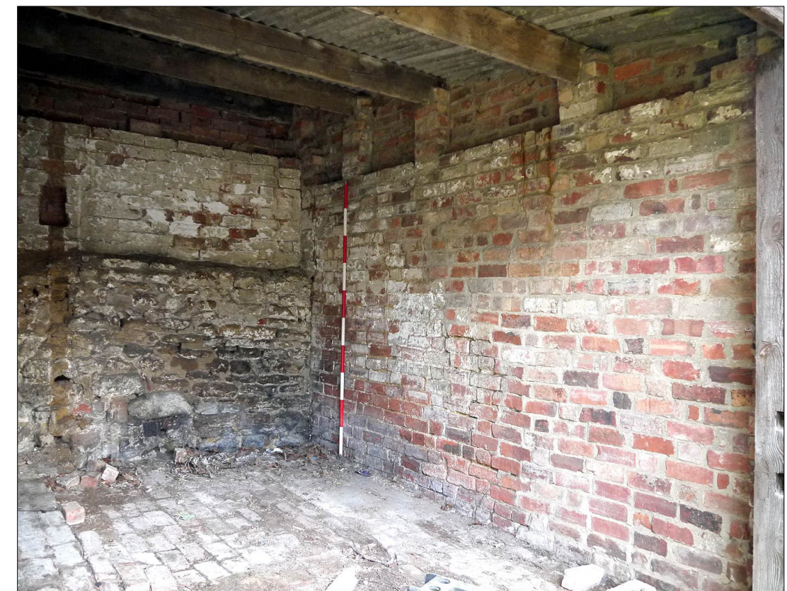
64. Open-fronted lean-to (vehicle store) attached to SE gable end of Building 1 (the stone barn). Facing E
