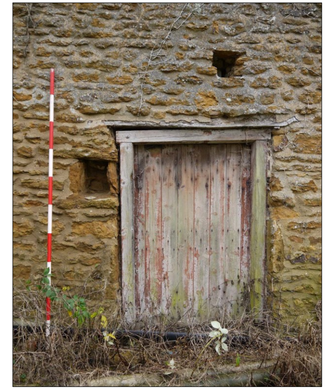
10. Building 1 (the stone barn). Loading door in NW gable end. Facing SE
