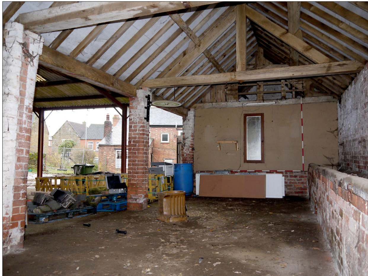
54. Interior of Building 5 (open-fronted cow shelter), facing SE. Manger to R. Rear of farmhouse visible outside in background
