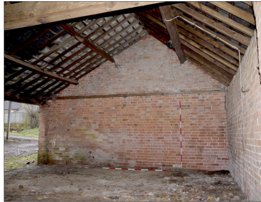
52. Interior of Building 4 (open shelter). Looking towards the rear wall of Building 3 (the Milking Parlour) Facing NE
