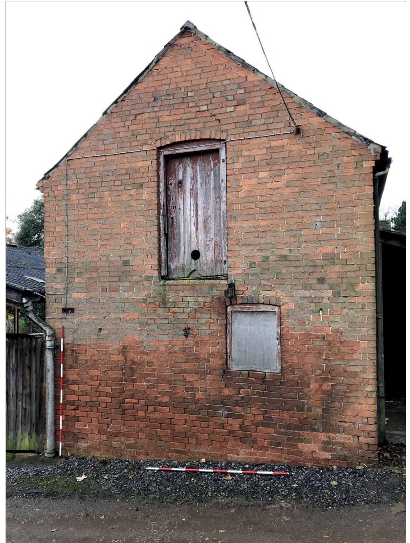
14. Building 2 (cow house), NE gable end with hayloft door and lower light in cow house. Facing SW
