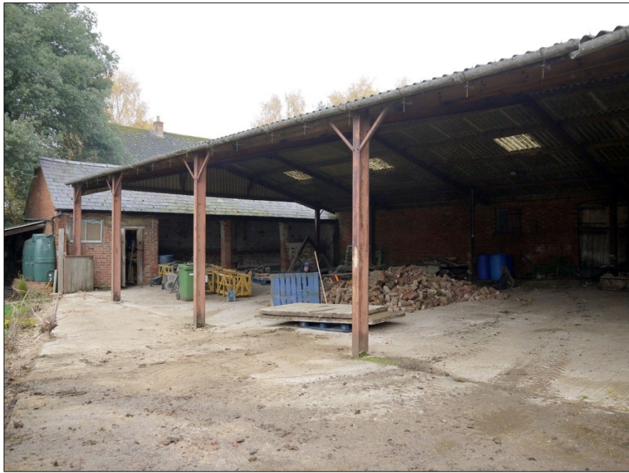
20. View towards Building 5 (open-fronted cow house) through mid-C20 open-sided yard barn. Facing SW
