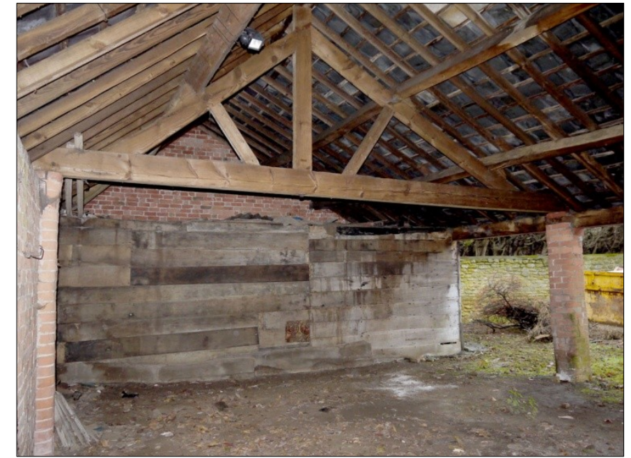
53. Interior of Building 4 (open shelter). Looking towards the timber partition wall of the vehicle lock-up at the SW end. Facing W
