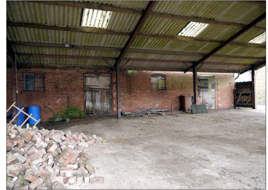
22. View of the frontage of Buildings 2 and 3 (cow houses/milking parlours) through mid-C20 open-sided yard barn. Facing N
