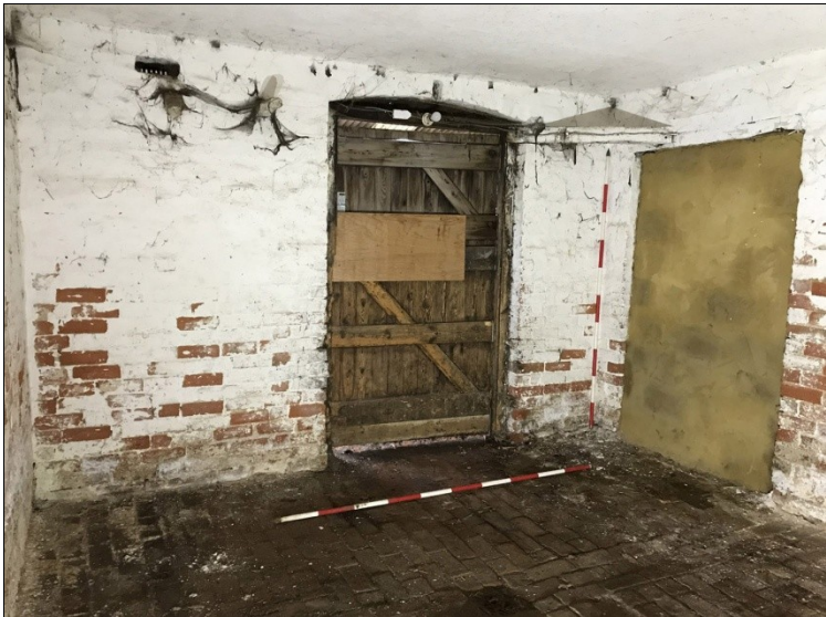
40. Interior of the loosebox, NE end of Building 2. Entrance from the yard and blocked doorway (R) to the SW box (milking parlour). Facing SE
