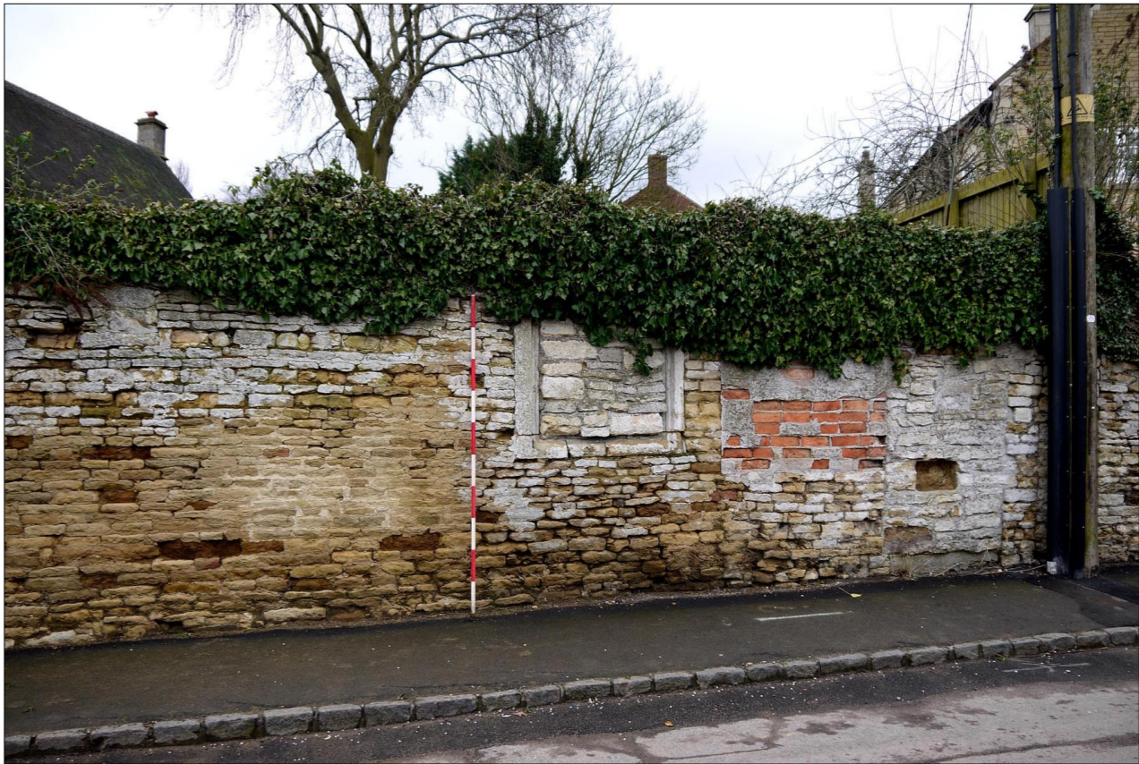
Figure 4. The boundary wall of the Application Site on High Street, incorporating blocked windows and door. Top: facing SE. Bottom: facing NE
