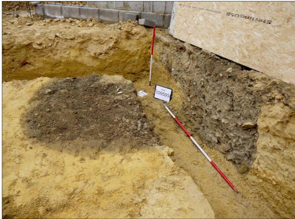
Above. 12.06. 2020. Western end of the cellar. The upper part of Section 3 to right
