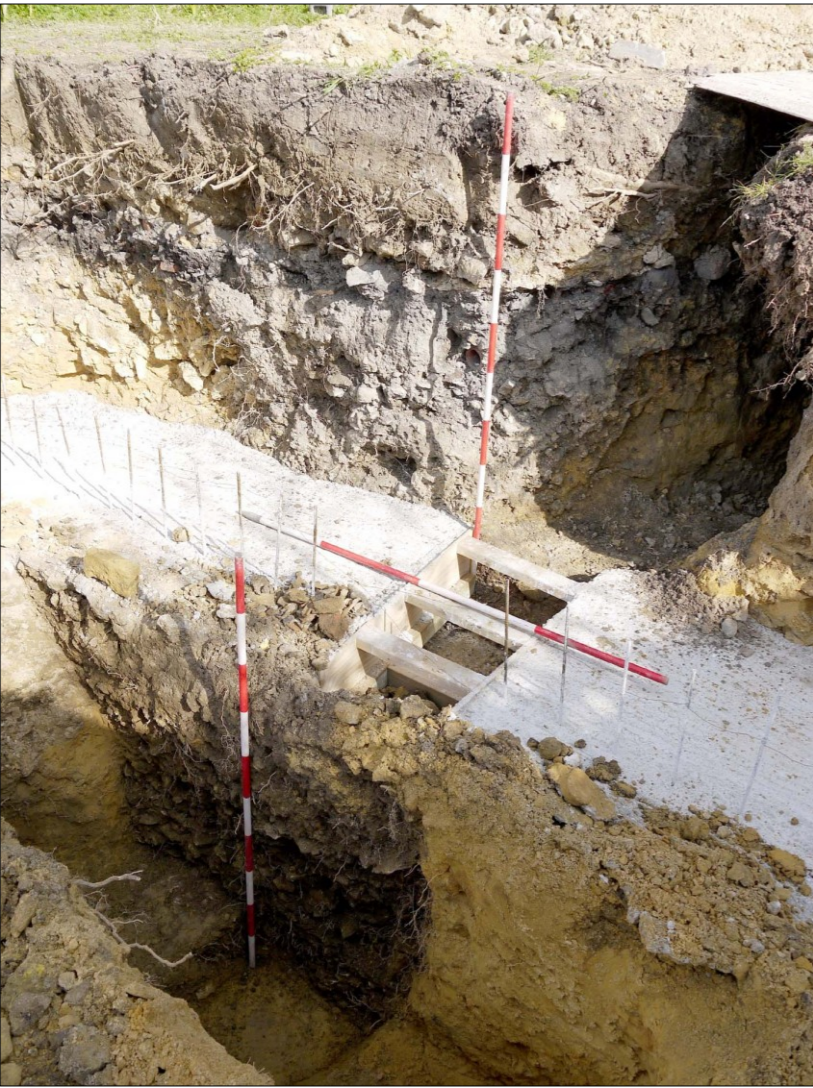
Left: 23.03.2020. View to NE after completion of retaining wall foundations. Section 1 in the background, Section 3 in foreground
