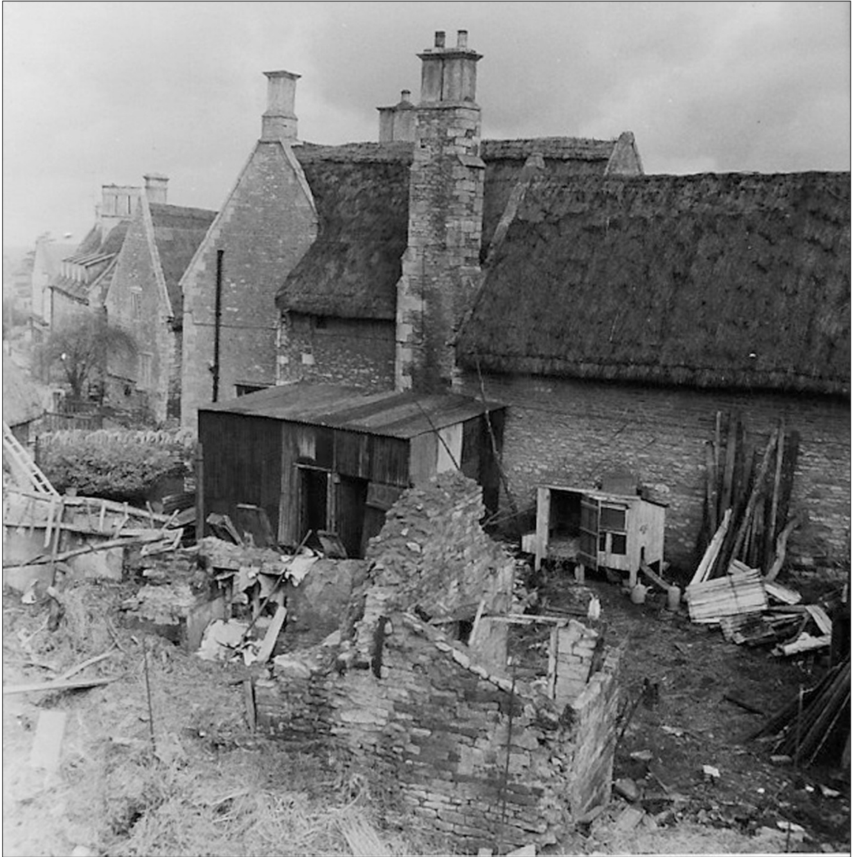
Figure 28. Demolition, 1959. The smaller cottage (Spendlove's cottage). The photograph shows the SE end of the building and attached outhouse with catslide roof
