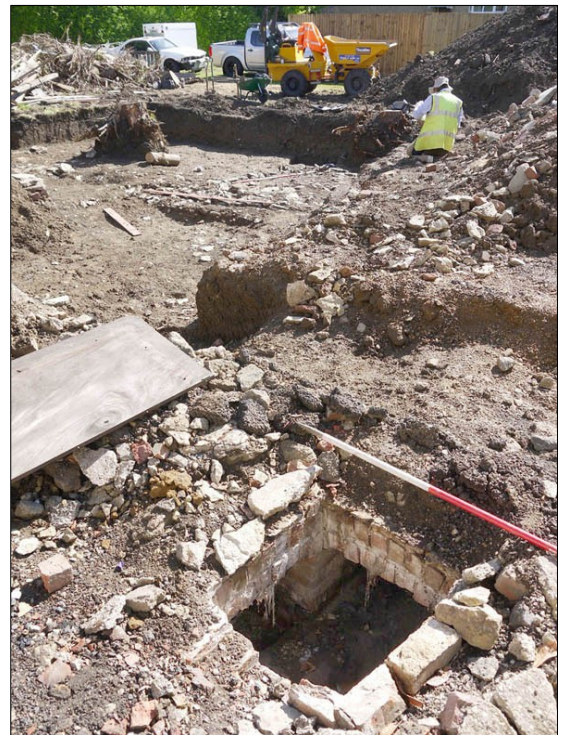
P3. Junction of brick culverts in SW corner of site, Facing NE
