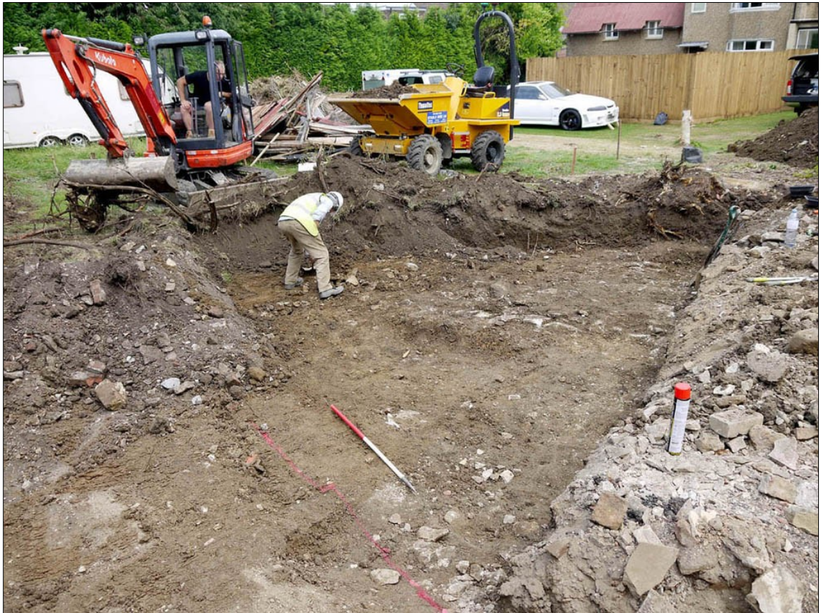
P1. Soil strip in progress, facing NE. No.1A London End in rear ground
