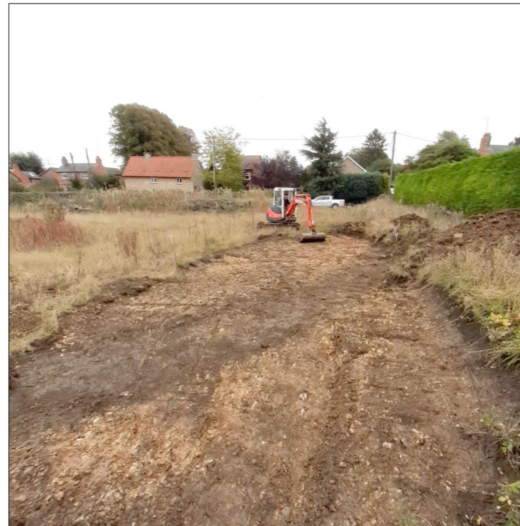
P 2. Soil strip on the W side of house footprint, showing previous levels of ground reduction. Facing S
