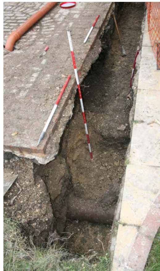
Plate 3. Trench 1: medieval wall foundation (north of pipe, after soak- away removal), facing north
