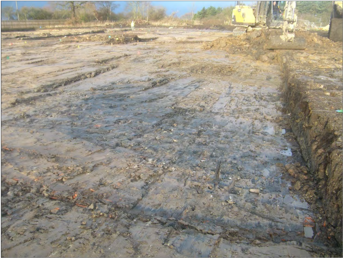
Plate 1: mechanical stripping of the demolition material on the site, revealing natural and archaeological deposits.
