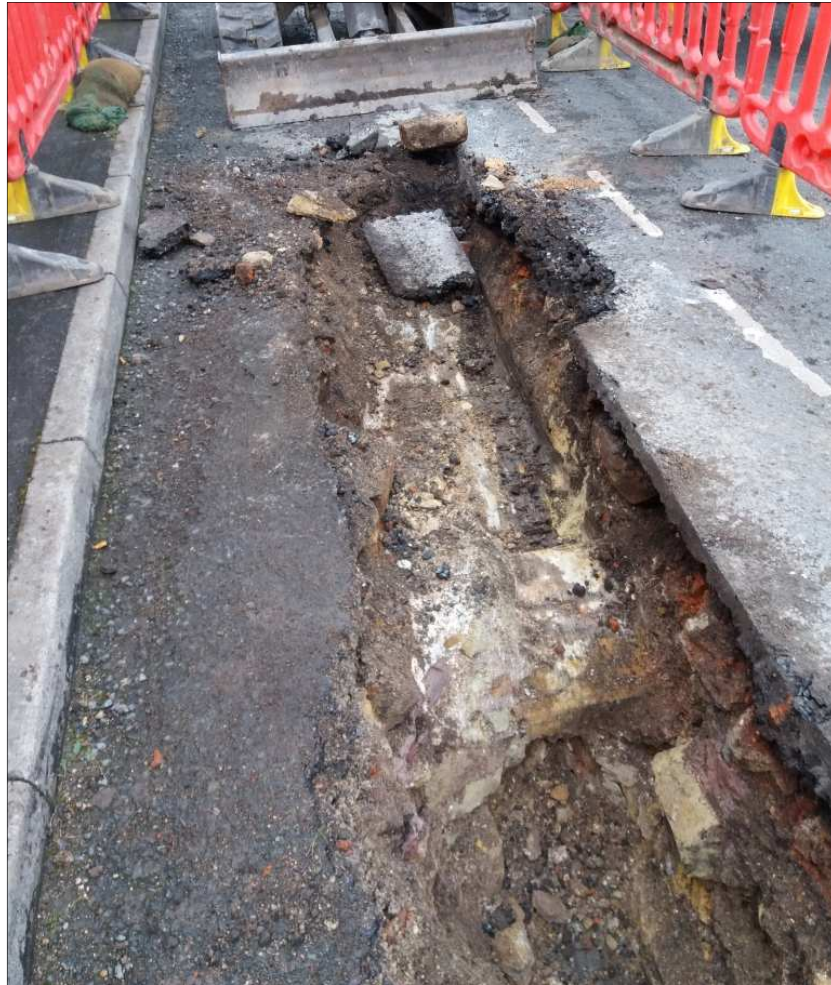
Plate 11: pre-excavation view of Walls 8 (foreground) and 9 (left) forming corner of possible cellar.
