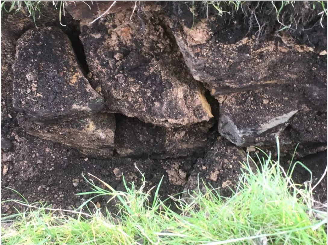
Plate 5: remnant of possible Wall 2 in south side of narrow water main trench. The wall collapsed immediately after this image was taken.
