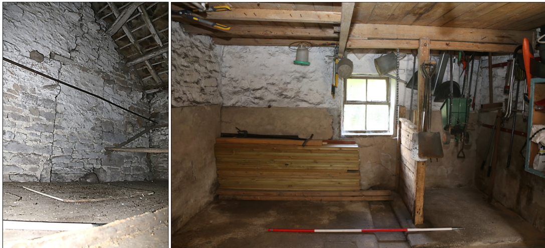
Plates 11 and 12: (left) blocked door (416) leading into room 410 in the upper storey of room 420, and (right) general view of room looking north-west with animal stall (423) and drain (421) visible.
