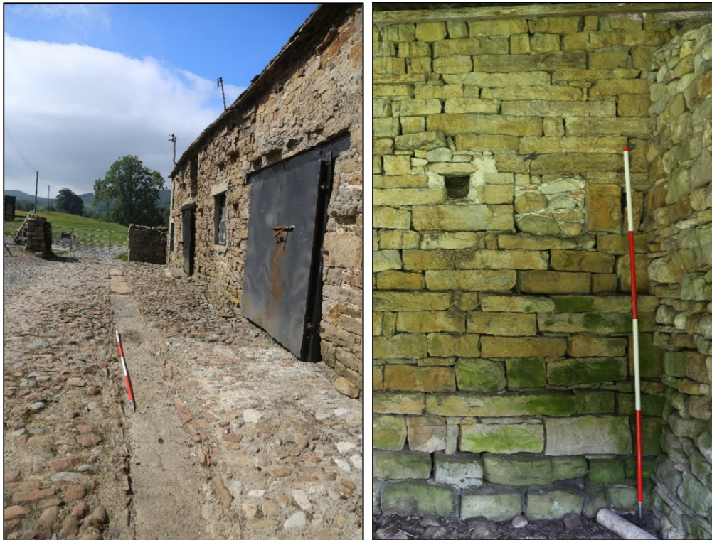
Plates 5 and 6: view of the drain in front of the east-elevation looking south-west and west facing elevation, blocked window (134) at south end with adjacent modern ventilation hole (132).
