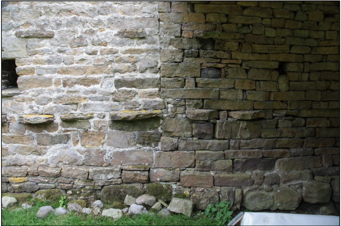
Plate 13: wall joint on the north-west elevation between the barn and the byre. The scar does not extend the full height of the wall but stops above the through-stones that extend into what is now the byre.
