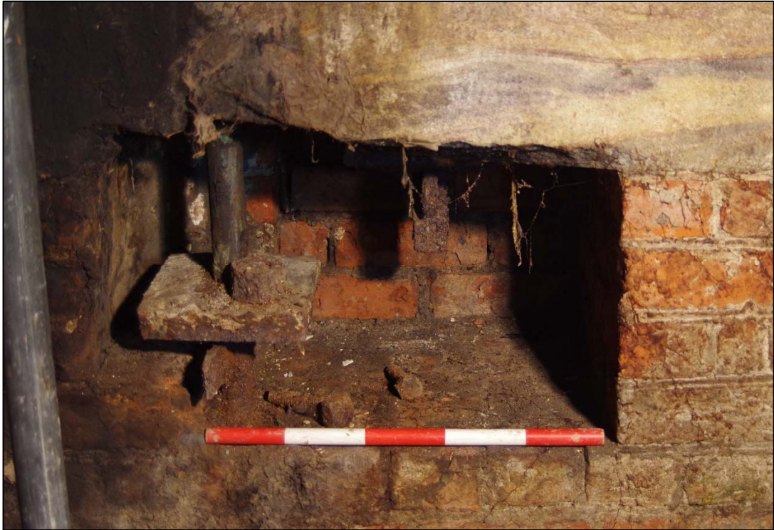
Plate 10: detail of anchoring mechanism 31, niche 36, showing crank handle beneath the square anchor plate.
