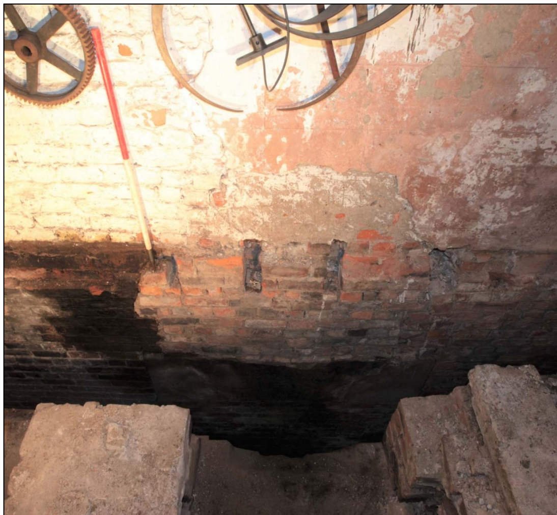
Plate 12: sandstone lintel and bricked up aperture 101 marking the original location of the western flywheel bearing. Iron mount for the eastern bearing (32) is situated in the niche in the foreground.
