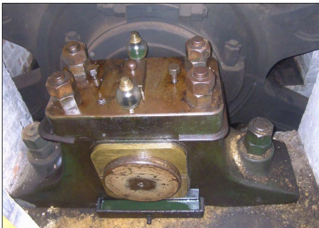
Plate 16: in situ bearing securing the flywheel within the western wall of the flywheel pit in the Edwardian beam hall.
