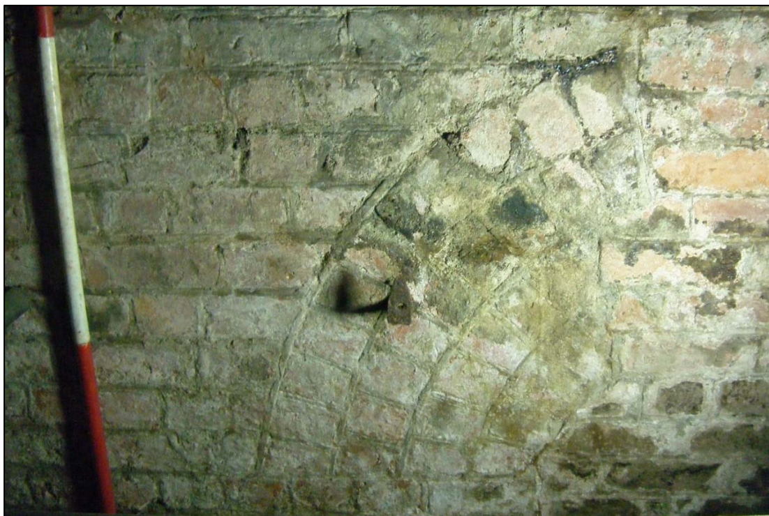
Plate 7: remains of bricked up arch 21 in the south wall of the pumping chamber.
