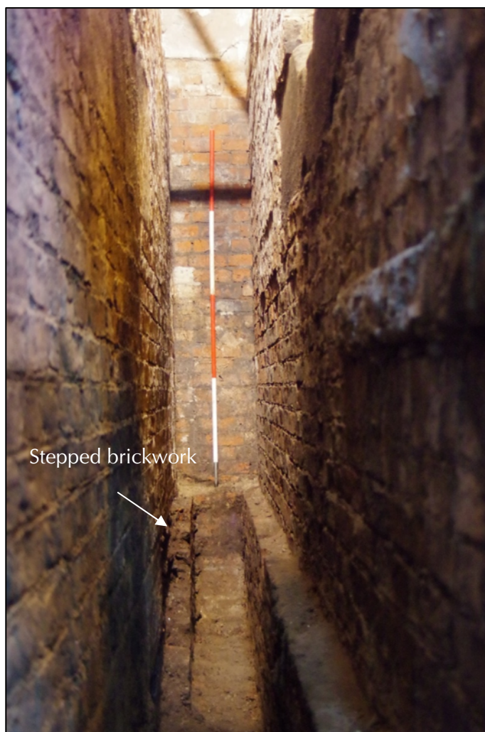
Plate 11: interior of flywheel pit 100, looking north, showing internal brick ledge and stepping within the east-facing elevation to accommodate the profile of the flywheel.
