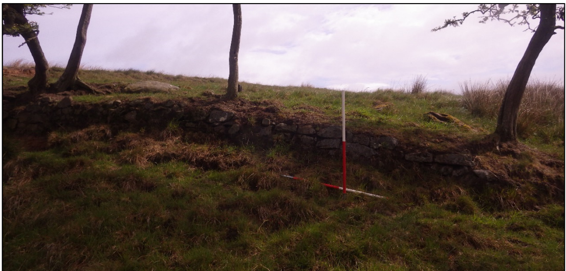
Plate 4: boundary wall of 010 looking east. The plantation is positioned above a gully which separates it from 011.
