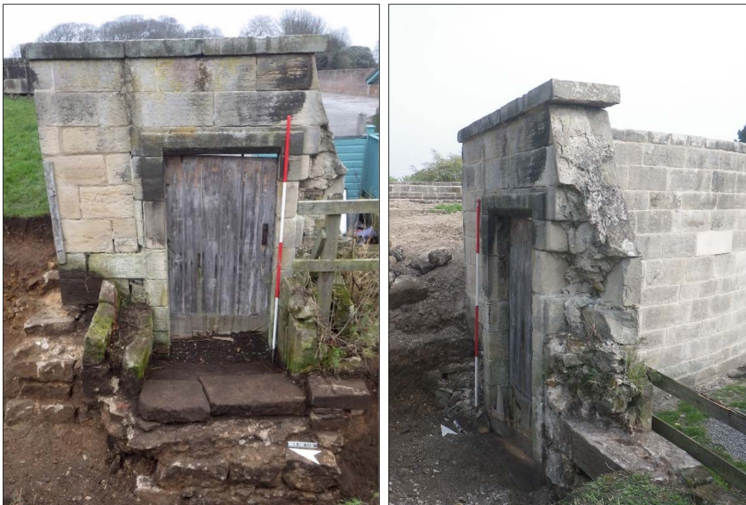
Plates 7, 8: (left) gateway 23 with step 31 and retaining wall 25 during primary excavation; (right) full extent of gateway exposed prior to renovation.
