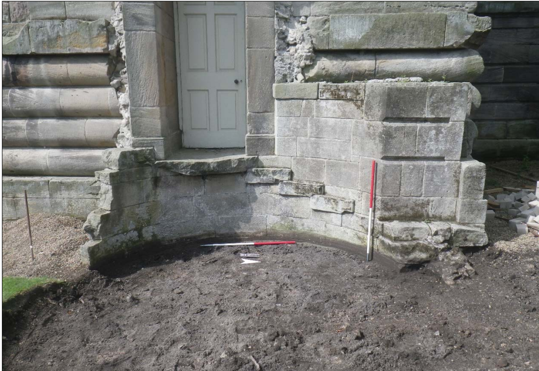
Plate 24: removal of turf in the stairwell of the south-east range prior to installation of gravelled area.
