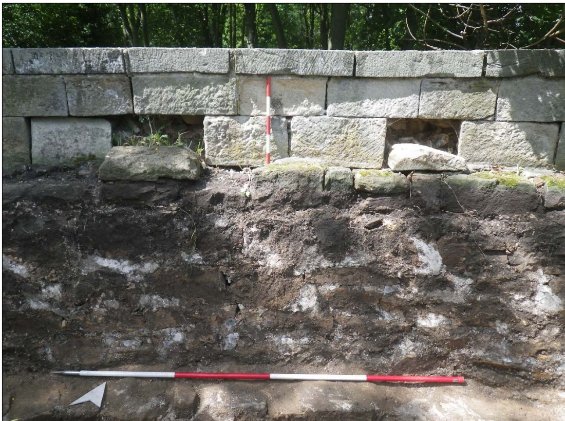
Plate 10: interior face of the north-west bastion after hand clearance, with weather damage to the ashlar courses and foundation plinth in the base of the trench.
