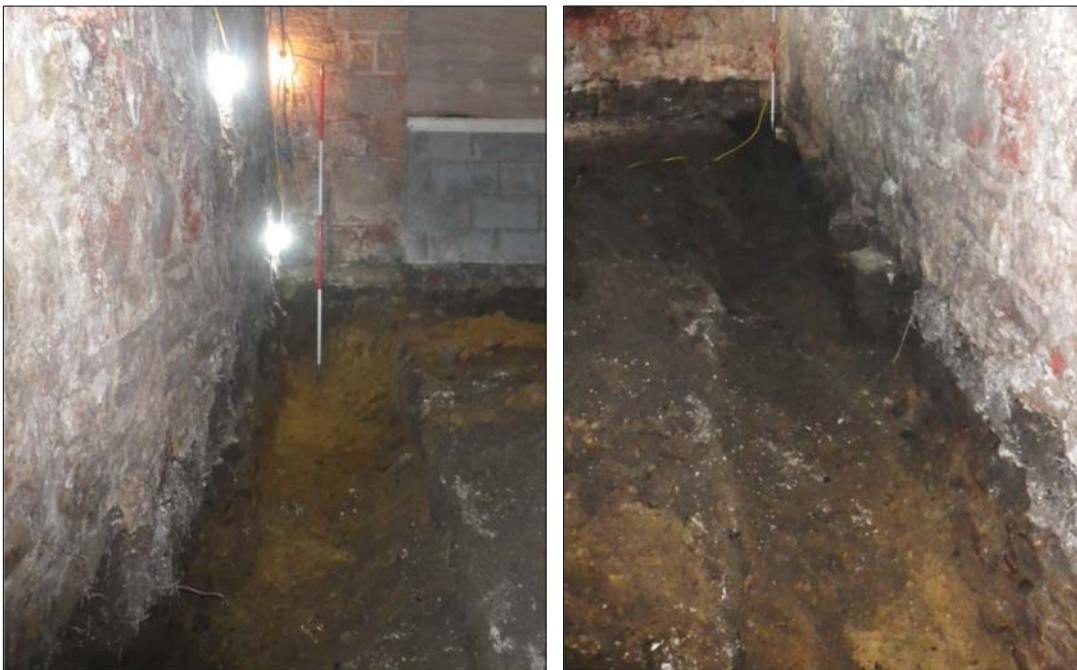
Plates 6-7: service trench along the south wall of the cartshed; looking west (left) and east (right).
