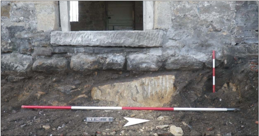
Plate 17: Foundation course 45 to the brewhouse at the northwest corner of the building lying directly on the natural bedrock.
