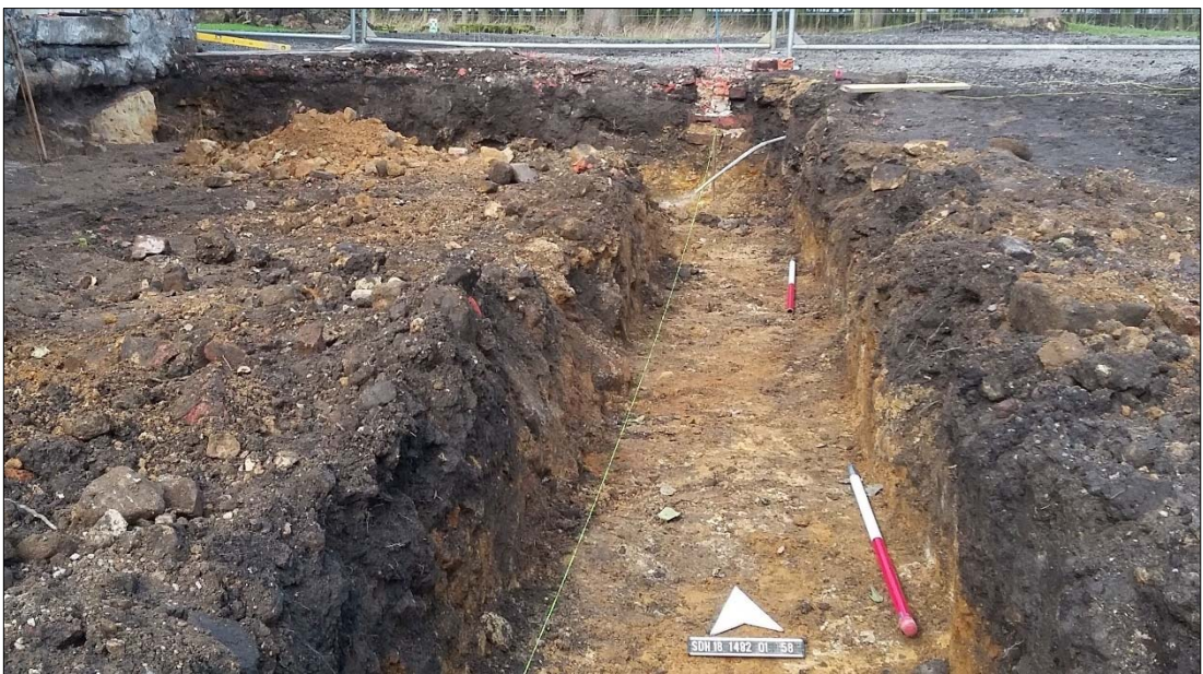
Plate 18: foundation trench for the brewhouse café development with modern deposits over weathered natural sandstone.
