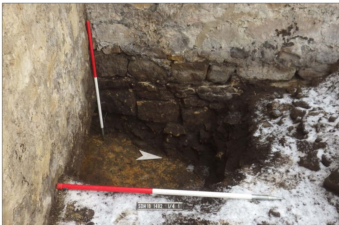
Plate 16: depth of foundations and gradient of natural clay 30 at the south-east corner of the brewhouse.
