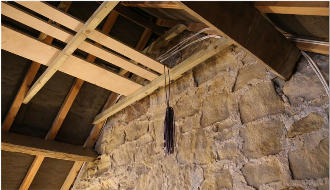
Plate 24: north-facing side of the partition wall apex, showing differential wear of the stonework.
