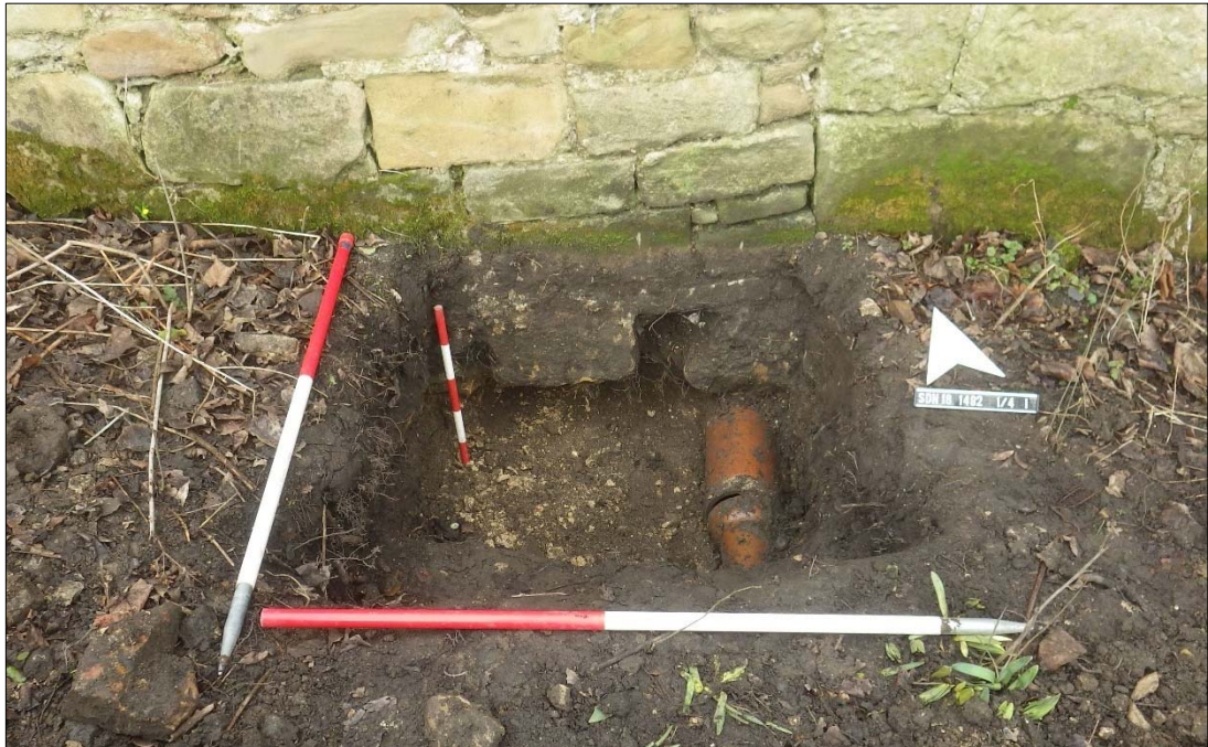
Plate 14: ceramic drain beneath boundary wall 78 in the underpinning trench at the south-west corner of the brewhouse (on the right).
