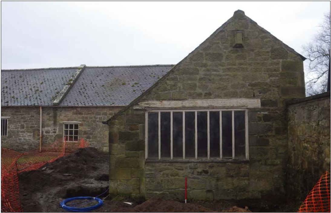
Plate 1: blocked cart-entry in west-facing gable elevation of the cartshed.
