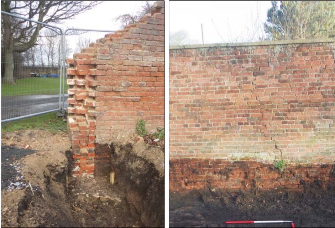
Plates 40, 41: (left) cross section through the wall exposed during dismantling, and (right) sample section of brickwork with concrete capping.
