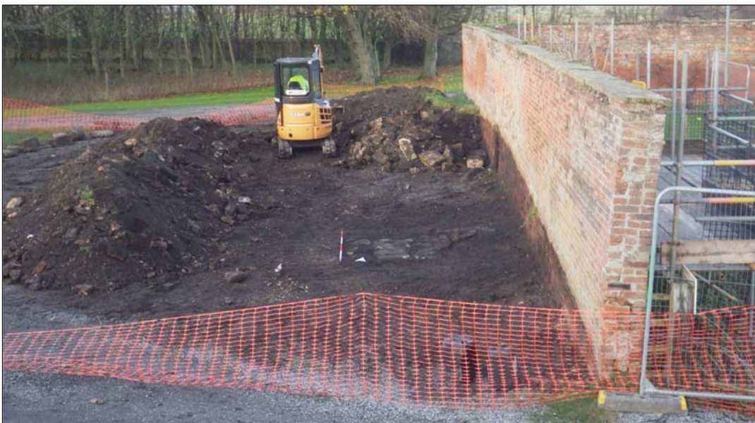
Plate 39: north section of the west wall of the walled garden during clearance of the turfed mound.
