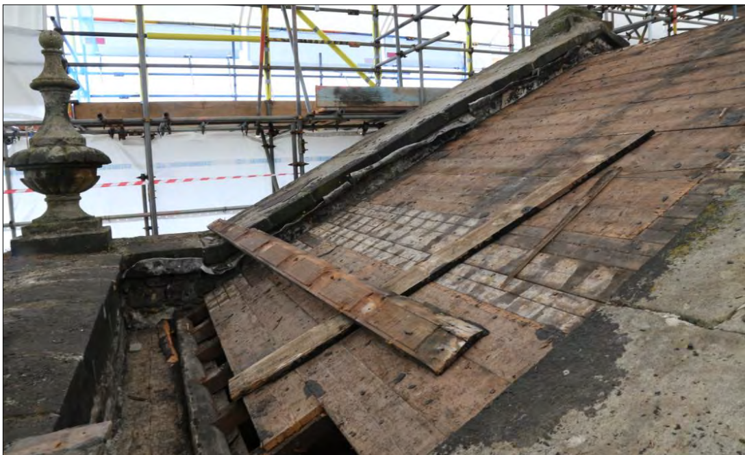
Plate 2: evidence of lead flashing surviving beneath the coping of the pediment chamber roof (130).
