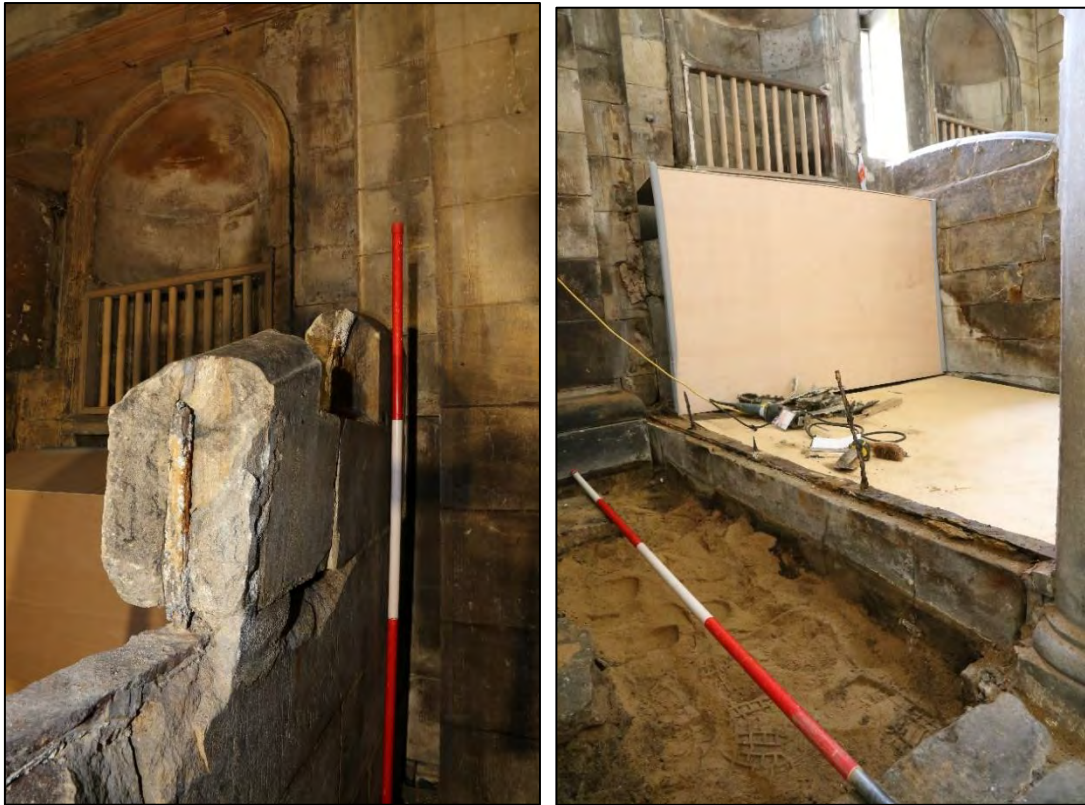
Plates 44, 135: (left) iron strap found across the upper part of the divider S13 with two of the three vertical iron dowels emerging upwards from the tie; (right) the lower strap near the base of divider S10.
