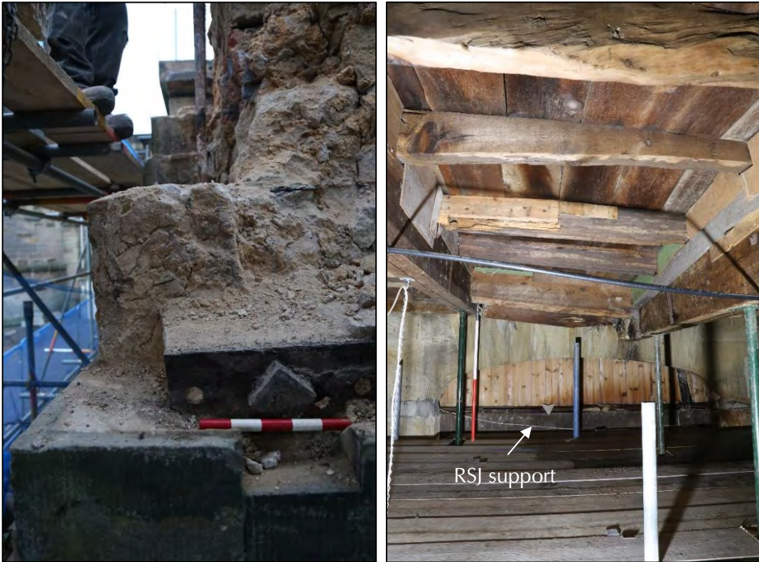
Plates 120, 121: (left) iron bracket tied in the masonry; (right) view of the inside of the carriage house looking south.
