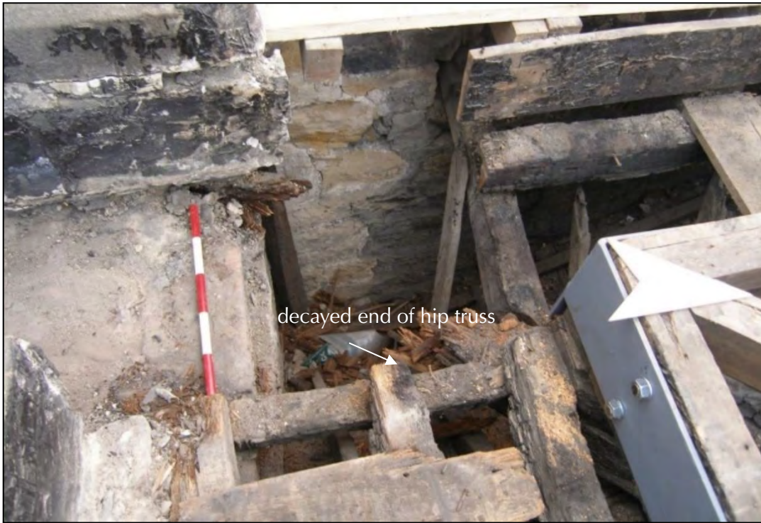
Plate 32: view of decayed hip truss in the south-west corner of the central roof. The timber is located at the junction of three gutters, draining south past the wall.
