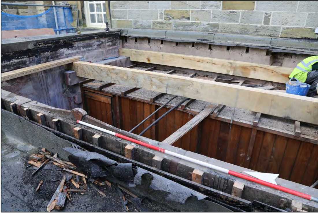
Plate 115: east side of truss 700 with the purlin holes visible in the masonry to the rear.
