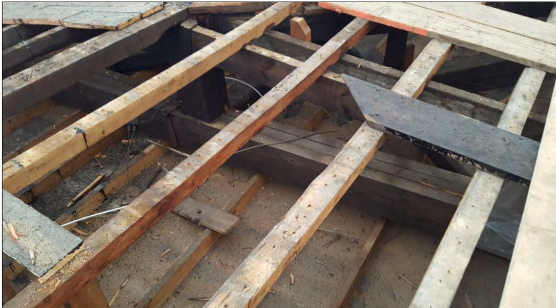
Plate 12: section of replacement roof structure in the north range – purlins truss and ceiling are all modern.
