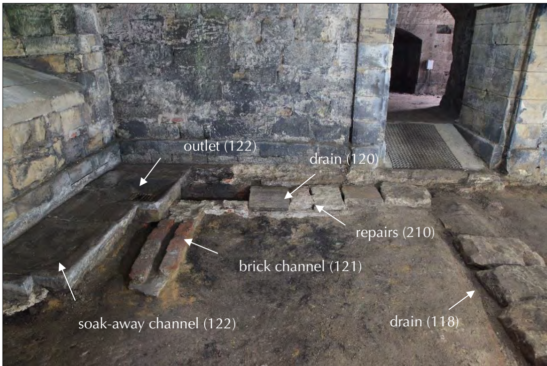
Plate 88: drainage area 122 and brick drain 121, with a phase of repair and alteration (210) to drains 118 and 120 visible along the north wall.
