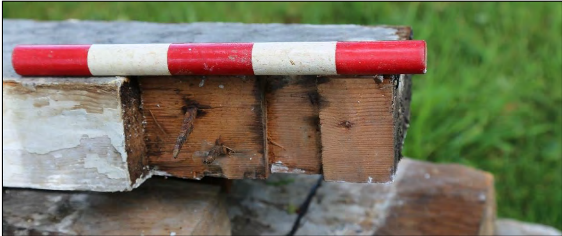
Plate 117: purlin cut to accommodate trusses with a deeper cut for the internal iron clamp.
