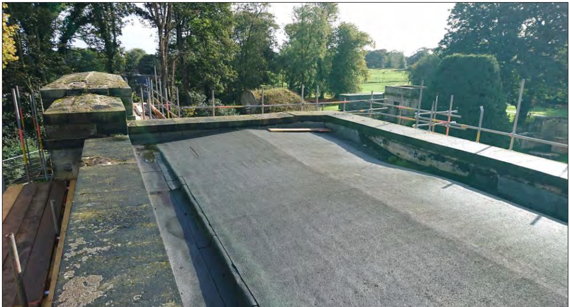
Plate 112: east roof of the Carriage House looking east, showing the shallow-pitched gable hidden by the parapet, and two flanking drainage channels. Image reproduced by kind permission of Mosedale Gillatt Architects.
