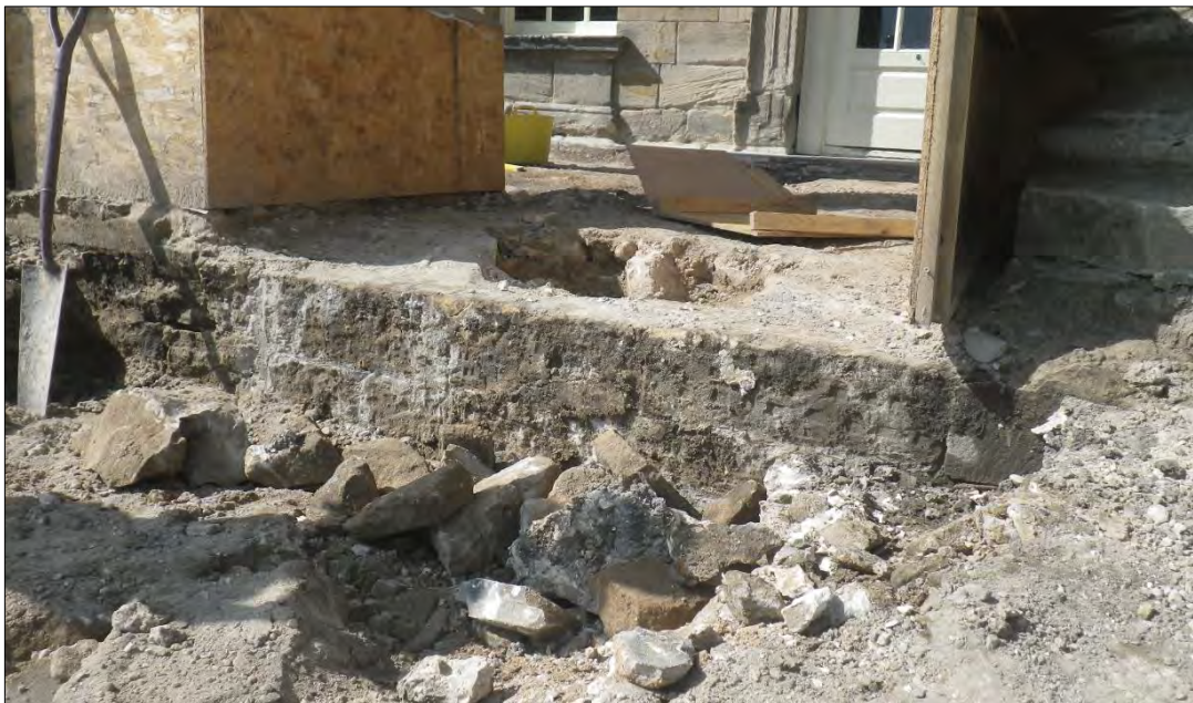
Plate 105: south face of the original upper landing riser exposed during excavation with rubble from the infill visible in the foreground.
