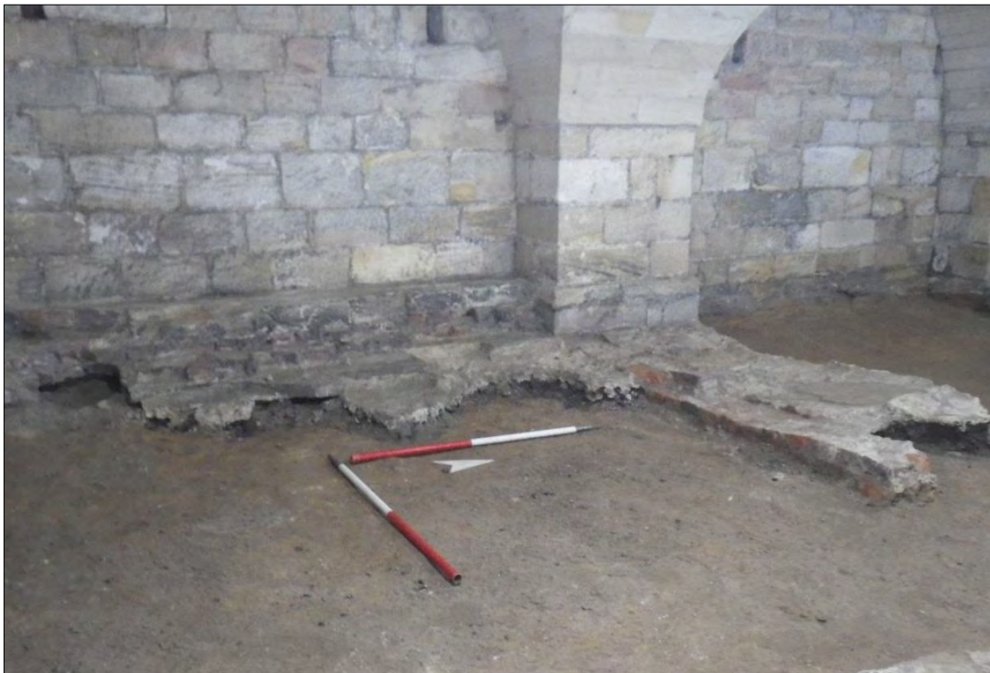
Plate 84: wall 127 with mortared floor surface 128 to the south, overlain by raised area 129 against the west wall.
