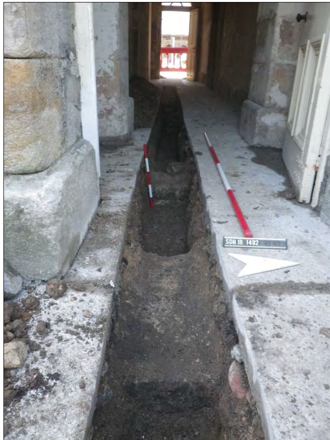
Plate 128: wall foundations 66 beneath the passage between the central stables and south block.
