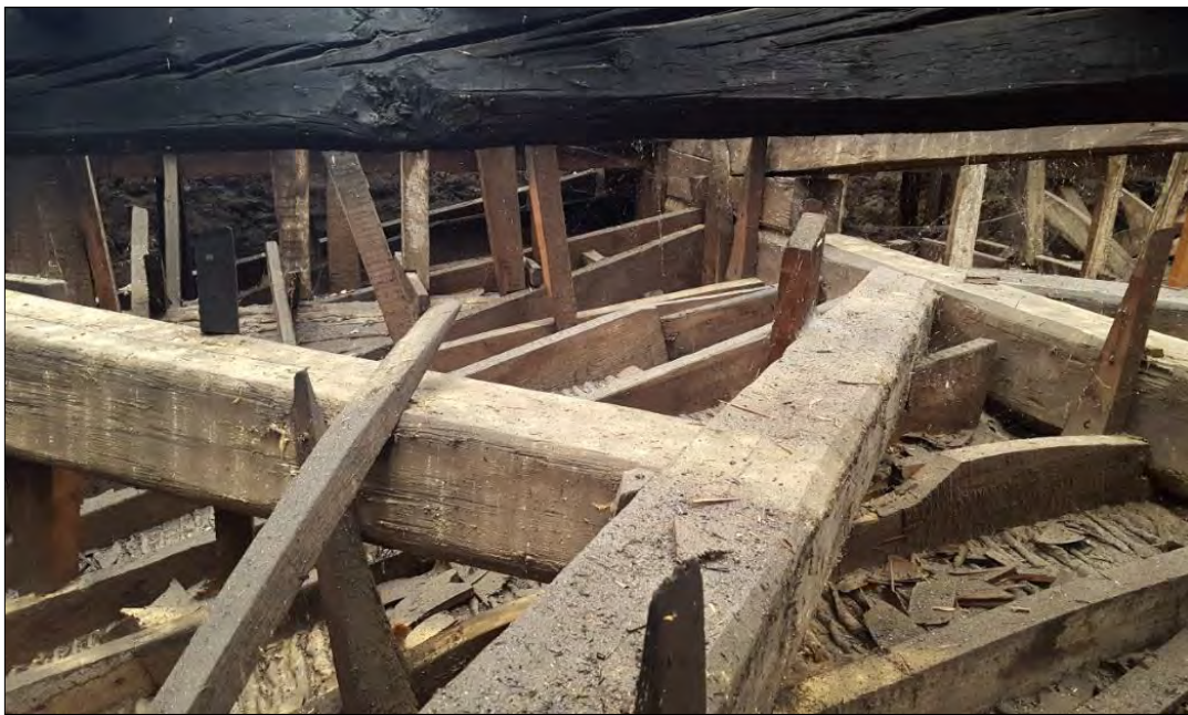
Plate 25: section of the south-west lower roof structure showing a principal truss, main joists, vaulting joists and ceiling struts. There is clear evidence of charring on the hip truss, just visible at the top of the picture
