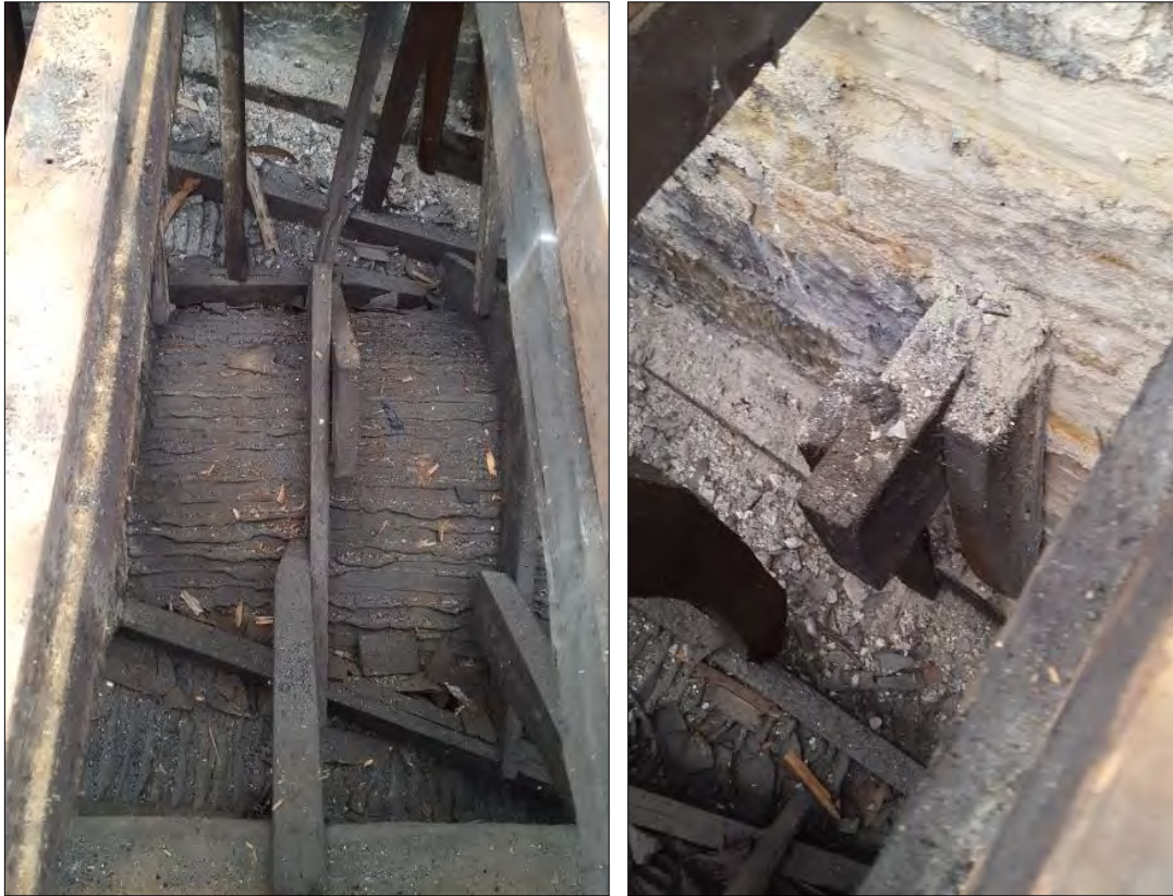
Plates 28, 29: detail of vaulted ceiling structure beneath central range (left) and (right) one of the vertical timbers and connecting floor joists tying the pediment chamber to the main roof structure.
