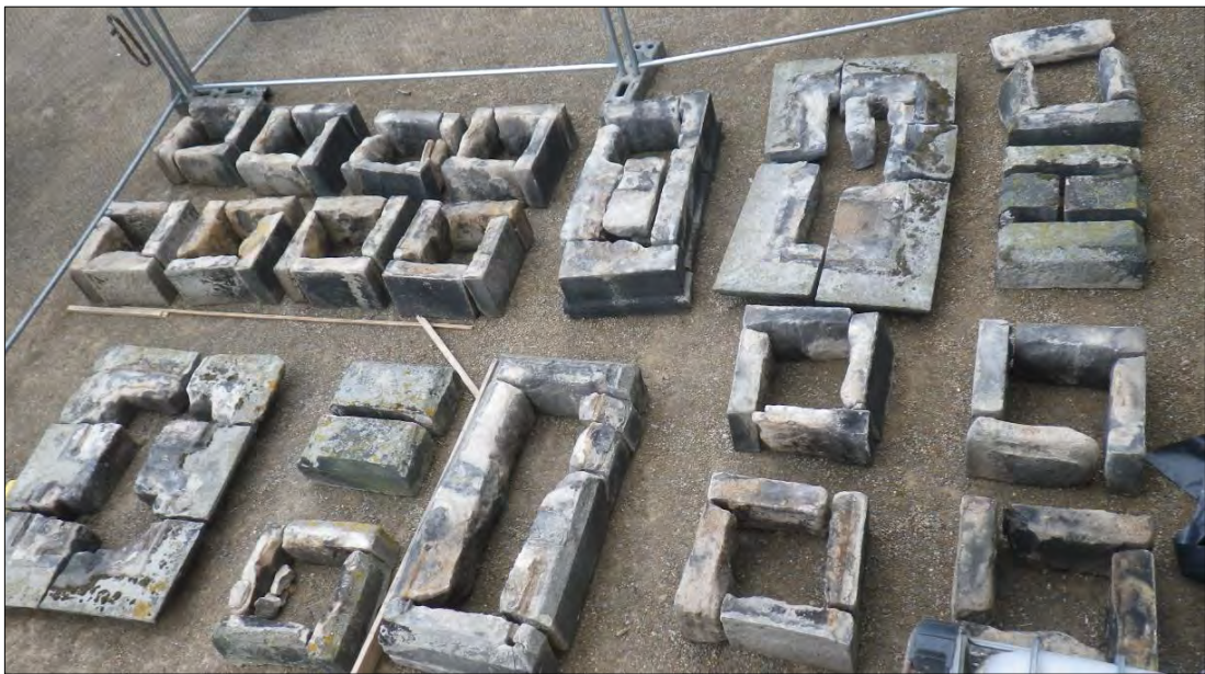
Plate 7: chimney copings removed and awaiting repair and reinstatement.
