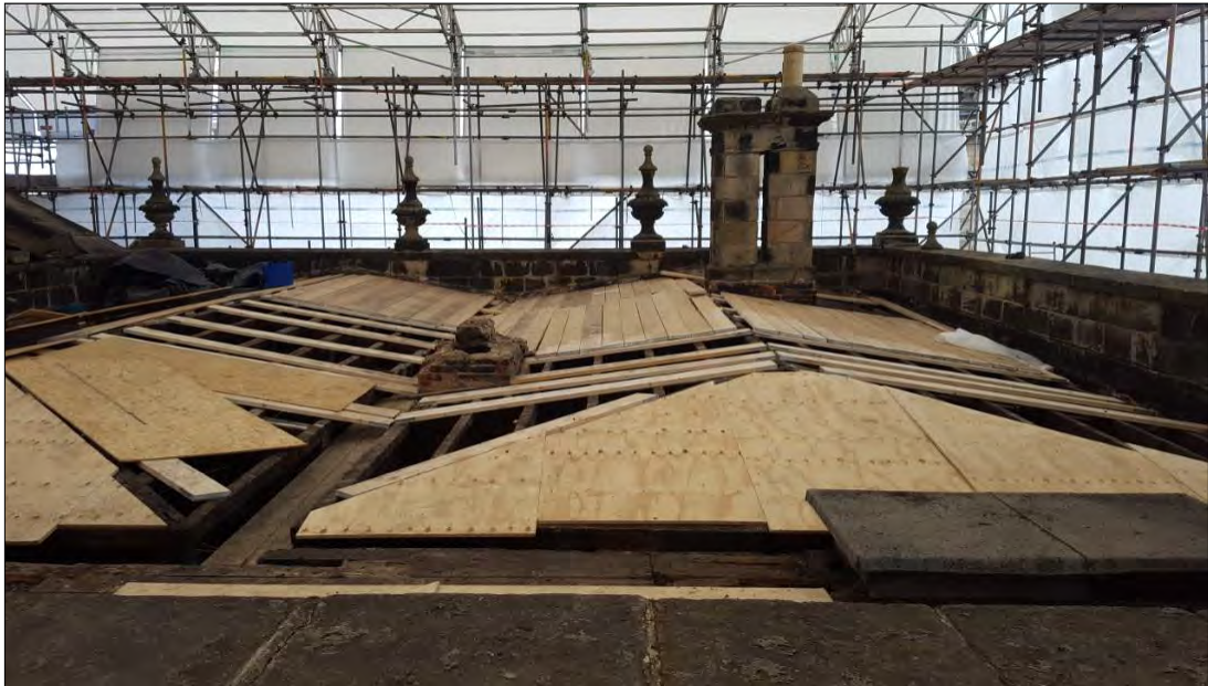
Plate 4: south range looking east towards the south-east stack (108). The remains of the of the central stack (107) are also visible in the valley between the two hipped sections.
