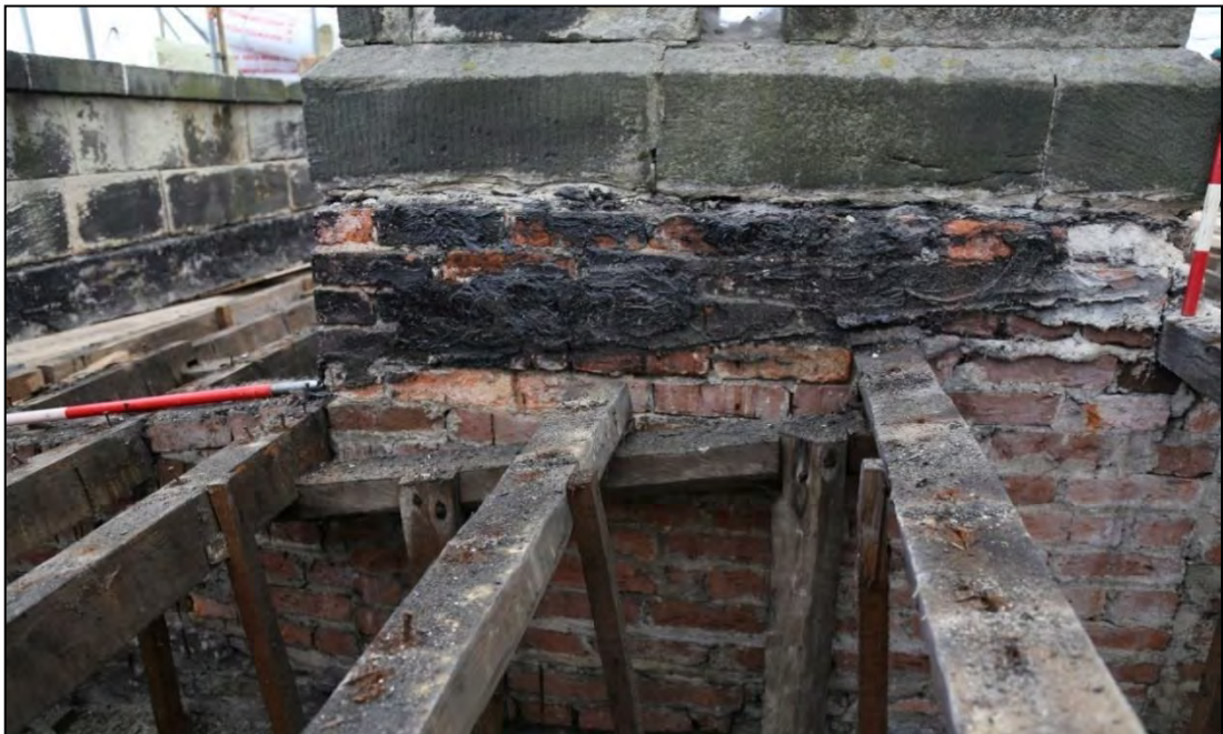
Plate 41: chimney 108 and raised section of the cross wall which supported the shallow pitched roof, replacing the former hip truss.
