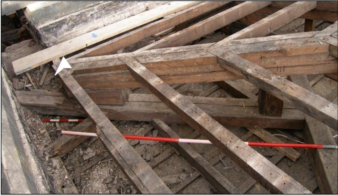
Plate 35: hip truss 201 in the north-west corner of roof 143. This originally spanned gutter 146 to tie into the wall but had been cut. The gutter passed under the stone wall at the top of the photo.
