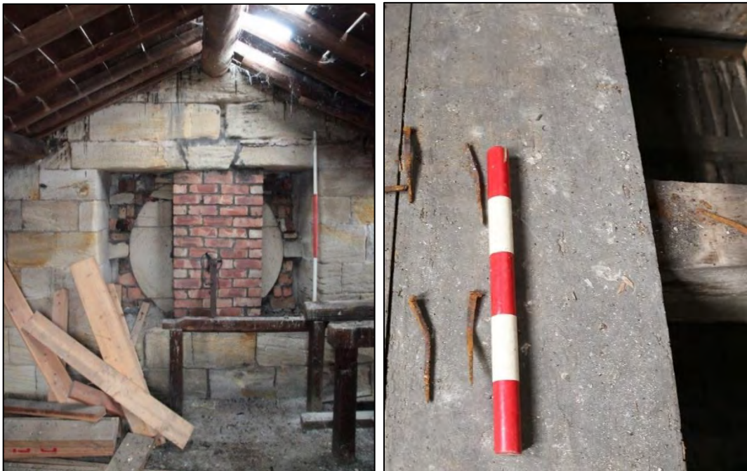
Plates 53, 54: (left) remains of clock gantry inside the pediment chamber; (right) nails removed from floorboards during repairs.
