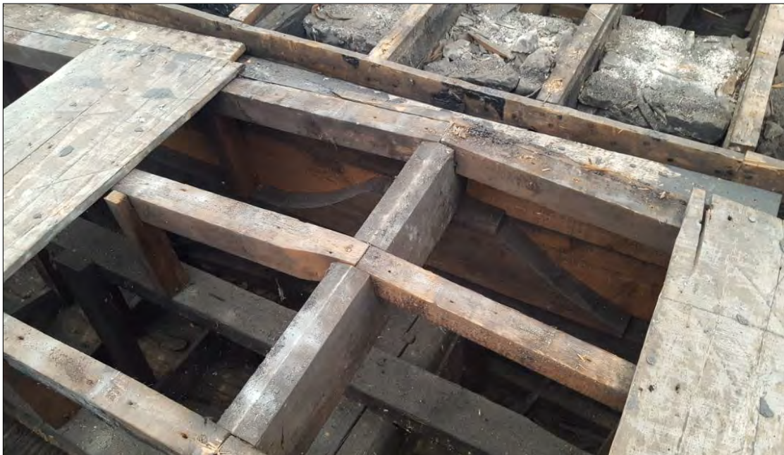
Plate 21: bracing associated with the inserted wooden gable. There are clearly three phases of development visible at this end of the roof.
