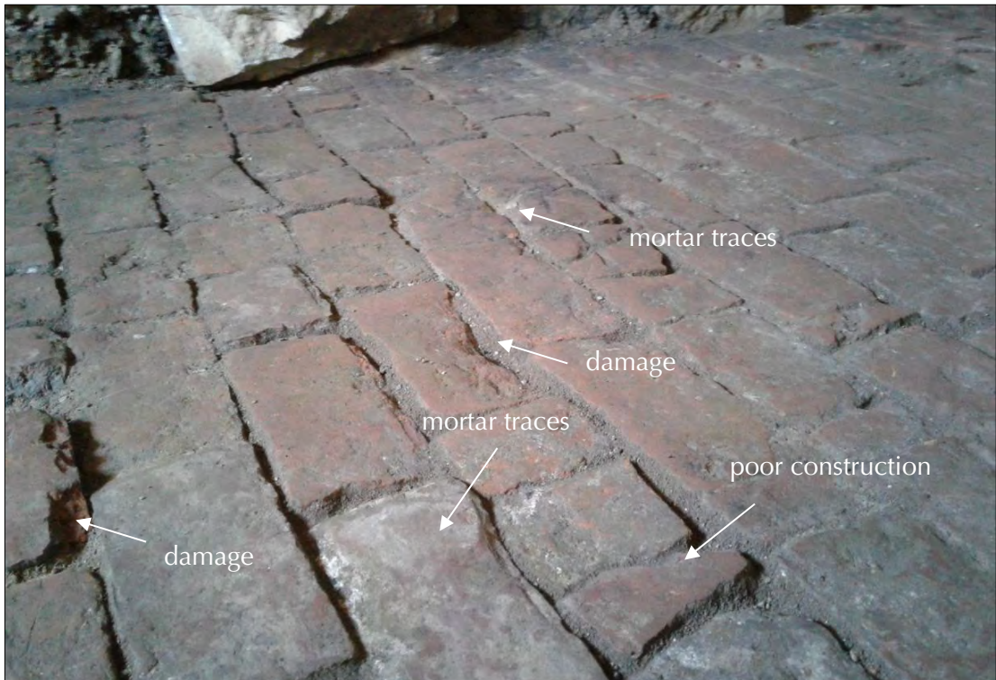
Plate 143: section of brick surface 133 in room B10 showing examples of mortar traces, uneven damage patterns and poor construction.
