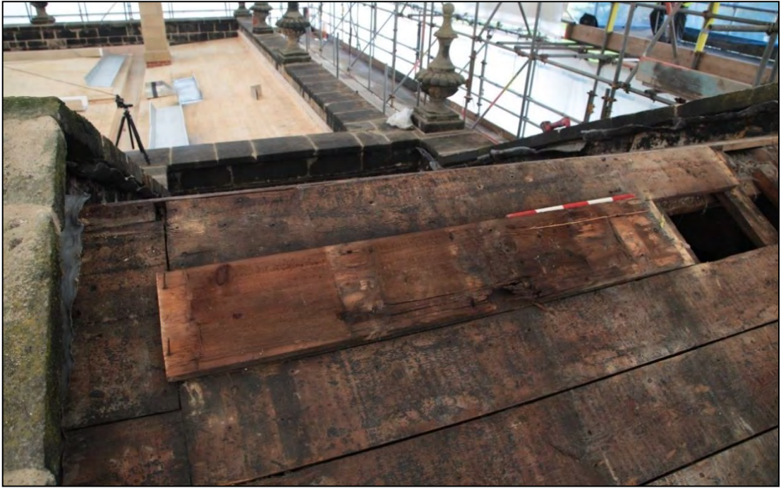
Plate 43: underside of one of the sarking boards removed from the pediment chamber roof. The groove formed to hold the rafters can be seen evenly spaced along the board.
