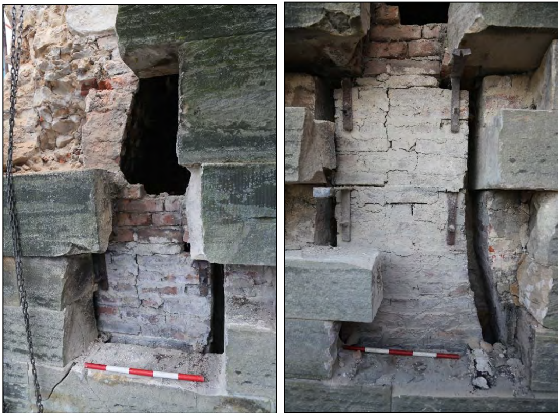
Plates 122, 123: (left) cavity visible at the top of the chimney; (right) the chimney tapers out near the base of the wall and was tied to the masonry through iron brackets.
