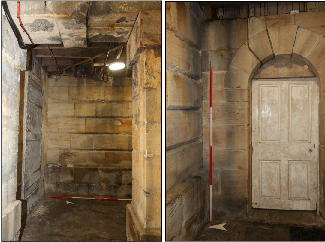
Plates 57, 58: (left) looking east down the east kitchen passage towards the end vestibule. The flat arch with dropped keystone is visible in the foreground, and wooden plank door entrance into the arcade can just be seen to the left of the picture; (right) door into the west staircase of the Central Hall.
