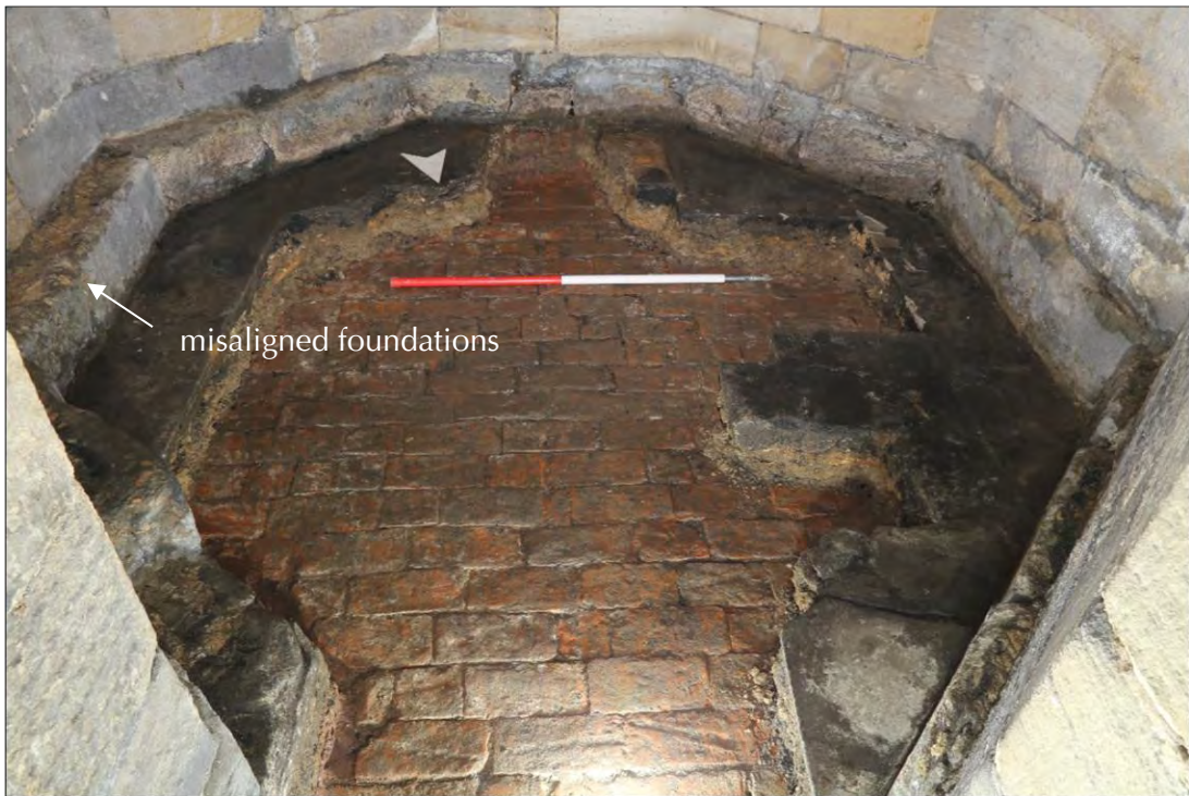
Plate 100: foundation course 201 and remains of floor make-up within the south-west turret, with groundwater seepage in brick surface 133 at the far wall.
