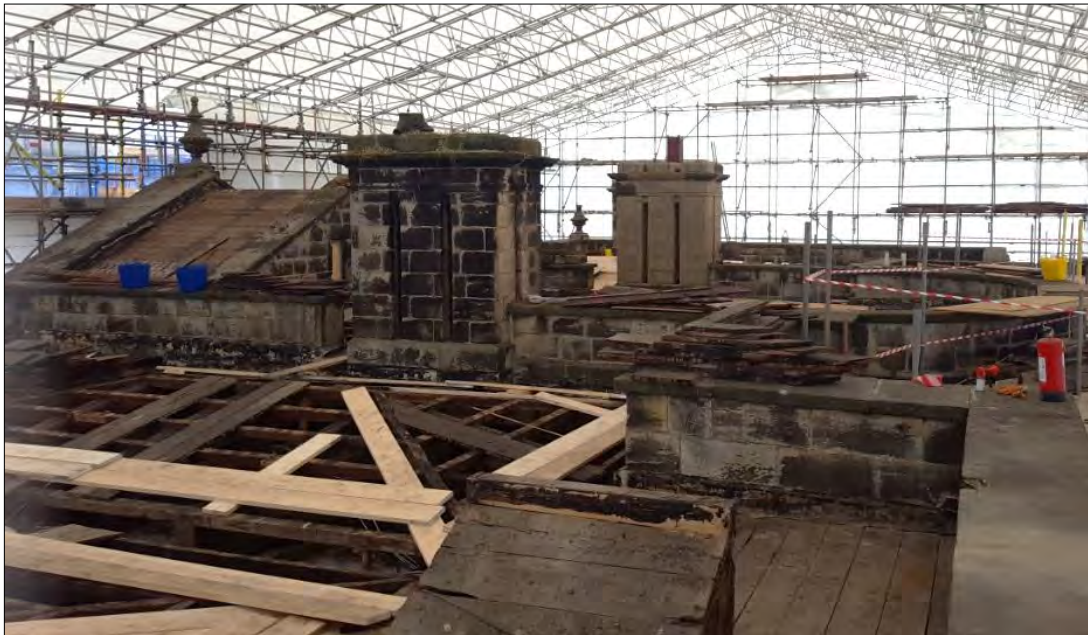
Plate 3: looking south-east across the west roof showing both main chimney stacks and the pediment chamber (130). The north stack (102) is clearly older than the south stack (103), the latter being replaced in the late 19th century.
