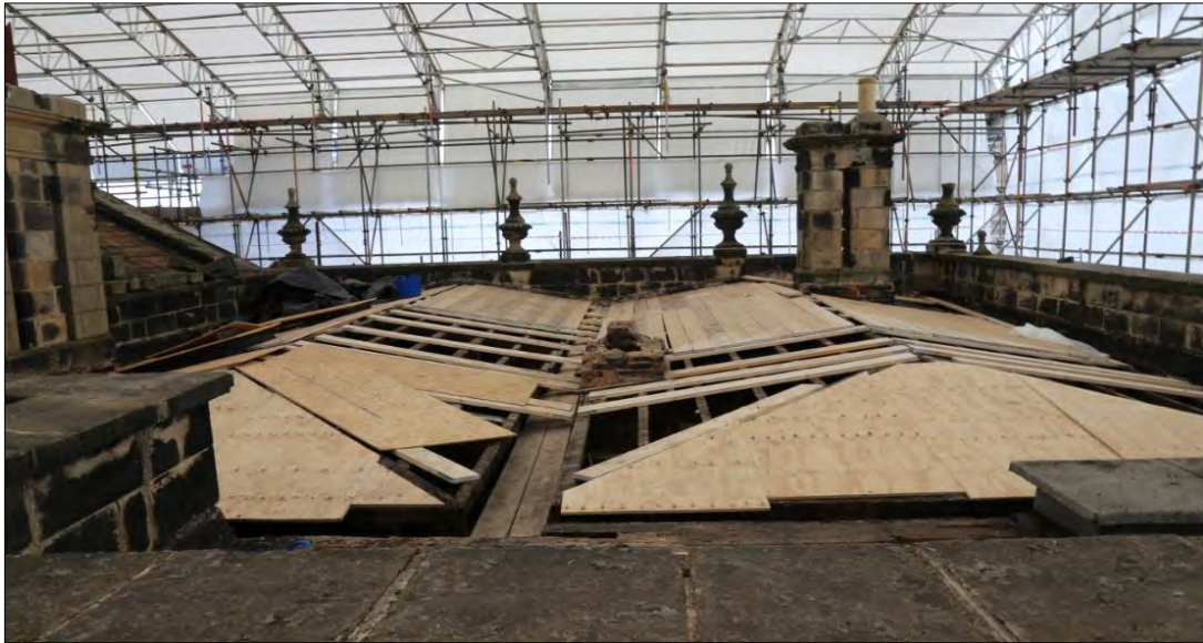
Plate 31: south range looking north, roof 143 to the north (left) and 144 to the south (right).
