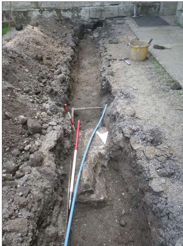
Plate 129: wall foundation 64 in the electrical ducting trench with the south wall of yard in the background.
