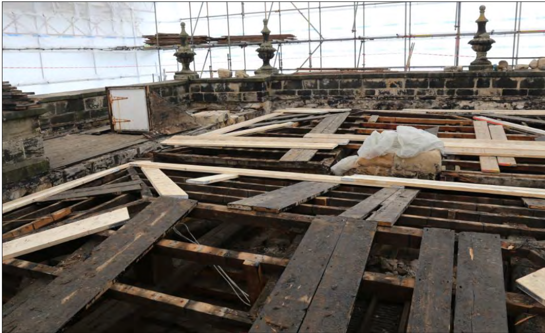
Plate 14: looking north-west across the western end of the north range showing the projecting bay (114) and the roof access hatch (117).
