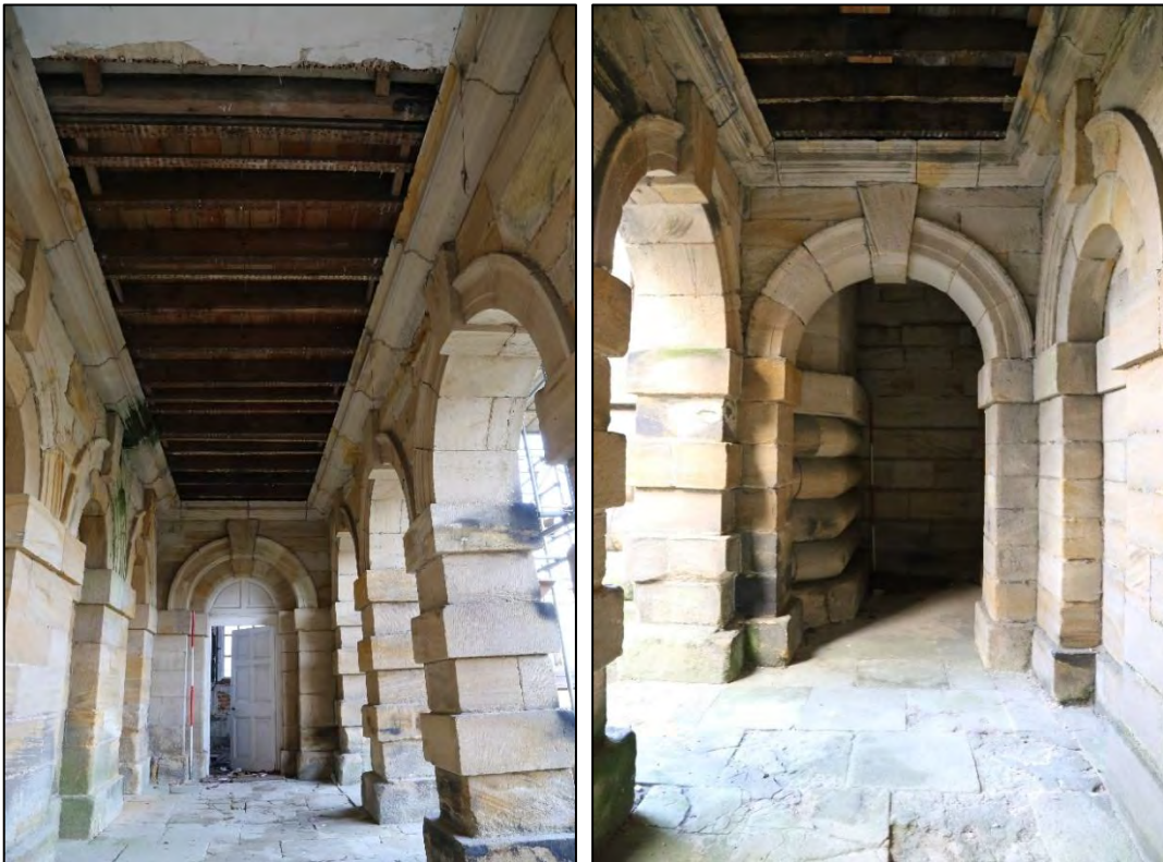
Plates 46,47: (left) door into the north-west pavilion marking the end of the northern end of the arcade, and (right) the east end of the arcade terminates in a round vestibule with the door to the kitchen passage just out of view on the south (right) wall.
