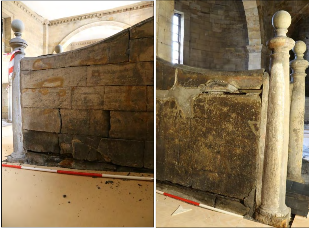
Plates 537, 138: (left) the masonry of S10 was cut flush with the stone divider; and (right) timber batten in S13 filling the gap between the post and masonry.
