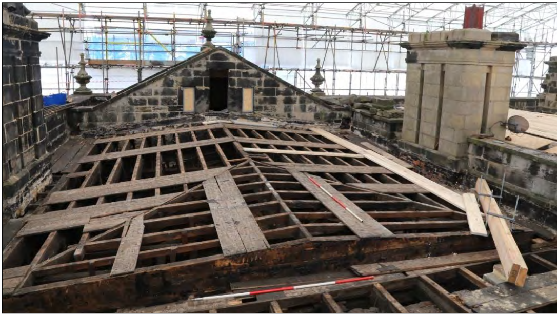
Plate 18: looking south-east across the central roof (122) showing the reconfiguration of the west end.
