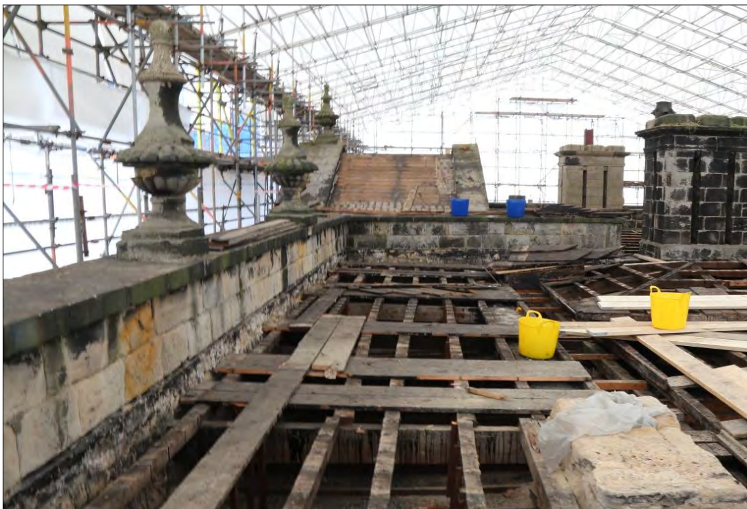
Plate 13: flat section of roof (113) running along the front of the north range, looking south towards the pediment chamber. Note the base of the dismantled chimney stack (105) in the bottom right corner of the photograph.
