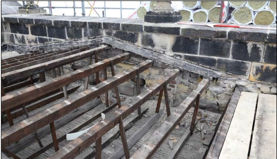
Plate 40: east end of the roof 143 looking east. The purlins can be seen tied directly into the east wall beneath the line of the inset gable (marked by a line of lead flashing).
