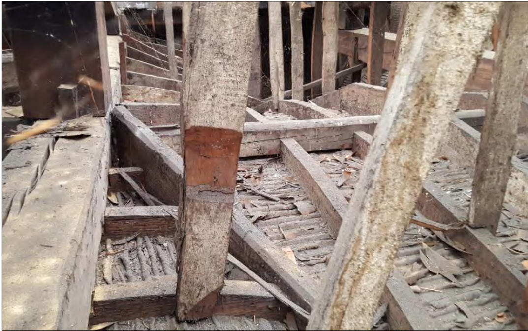
Plate 26: detail of lower roof and ceiling structure at the west end of the central range. The strut at the centre of the picture has been either reused or was intended to be in an alternative position. It has been shaped to accept a cross timber.
