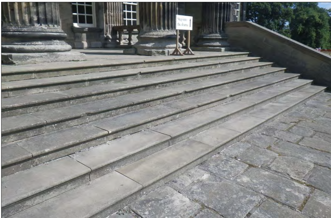
Plate 103: pre-intervention survey of the portico steps showing cast-concrete pavers of the upper flight and flagstones of the intermediate half landing.
