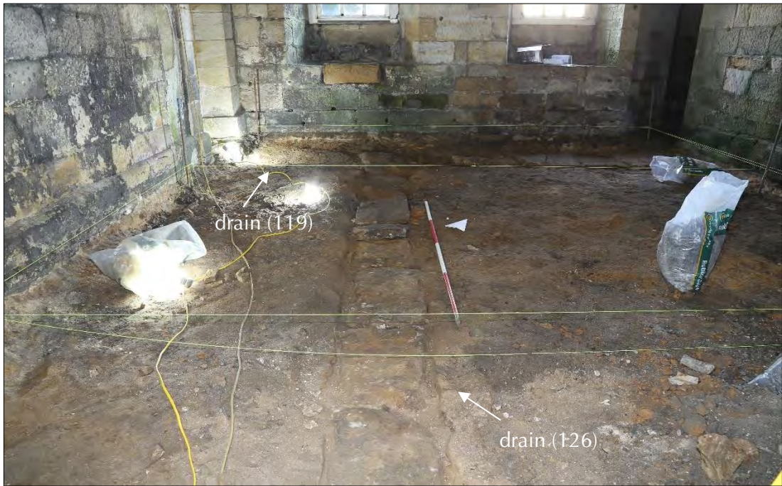
Plate 90: B04 during ground reduction, with drain 126 running north-west and drain 119 on the north side of the room.
