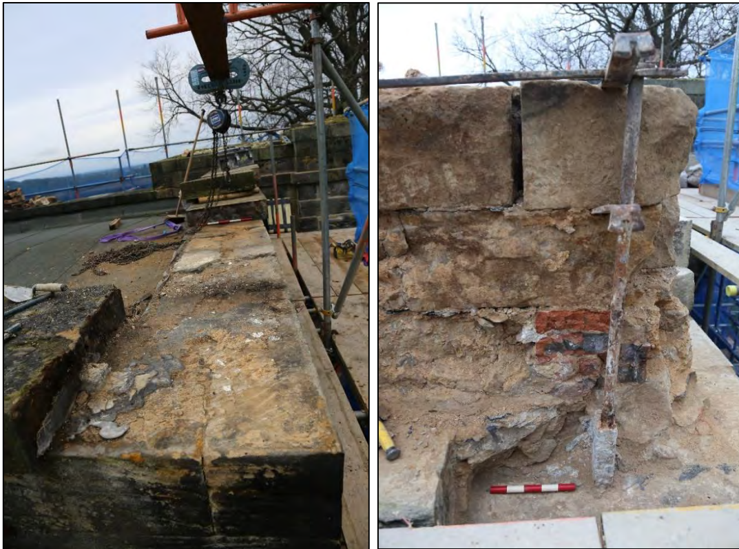
Plates 118, 119: (left) looking north, the removal of the coping stones along the eastern side of the building; (right) iron beam, pin, and brackets revealed behind masonry.
