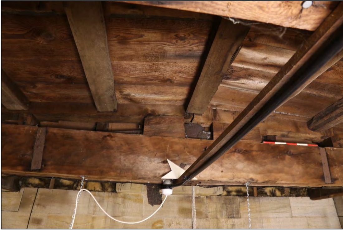
Plate 114: truss 600; looking west toward the cross wall and chimney. The iron brackets are visible on either end of the tie beam.
