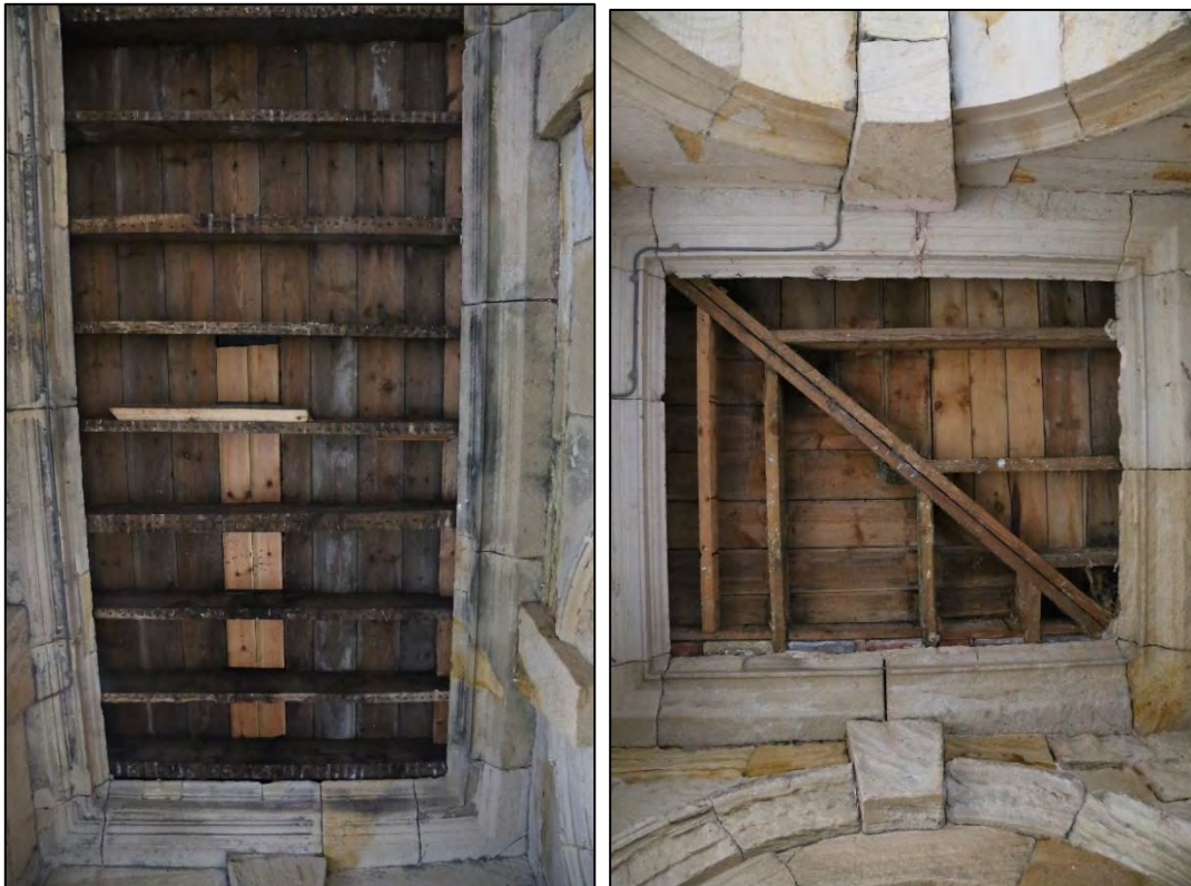
Plates 50, 51: (left) ceiling above the west arcade connecting with the Central Hall. A repair is visible on one of the joists; (right) the junction between the west arcade and the south arcade.
