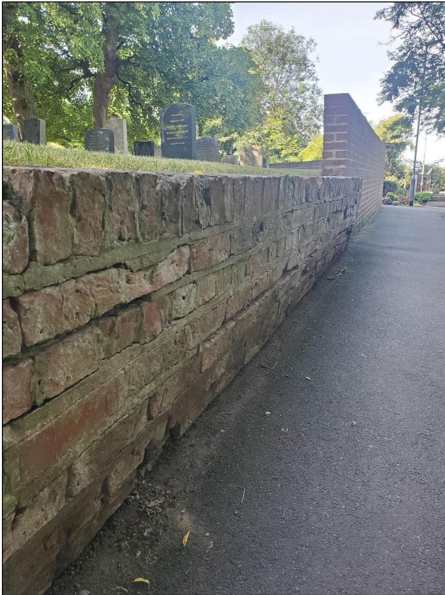
Plate 1: Bowing of the western boundary wall, looking south towards the 2007 reconstruction.
