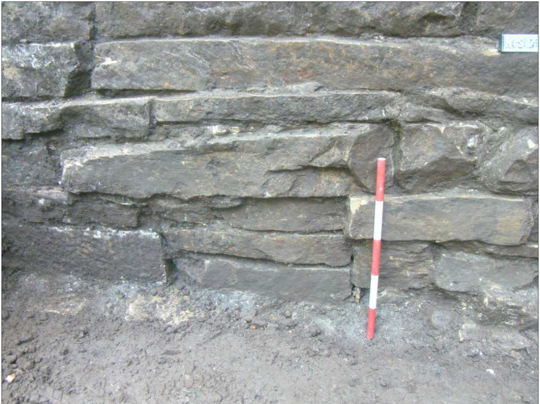
Plate 2. Blocked ventilation hole within possible medieval foundations 004
