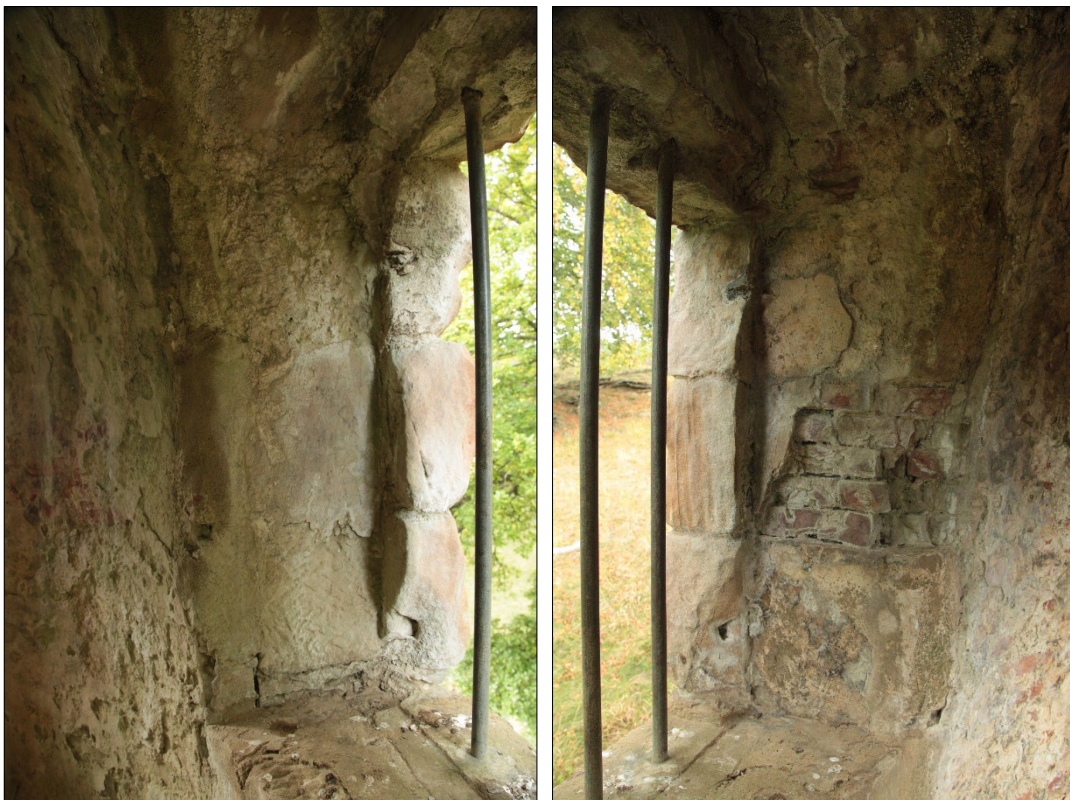
Plate 34: detail showing the north-facing window recess, west side (left) east side (right).
