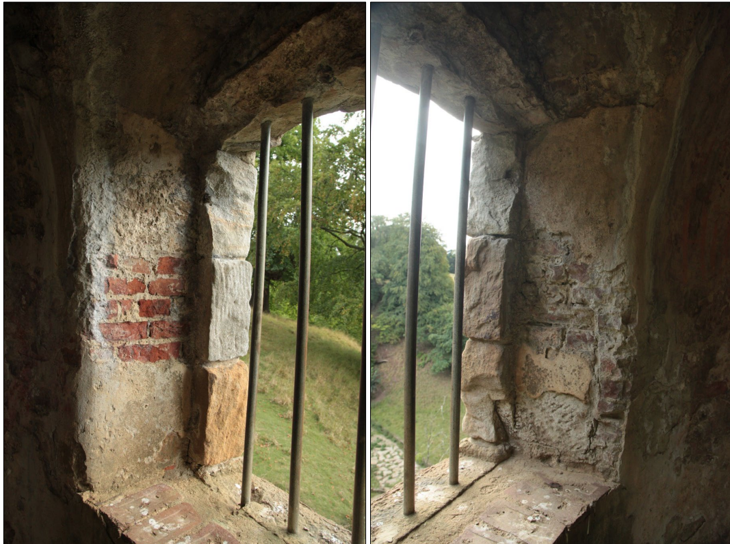
Plate 29: detail showing the south-facing window recess, east side (left), and west side (right).
