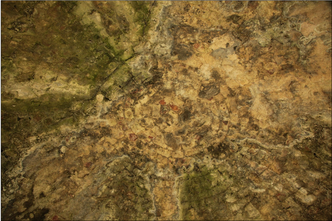
Plate 28: detail showing the header bond used to create the top of the dome.
