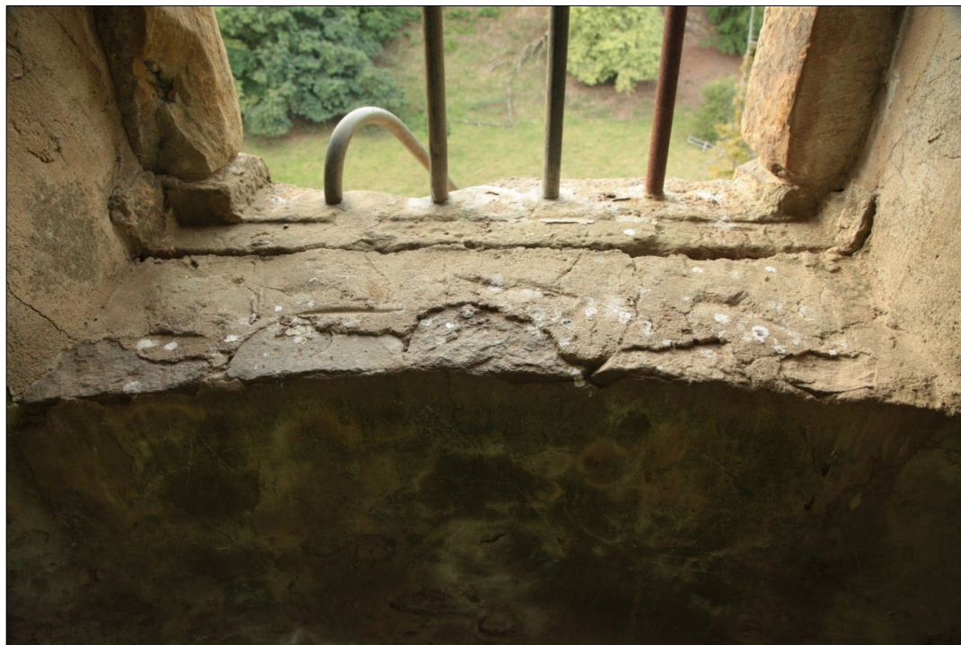
Plate 33: detail showing the inner stone windowsill and the moulding of the outer moulded sill.
