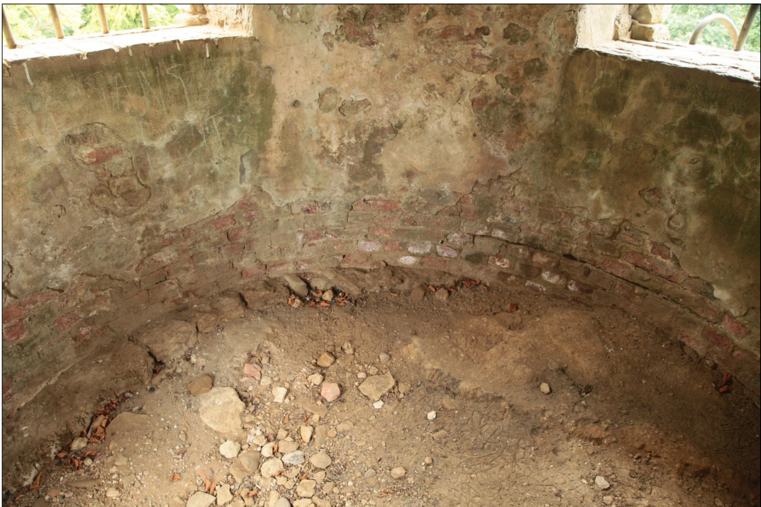
Plate 26: detail showing the curved stone foundation at the base of the exposed brick lining and the raised area to the right.
