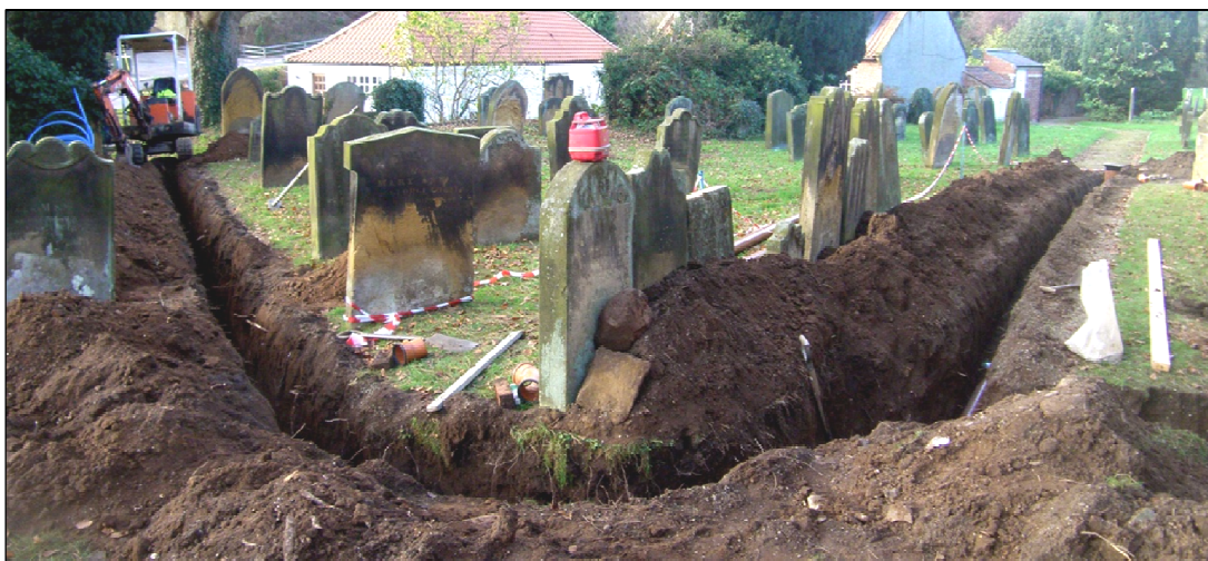
Plate 3 overall view of drain trench passing the west end of the church (to right) and turning down path to gate (left), facing north-west
