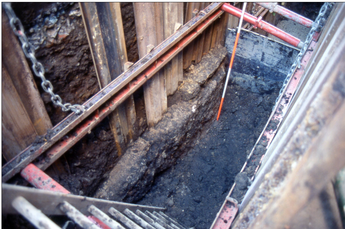
Plate 4 High Petergate, York: oblique view of north-east face of mortared foundation of Roman gatehouse
