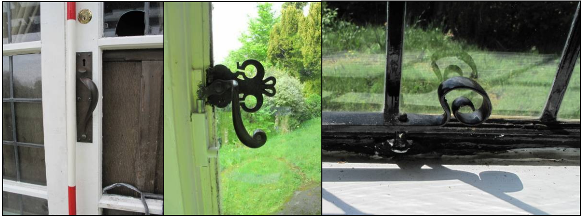
Plate 7: detail of door and window catches: veranda, Room 2 and Room 9 (left to right)
