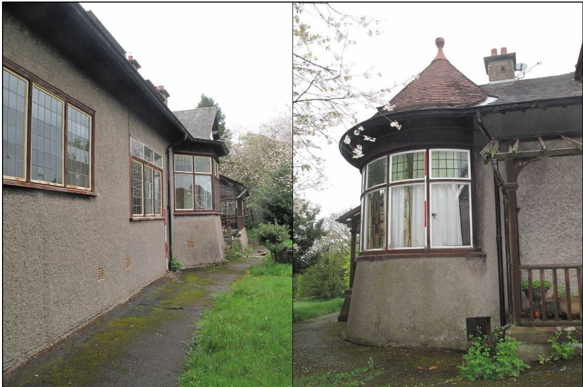
Plate 6: windows in south-west facing elevation, facing east, and the corner tower, facing north-west. Note the small window at the base of the tower.
